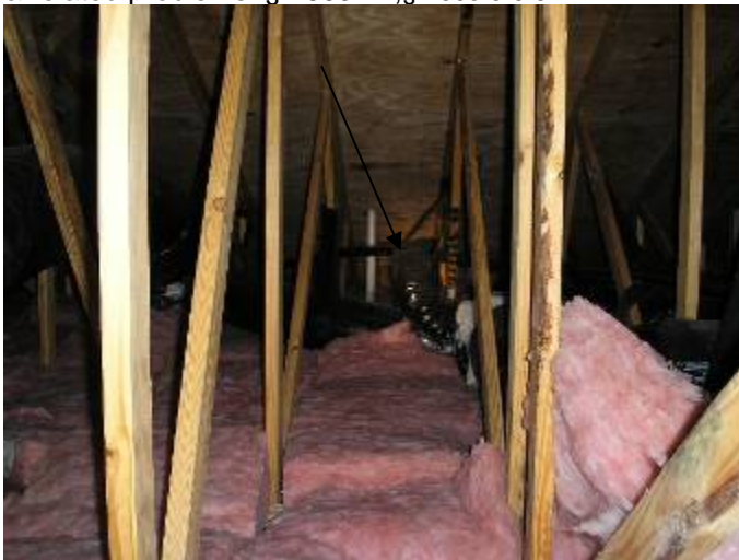
Some of the ductwork was not correctly supported off the attic insulation or other ductwork to prevent condensation & related problems. §M603.11, §M603.5.6.6
