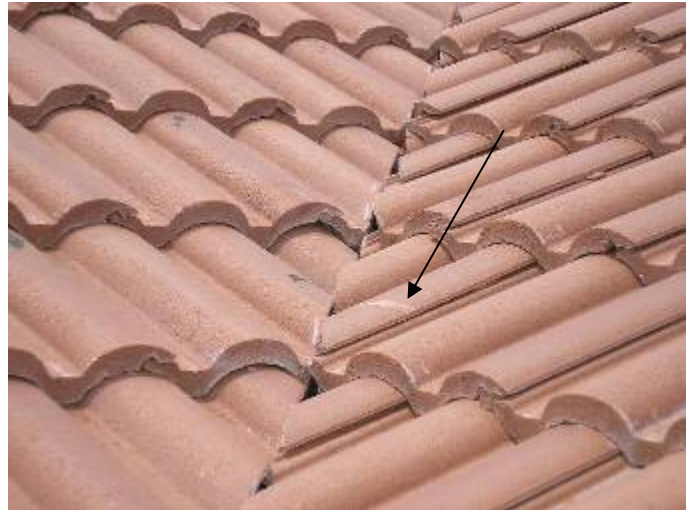
There were some broken tile pieces that were incorrectly "glued" back together with an RT-600 type adhesive product. These tiles should be removed & replaced.
