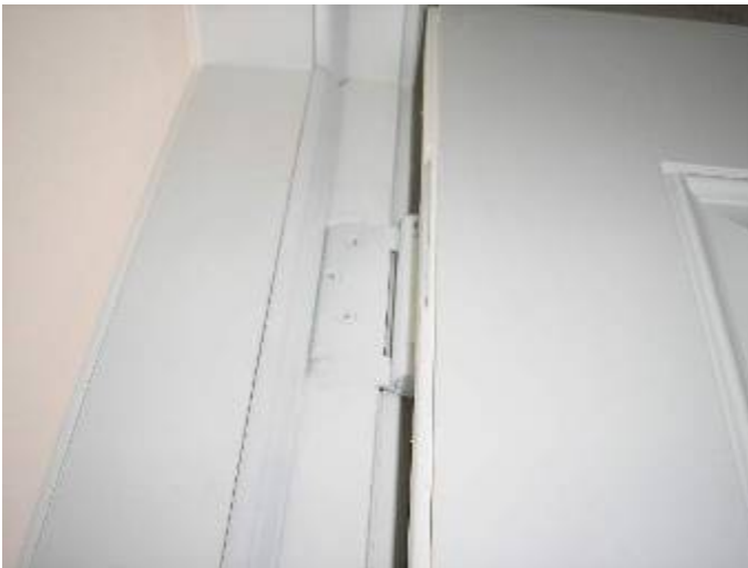
Touch-up paint was applied at the hinges at the garage/laundry door frame at the time of the inspection.
