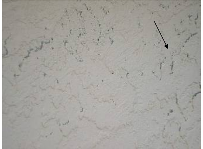
There were still some areas with exposed stucco & not enough paint on the exterior walls.
