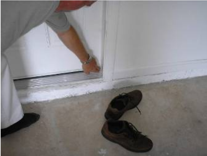
There was an unsealed gap between the door & frame at the garage/laundry area access. §13-606.1.ABC.1.2
