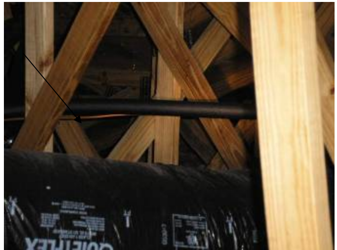
Some of the AC refrigerant line piping was not correctly supported in the attic. §M305.4
