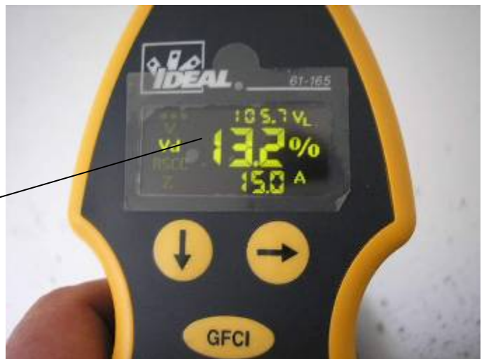
Some of the receptacle outlets had voltage drops that exceed 5% 2002(NEC) 210.19 Conductors. - See Below.
