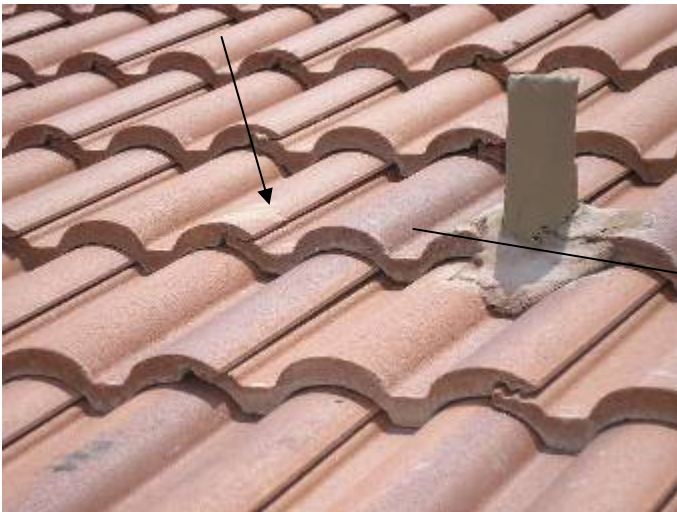
There were some broken tile pieces that were incorrectly "glued" back together with an RT-600 type adhesive product. These tiles should be removed & replaced.
