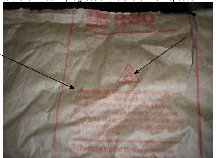
There is exposed kraft paper insulation backing in the attic. The manufacturer states the facing will burn & should not be exposed. §M304.1, §708.2
