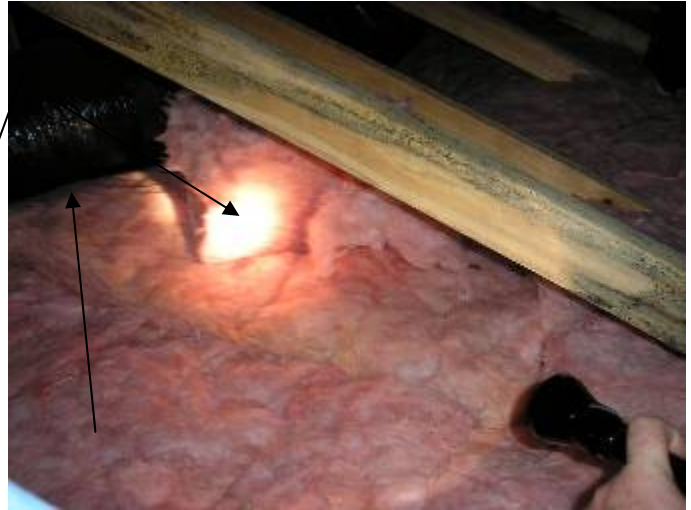
All debris & insulation scraps should be removed from the attic.
