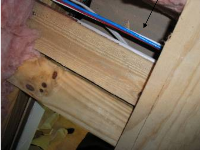
Insulation had not been installed at the back of the drywall by the attic access opening. §13-604.1.ABC.1
