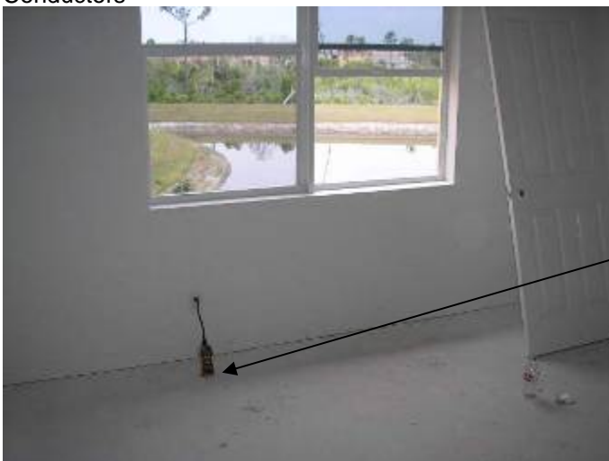
Location of the previous photo/s. Some of the voltage drops exceed 5%. 2002(NEC) 210.19 Conductors
