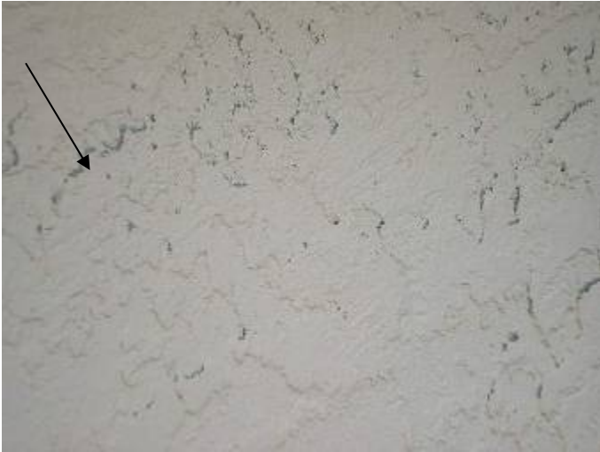
There were still some areas with exposed stucco & not enough paint on the exterior walls.
