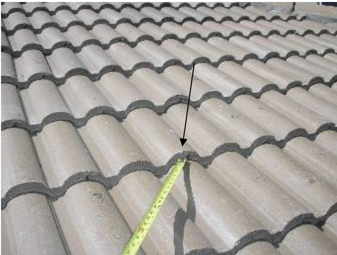
There were still some broken & incorrectly repaired roof tiles at several locations. The broken roof tiles should be removed & replaced, not "glued" back together.
