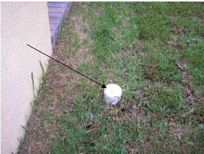
The plumbing waste line cleanout access is located in an area where pedestrian traffic is likely. The cleanout pipe is a trip hazard. §P708.2 A countersunk head should be used.
