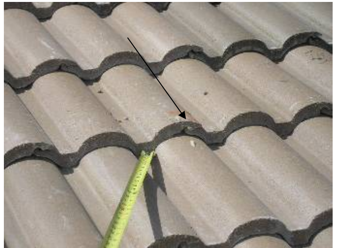
There were still some broken & incorrectly repaired roof tiles at several locations. The broken roof tiles should be removed & replaced, not "glued" back together.
