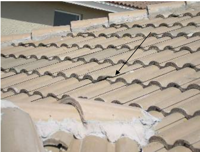
There were still some broken & incorrectly repaired roof tiles at several locations. The broken roof tiles should be removed & replaced, not "glued" back together.
