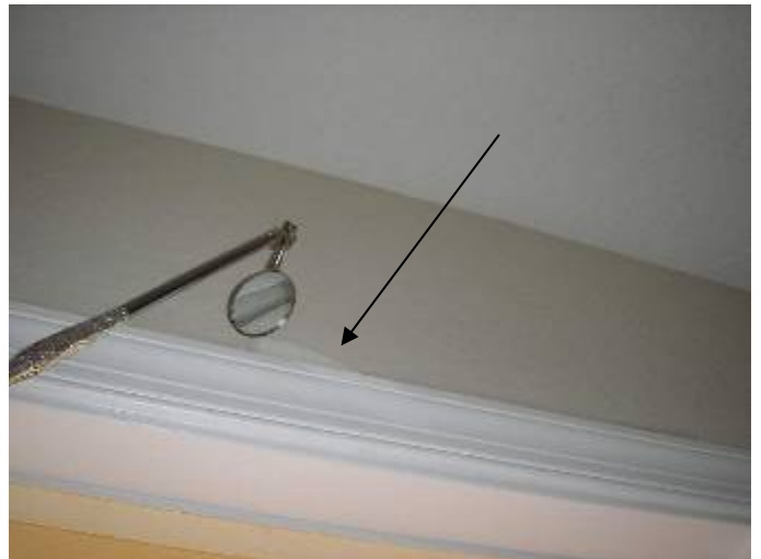
There was still no paint on the top of the front door trim.
