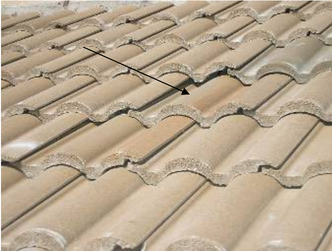
There were tiles that did not appear to be correctly set at multiple locations. We were not granted access to walk the roof to verify this condition.
