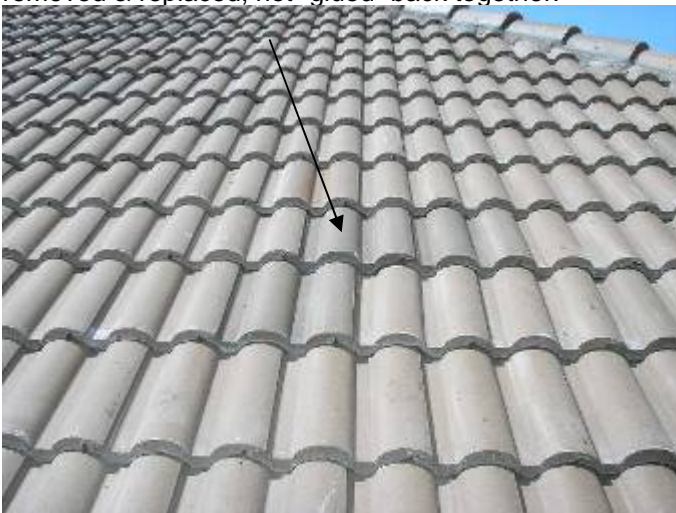
There are replacement tiles that do not match the original roof color.
