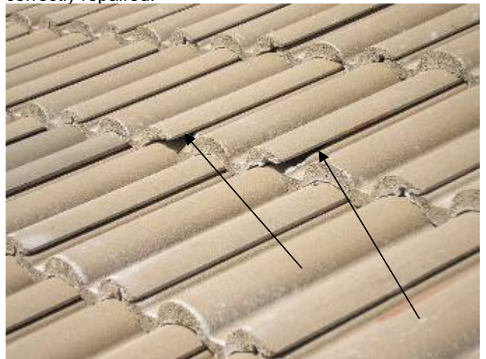
There were tiles that did not appear to be correctly set at multiple locations. We were not granted access to walk the roof to verify this condition.
