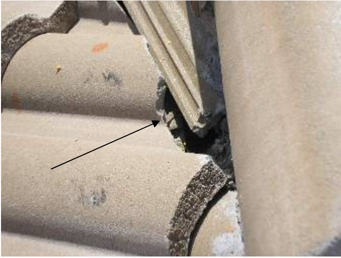
There was still some construction debris in the valleys. All debris should be removed from the roof.
