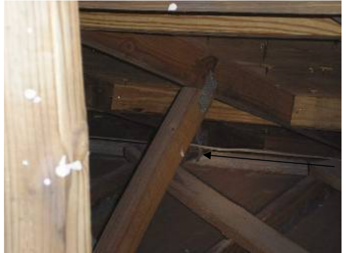
We were unable to verify all corrections in the attic as we were requested by the builder not to leave the ladder.
