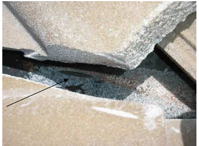
There appear to be cuts in the roof underlayment in the valleys. Any damaged roof underlayment should be correctly repaired.
