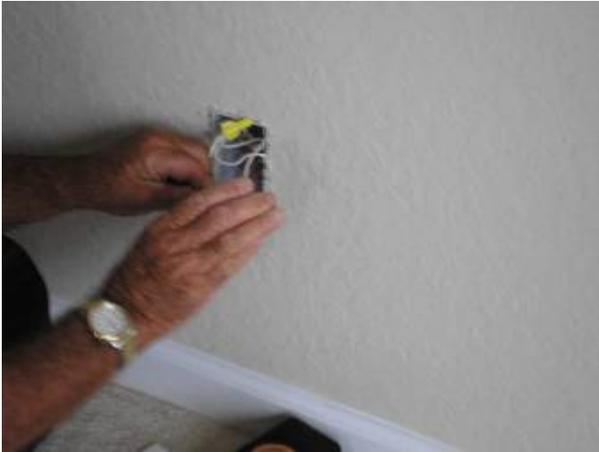
The west master bedroom receptacle tested loose or open ground. The grounding condition was repaired during the inspection.
