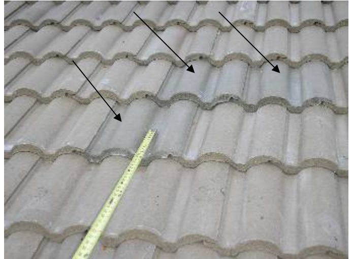
There are replacement tiles that do not match the original roof color. The tiles should be removed & replaced with matching color tiles.
