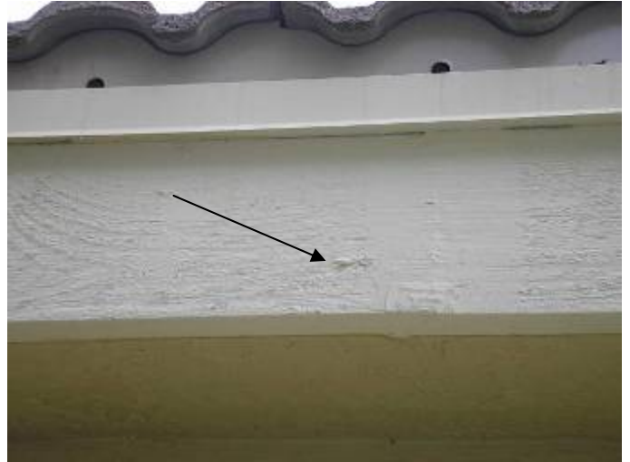
There were several nails protruding through the fascia. Dr Warren requested we mention this concern.
