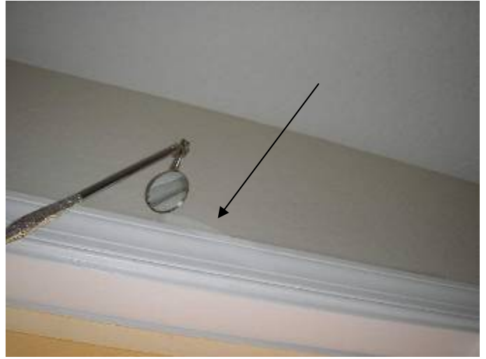
There is no paint on the top of the front door trim.
