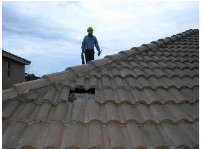
Note: Roof repair work was in progress during the time of the inspection.
