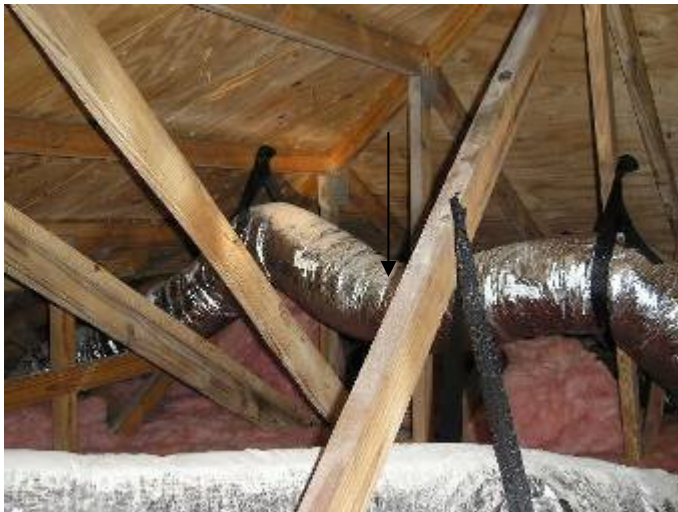
Some of the AC ductwork was sagging & not correctly supported. §13-610.1.ABC.3.3.6
