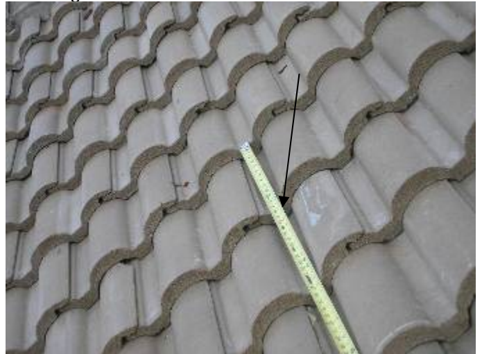
The roof tiles are 16 & 1/2" in length. There should be no more than 13 & 1/2 inches of exposed roof tile to allow for the correct headlap. §1518.8.11 See Below & builder response
