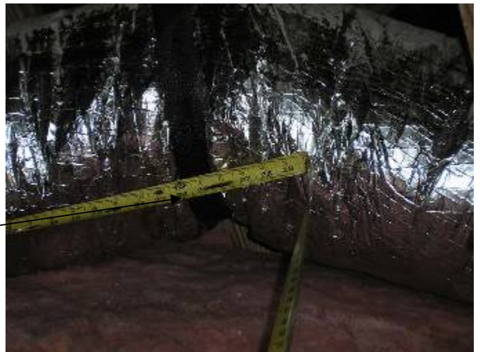
The ductwork needs to be supported within 18 inches of the distribution box. §13-610.1.ABC.3.3.6
