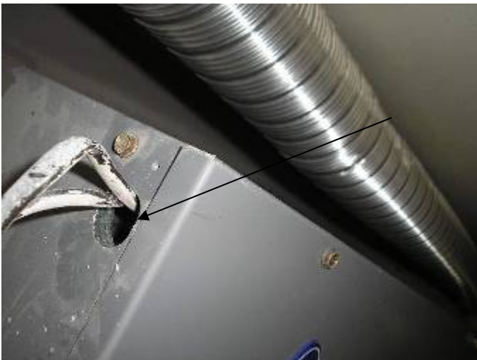
The AC air handler is not completely sealed; the grommet has not been installed around the wiring through the top of the unit. §13-410.1.ABCD.3.5
