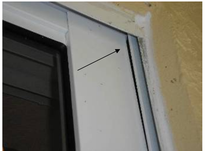
There were gaps between the sliding glass doors & frame. §13-606.1.ABC.1.2
