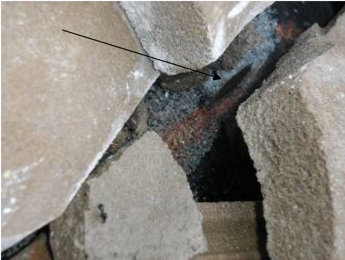
There appear to be cuts in the roof underlayment in the valleys. Any damaged roof underlayment should be correctly repaired.
