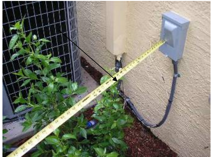
The landscape vegetation obstructs the required working space clearance at the AC disconnect electrical access cover. 36" clearance is required. 2002 NEC 110.26
