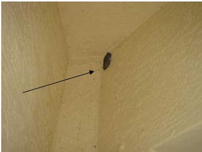
Wasps' nests should be removed from the exterior of the building. -Hazard.
