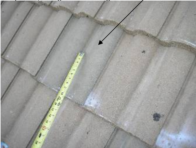
There are replacement tiles that do not match the original roof color. The tiles should be removed & replaced with matching color tiles.
