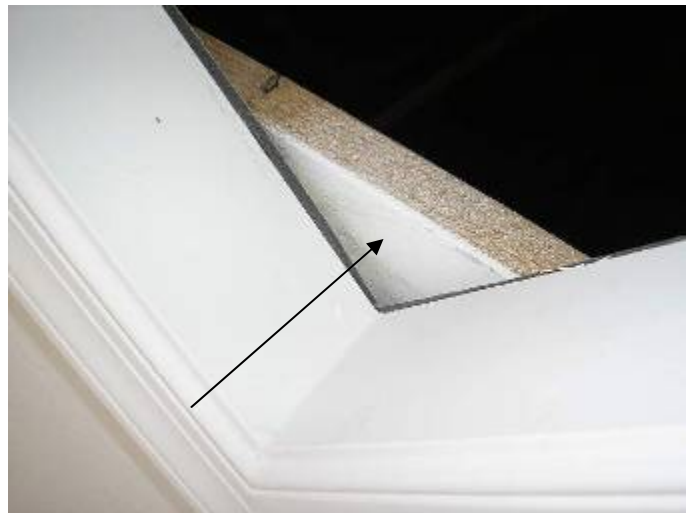
The 2x4 ceiling support bracing does not allow the attic access lid to be opened easily. $2309.6
