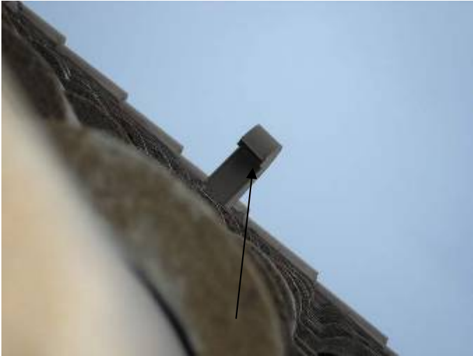
Some of the exhaust vent hoods do not appear to have the correct screening or dampers to prevent pest intrusion.
