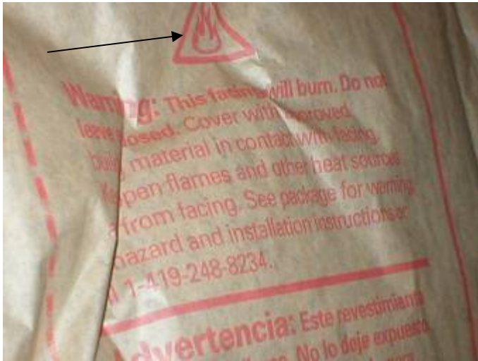
The manufacturer states the paper facing is flammable & should not be exposed. §M304.1, §708.2
