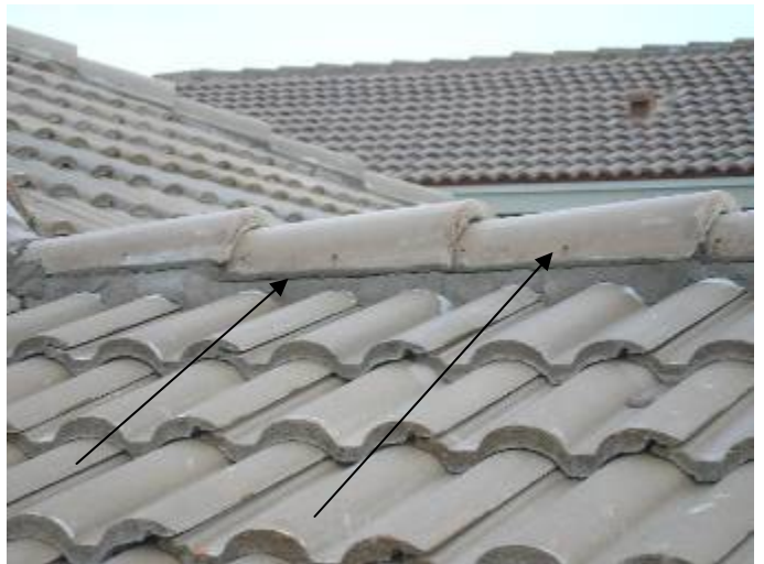
Some of the hip & ridge cap tiles do not appear to be correctly secured or bonded. We were not granted access to walk the roof to verify this condition.
