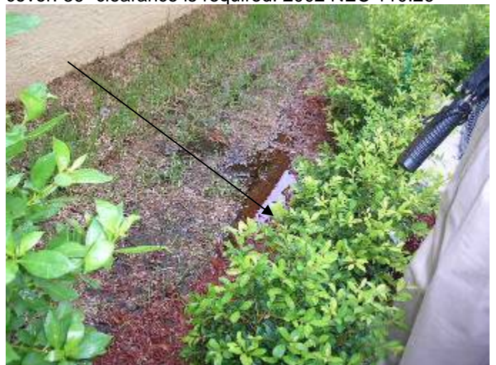
The yard at the sides of the building are very wet & did not appear to be draining correctly. The rear yard appears to be pitched towards the building.
