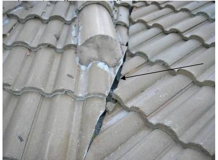
Location of the previous photo/s. All debris should be removed from the roof. There is exposed underlayment at some of the valleys R118-3.09
