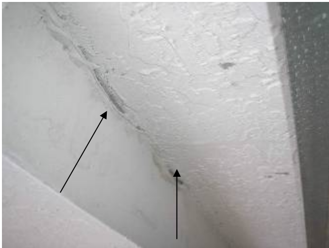
There were unsealed openings in the drywall under the electrical panel in the garage.
