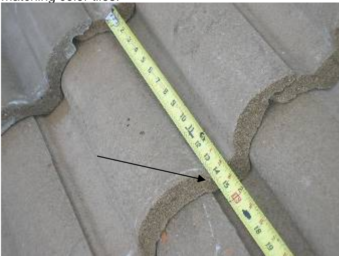
The tile exposure is 14 inches or more at multiple locations. This indicated there is less than 3" overlap.
