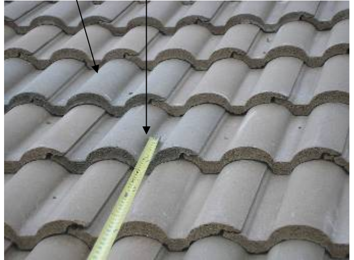
There are replacement tiles that do not match the original roof color. The tiles should be removed & replaced with matching color tiles.
