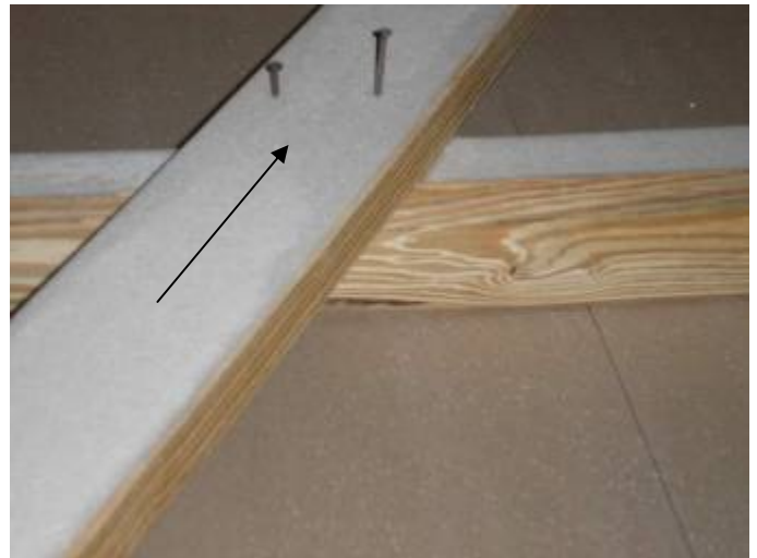
The ceiling joist (rat run) was not completely secured in the attic. §2306.2
