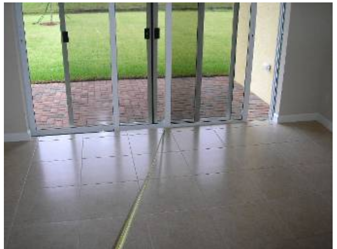
The sliding glass door was sticking in the frame.
