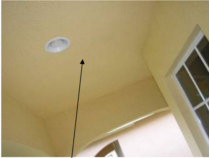
The stucco at the entryway ceiling is concave or curved up & does not appear to be the correct thickness. Review the builder's stucco report to determine if this area was tested.
