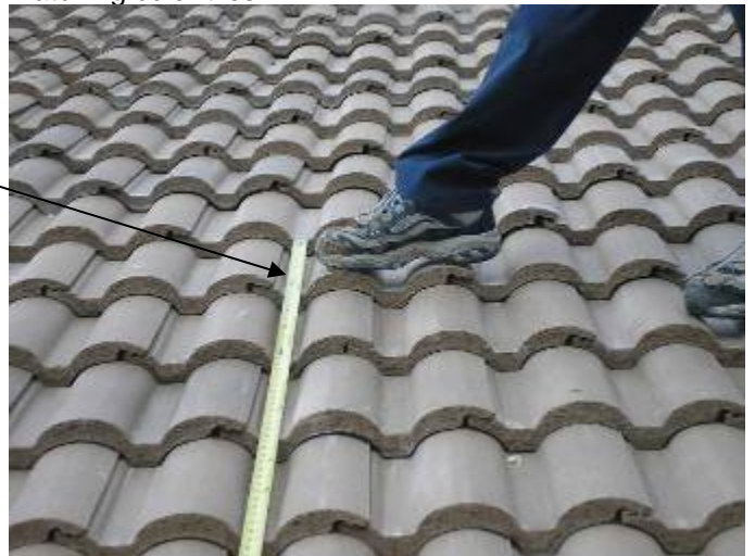
The roof tiles are 16 & 1/2" in length. There should be no more than 13 & 1/2 inches of exposed roof tile to allow for the correct headlap. §1518.8.11
