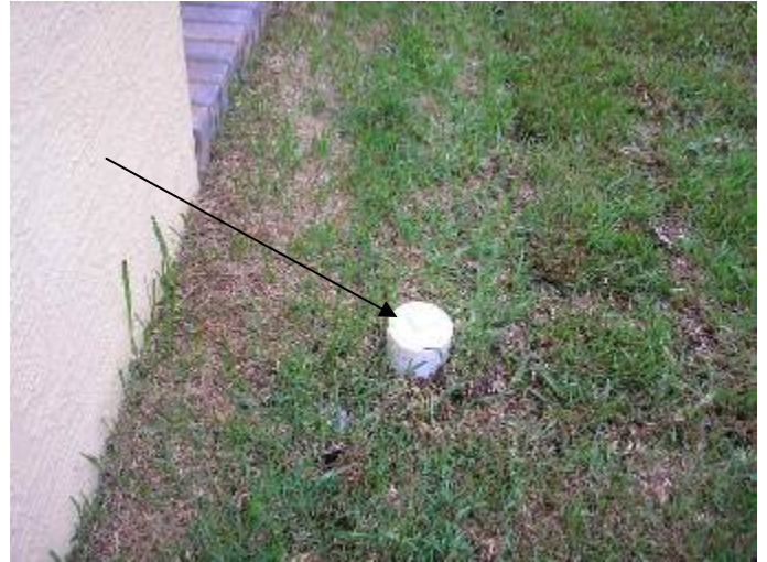
The plumbing waste line cleanout access is located in an area where pedestrian traffic is likely. The cleanout pipe is a trip hazard. §P708.2
