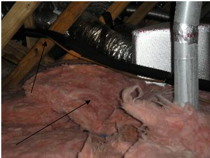
Some of the AC refrigerant line piping was not correctly supported at 6 ft intervals as required in the attic. §M305.4 Some of the insulation was out of place in the attic.
