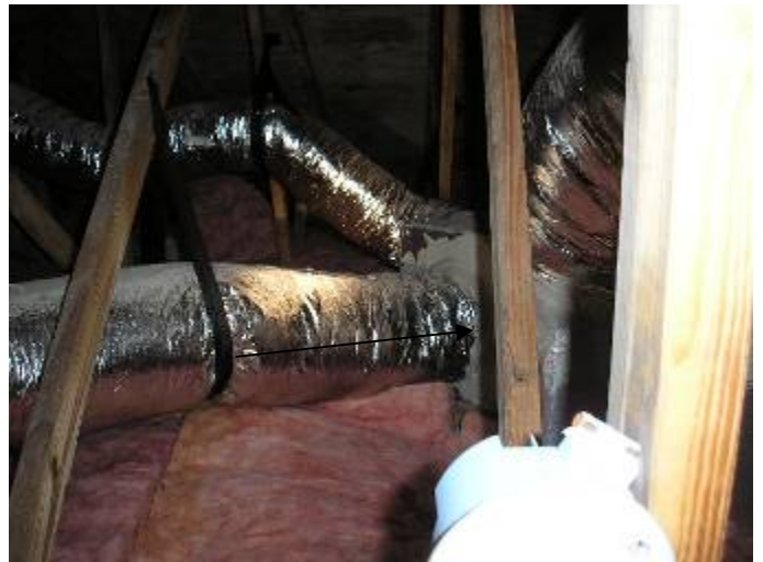
The ductwork needs to be supported within 18 inches of the distribution boxes. §13-610.1.ABC.3.3.6
