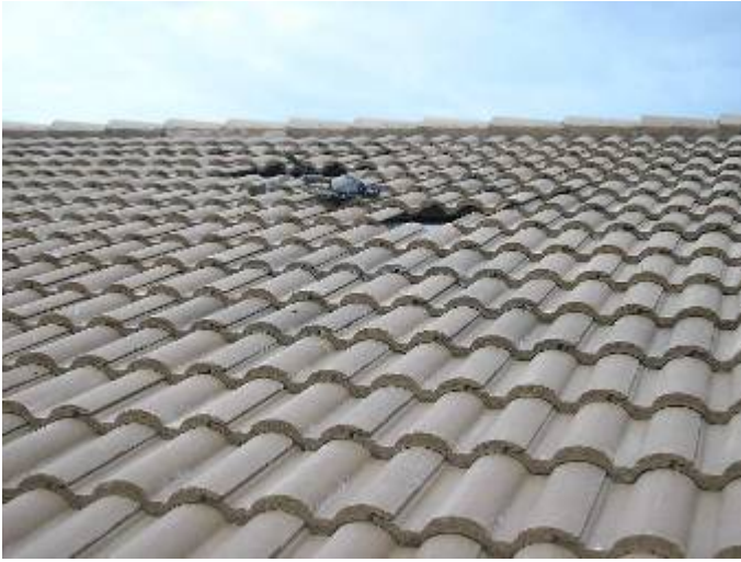
Note: Roof repair work was in progress during the time of the inspection.
