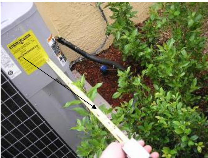
The landscape vegetation obstructs the required working space clearance at the condensing unit electrical access cover. 36" clearance is required. 2002 NEC 110.26
