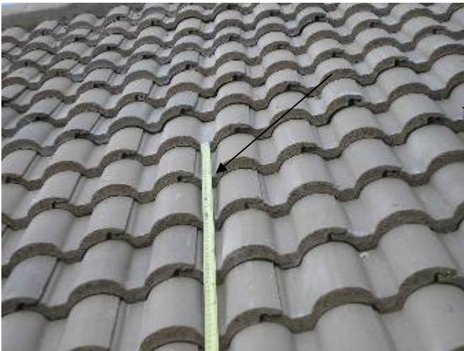
The tile exposure is 14 inches or more at some locations. The tile headlap or overlap is required to be 3 inches. §1518.8.11
