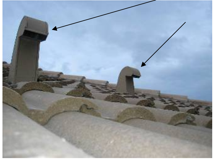
Some of the exhaust vent hoods do not appear to have the correct screening or dampers to prevent pest intrusion.
