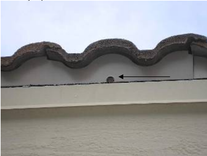
Some of the bird stop weep hole openings are blocked & obstructed with construction debris. All of the weep holes should be open & free of debris. §1518.8.9 Florida Building Code
