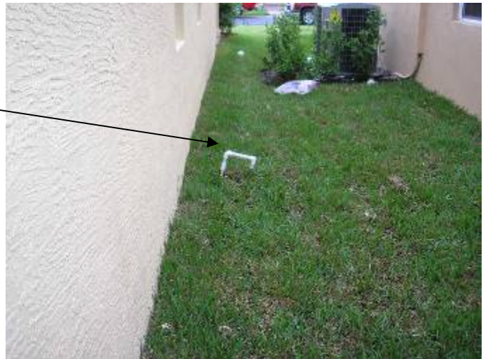
The builder's representative agreed to straighten out the AC condensate drain piping.
