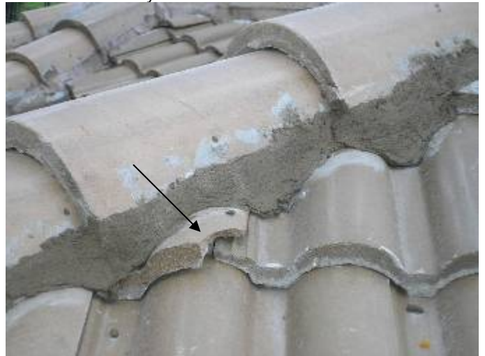
The broken tiles should be removed & replaced with new tiles.
