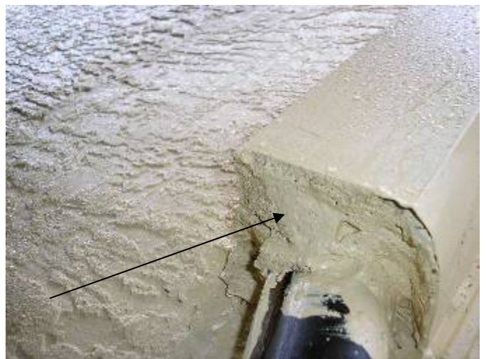
Cement, mortar or non-corrodible metal should be used to close the opening around the refrigerant line piping. §1205.1.2.2
