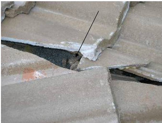
There is broken tile & debris in some of the valleys.
