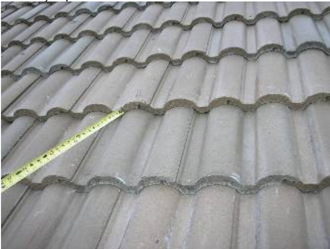
There were cracked & broken tiles on the roof at several locations.
