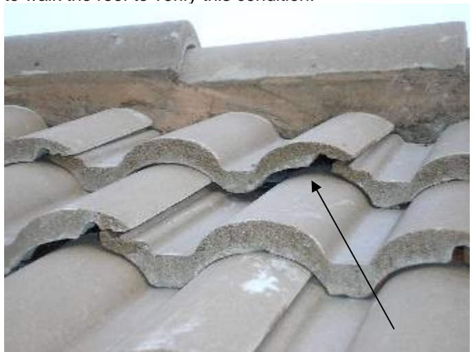
There were tiles that did not appear to be correctly set at multiple locations. We were not granted access to walk the roof to verify this condition.
