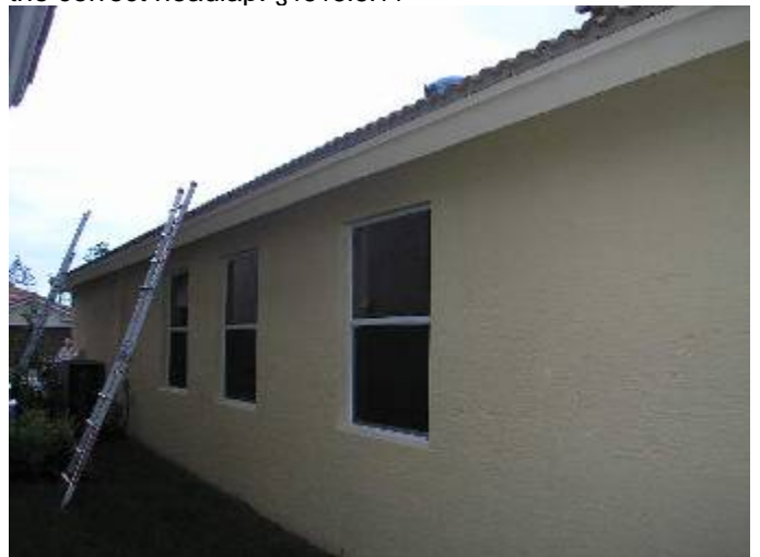
Location of the previous photo/s. See the documentation from the builder that states the tile headlap does not need to be a minimum of 3 inches in all cases.
