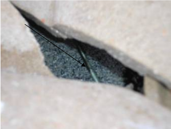
There appear to be cuts in the roof underlayment in the valleys. Any damaged roof underlayment should be correctly repaired.
