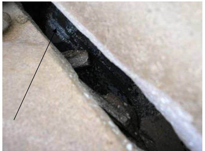
There appear to be cuts in the roof underlayment in the valleys. Any damaged roof underlayment should be correctly repaired.
