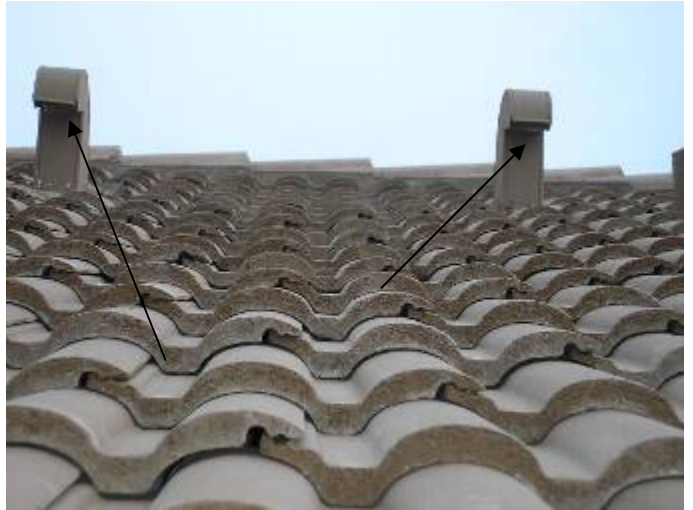
Some of the exhaust vent hoods do not appear to have the correct screening or dampers to prevent pest intrusion.
