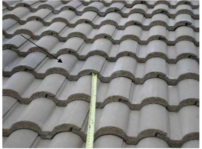
There are replacement tiles that do not match the original roof color. The tiles should be removed & replaced with matching color tiles.
