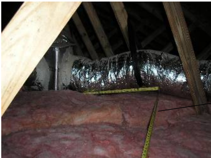
The ductwork needs to be supported within 18 inches of the distribution box. §13-610.1.ABC.3.3.6
