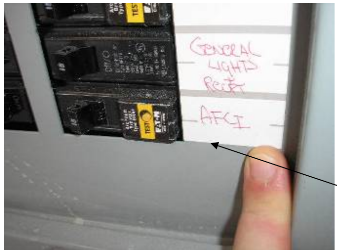
The circuits are not all completely identified to indicate the location of service.
