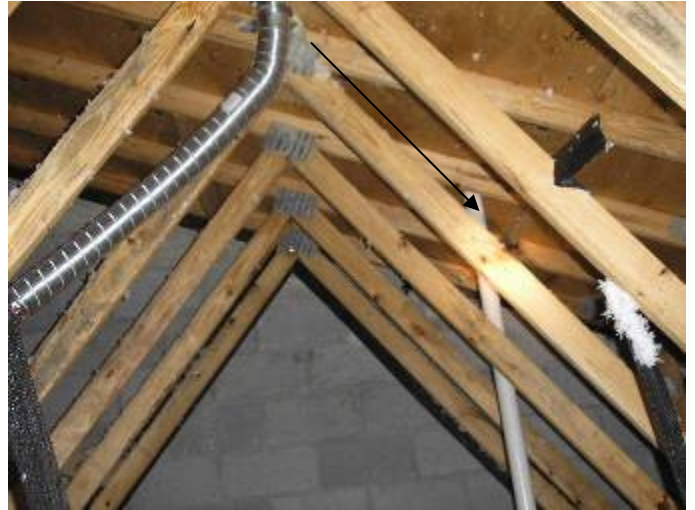
The plumbing drain waste vent stack terminates too close to bath exhaust vent opening. Sewer gasses can re-enter attic & house- Potential Hazard. §P904.5 Florida Building Code
