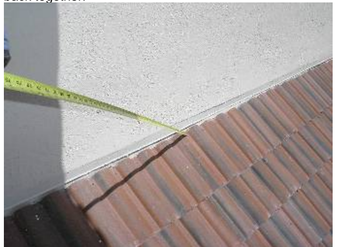
The roof wall abutments have not been correctly pointed up with mortar at the back patio. R118-3.13
