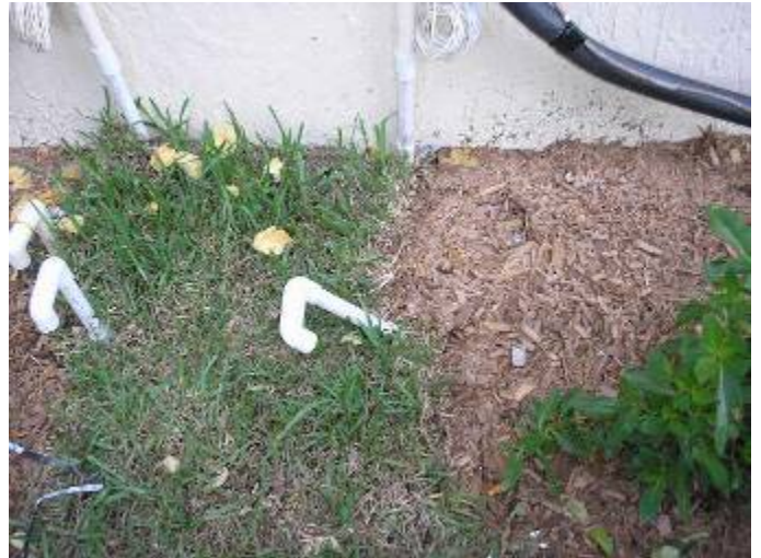
The condensate drain line is leaning over & not plumb or correctly supported.
