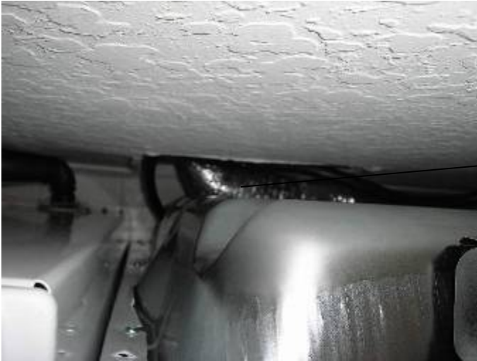
The foil vent duct is a fire hazard per the manufacturer.
