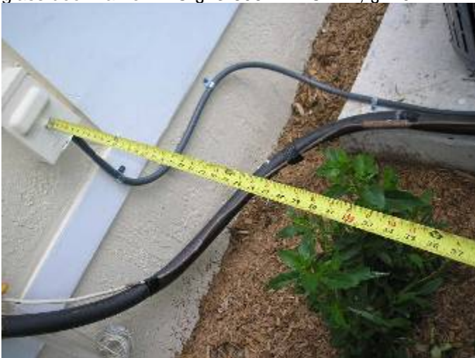
The landscape vegetation obstructs the required working space clearance at the AC disconnect electrical access cover. 36" clearance is required. 2002 NEC 110.26 2002 NEC
