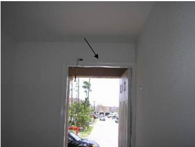
The top of the trim is not correctly sealed to prevent AC loss at the front & garage access door frames. FBC §13-606.1.ABC.1.2
