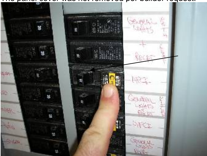
The AFCI arc fault breaker did not move to the fully tripped position when tested.
