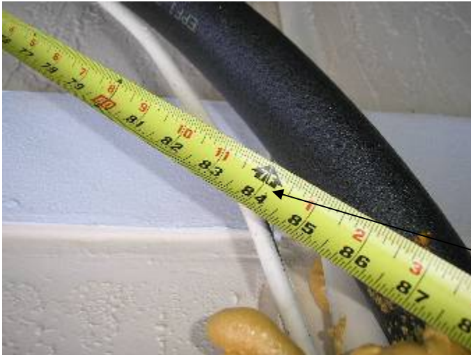
The exterior AC refrigerant line piping was not correctly supported at 6 ft intervals as required. §M305.4
