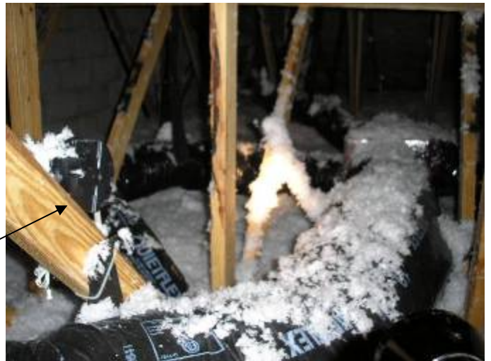
Some of the AC ductwork is not correctly installed or supported in the attic. §13-610.1.ABC.3.3.6
