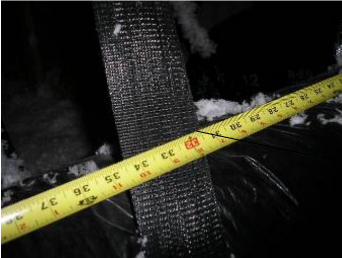
Some of the AC ductwork is not correctly installed or supported in the attic. The ducts are sagging & also need to be supported within 18" of connections or fittings.
