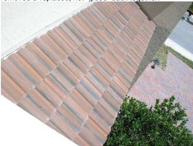
Location of the previous photo/s from the master balcony. The builder does not permit inspectors to walk on the roof.
