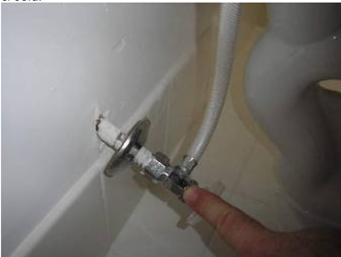
Some of the plumbing supply lines are not correctly secured behind the wall at the W.C. (toilets) & for the sink faucets. This line was bent & not level.
