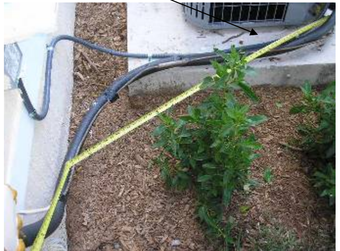
3 Anchors are required on each side of the condensing unit. M301.13.1 The AC refrigerant line piping was not correctly supported at 6 ft intervals as required. §M305.4
