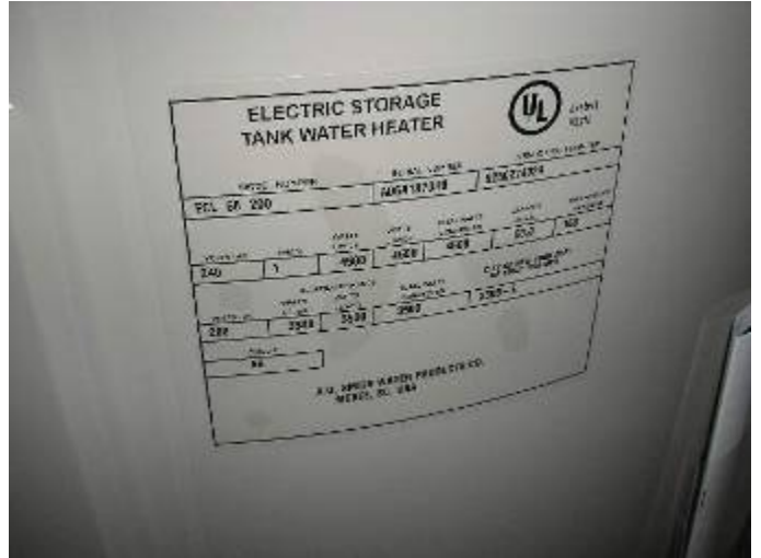
Note: 50 gallon electric water heater.
