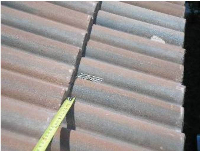
All debris should be removed from the roof.
