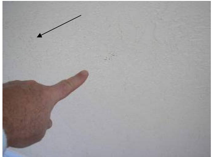
Some of the stucco is visible indicating there is not enough paint on the exterior walls.
