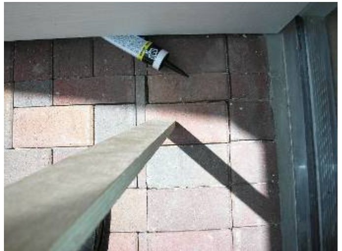
Some of the pavers were loose, damaged or out of place at the driveway & walkway.
