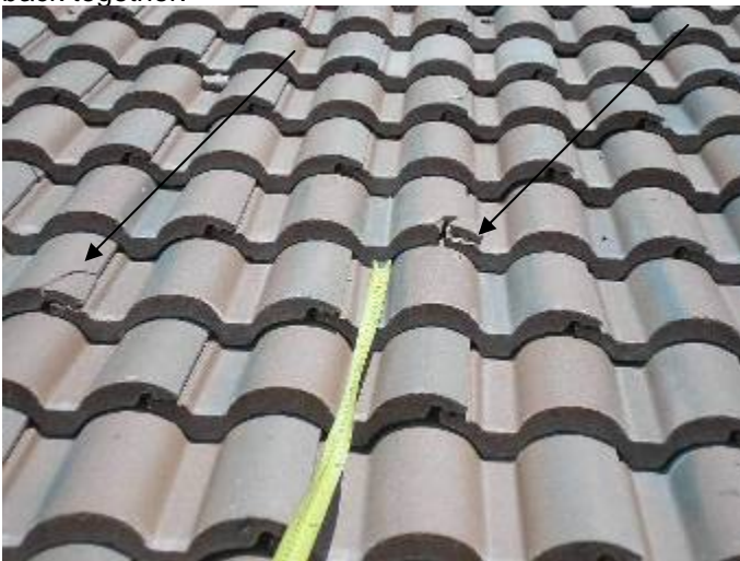
There were broken & incorrectly repaired roof tiles at several locations. The broken roof tiles should be removed & replaced, not "glued" back together.
