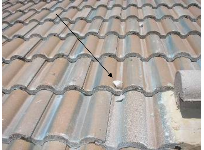
There is broken tile & debris at several locations.
