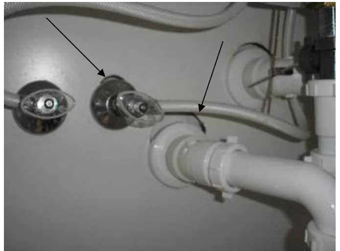
Some of the plumbing supply lines are not correctly secured or sealed at/behind the wall at the W.C. (toilets) & for the sink faucets.
