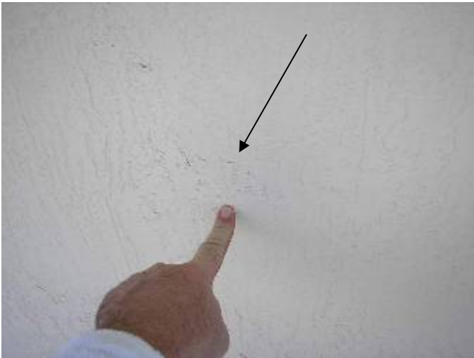
Some of the stucco is visible indicating there is not enough paint on the exterior walls.
