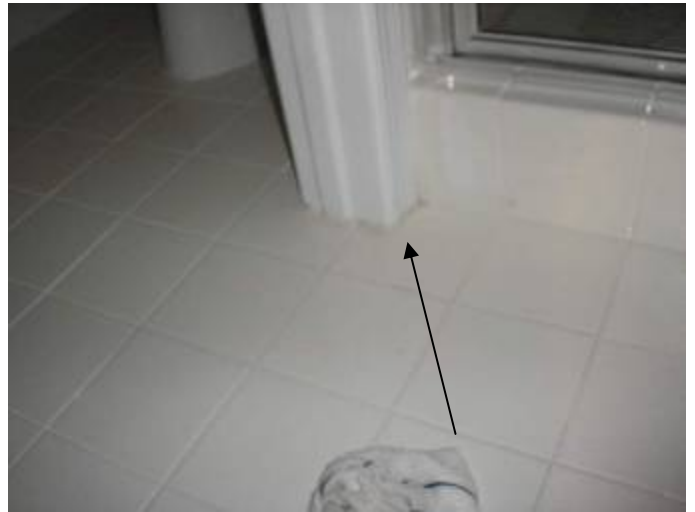
Water leaked from the shower through the wall to the master bathroom floor after about ½ hr. §P417.5.2
