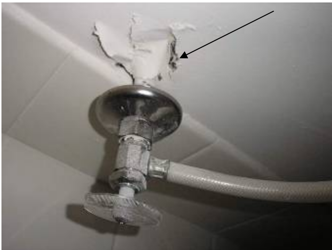
Some of the plumbing supply lines are not correctly secured or sealed at/behind the wall at the W.C. (toilets) & for the sink faucets.
