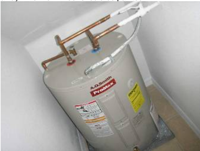
Note: the power was not on until the end of the inspection. Plumbing faucets need to be reviewed for hot & cold.
