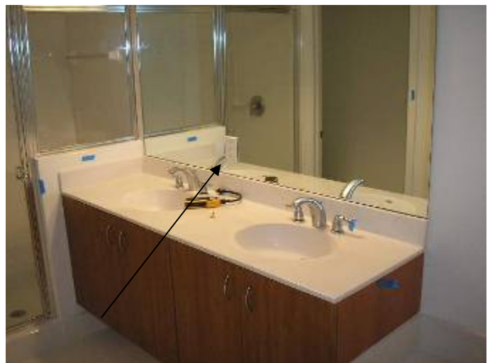
Note: There is only 1 receptacle outlet at the master bathroom lavatory sink area. Review the electrical plan to confirm there should not be 2 separate outlets.
