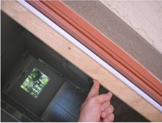
A straight edge was verified at the front door frame & used to check the exterior walls.
