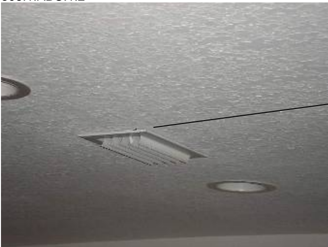
Some of the AC vent registers are not completely sealed or secured at the drywall.
