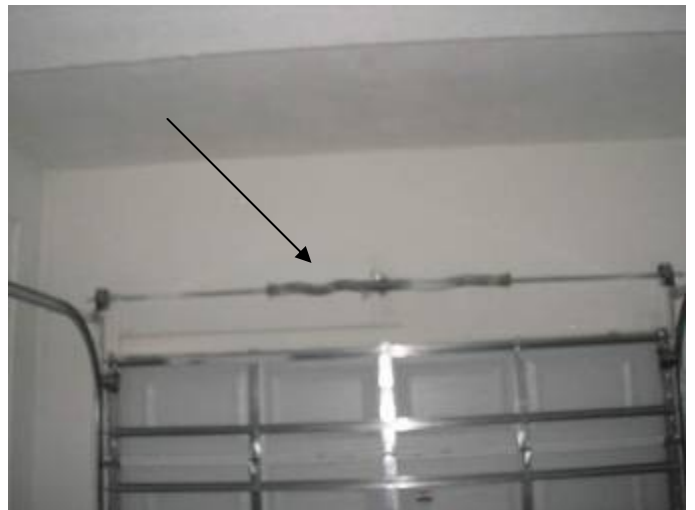
The garage vehicle auto door opener counter balance spring did not operate correctly. The door slams down when it is let go.
