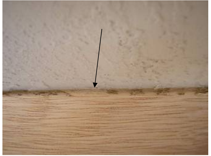
Some of the stucco work appears to be uneven, concave & not the proper depth. ASTM C 926, §2504.2 §1403.1.3
