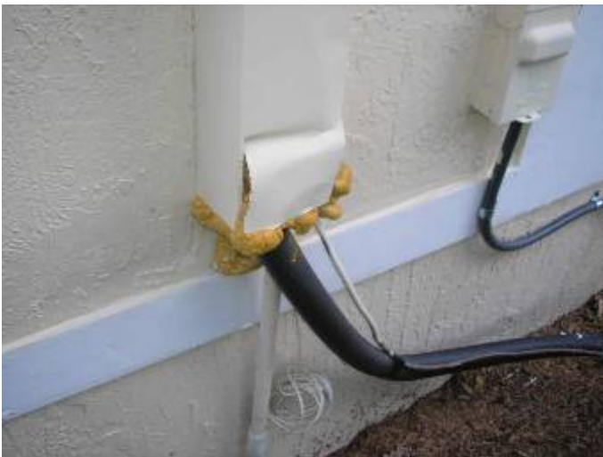
The AC line cover is damaged with sharp edges. Cement, mortar or non-corrodible metal should be used to close the opening around the refrigerant line piping.
