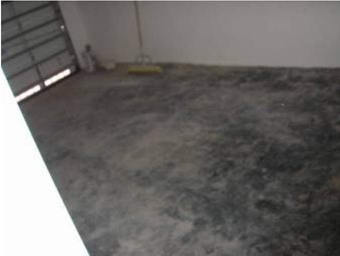
There is staining or discoloration on the garage floor. It does not appear that the discoloring can be washed away. The "new" floor should be painted.
