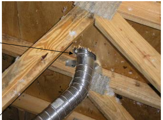
The area around the exhaust vent ducting is not sealed to prevent water & pest intrusion into the attic & house.
