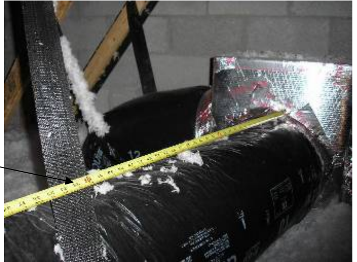
Some of the AC ductwork is not correctly installed or supported in the attic. §13-610.1.ABC.3.3.6
