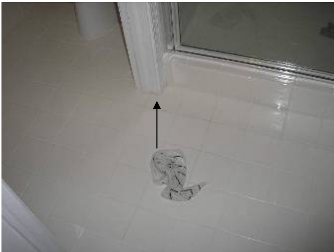
The tiles will need to be removed & the pan relined for a correct repair. §P417.5.2
