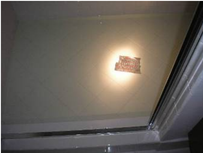
The 2 nd floor drains were taped & 1 & ½ inches of water was left to stand. §P417.5.2
