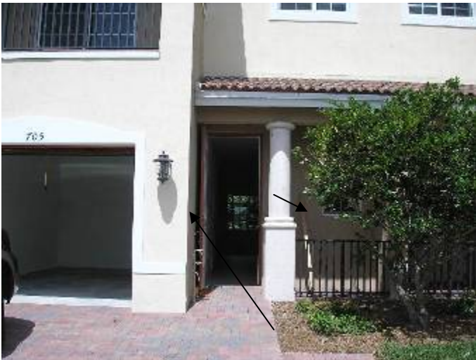
We recommend core sampling at these locations to verify the thickness of the exterior stucco & compliance with ASTM C 926.
