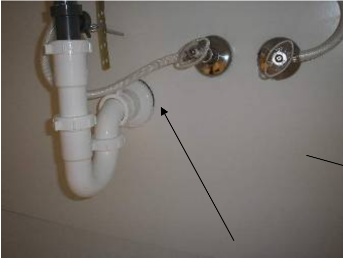
Some of the plumbing supply lines are not correctly secured or sealed at/behind the wall at the W.C. (toilets) & for the sink faucets.
