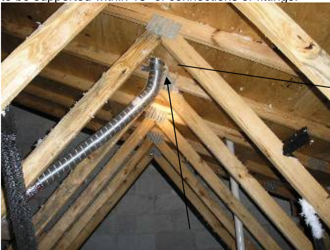
The openings in the roof sheathing/at the exhaust vents can become air intakes when the AC is operating. There is no designed make-up air provided with this AC system.
