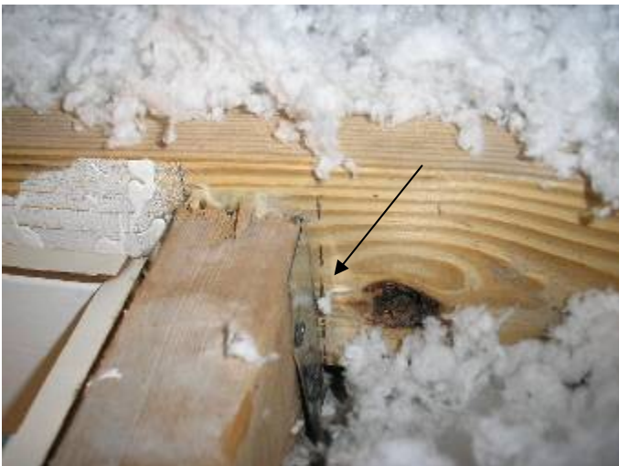
The drywall screws & light gauge metal are not designed to support the weight of persons entering the guest house attic. §2504.5
