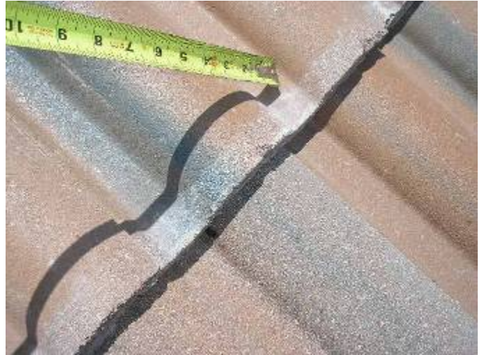
There is paint overspray on many of the roof tiles.
