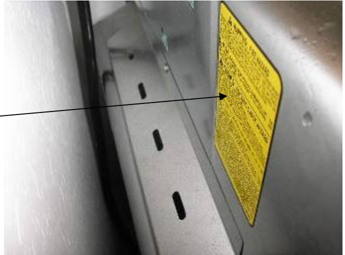
The thin aluminum foil dryer vent duct material is a fire hazard per CSPC & the manufacturer. See the warning label on the back of the dryer. §M304.1
