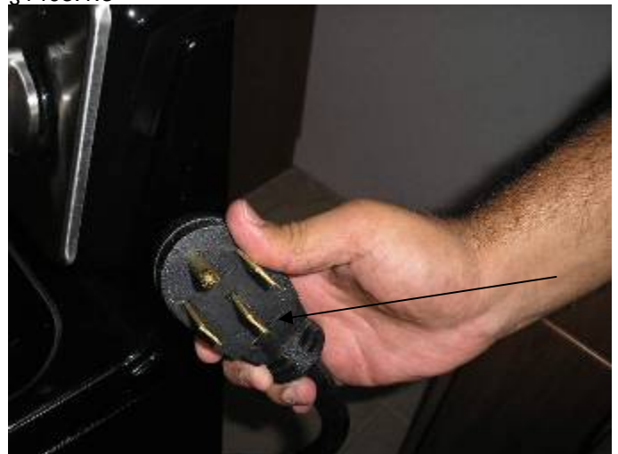
The range is installed with an electrical cord rated at 40 amps. The 50 amp overcurrent protection breaker in the main distribution panel is too big. §M304.1
