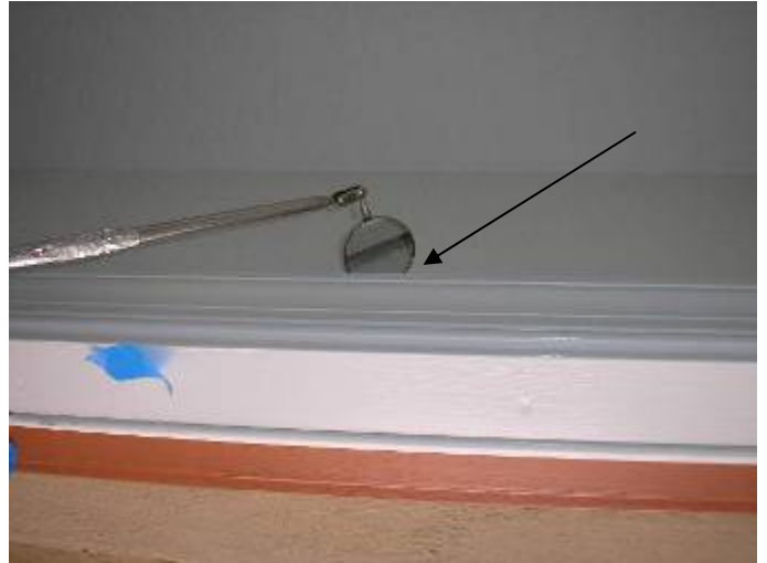
The top of the trim is not correctly sealed to prevent AC loss at the front & garage access door frames. FBC §13-606.1.ABC.1.2
