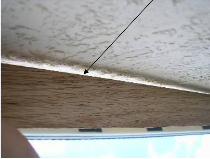
Some of the stucco work appears to be uneven, curved in/concave & not the proper depth. ASTM C 926, §2504.2 §1403.1.3
