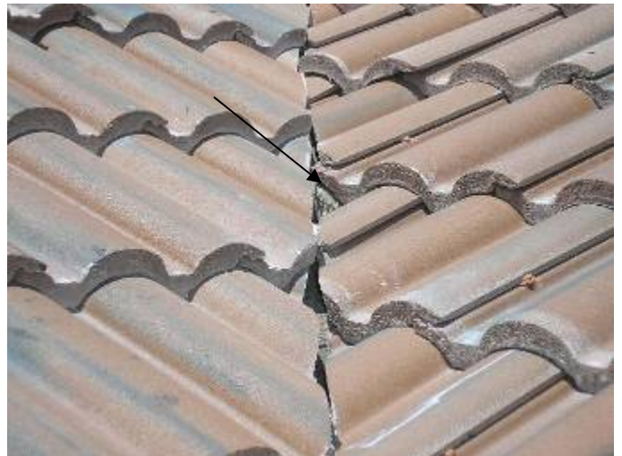
There is broken tile & debris in some valley locations.
