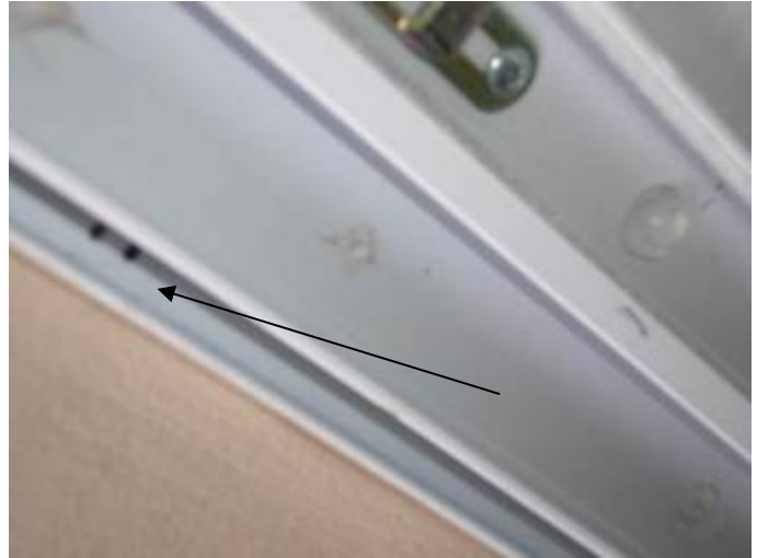
Some of the openings in the frame are not completely sealed to prevent water & pest intrusion at the sliding glass doors. FBC §13-606.1.ABC.1.2.
