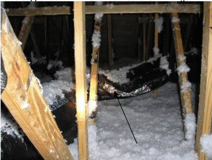
Some of the AC ductwork is not correctly installed or supported in the attic. The ducts are sagging & also need to be supported within 18" of connections or fittings.
