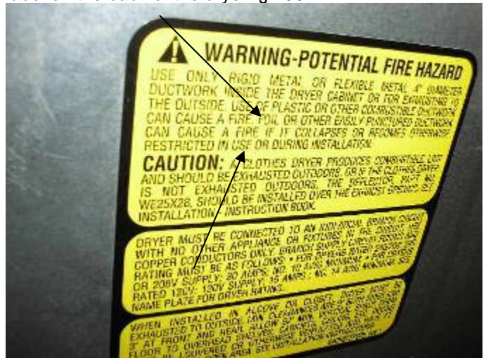
The thin aluminum foil dryer vent duct material is a fire hazard per CSPC & the manufacturer. See the warning label like this one on the back of the dryer. §M304.1
