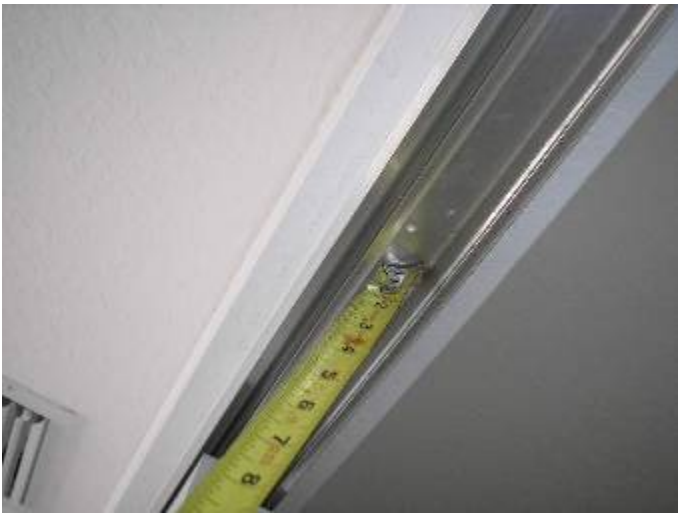
Some of the screw anchors are not installed at the bedroom closet door top tracks.
