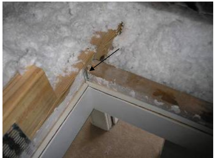
The drywall screws & light gauge metal are not designed to support the weight of persons entering the guest house attic. §2504.5
