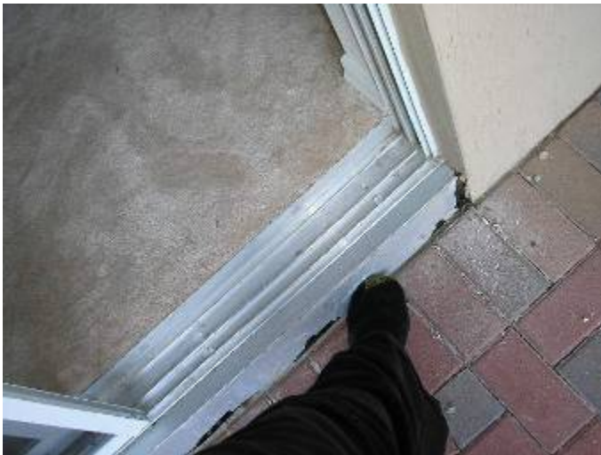
The flashing is not sealed at the bottom at the master balcony sliding glass doors.
