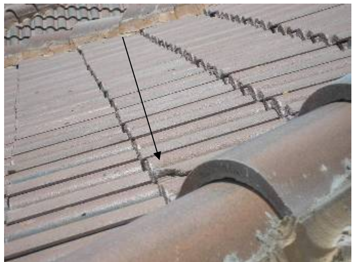
There were broken & incorrectly repaired roof tiles at multiple locations. The broken roof tiles should be removed & replaced, not "glued" back together.
