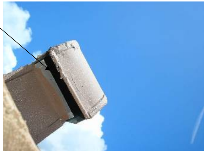
Some of the exhaust vent hoods do not appear to have the correct screening or dampers to prevent pest intrusion.
