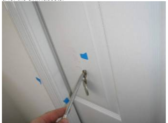
Damage to the pocket door should be corrected.
