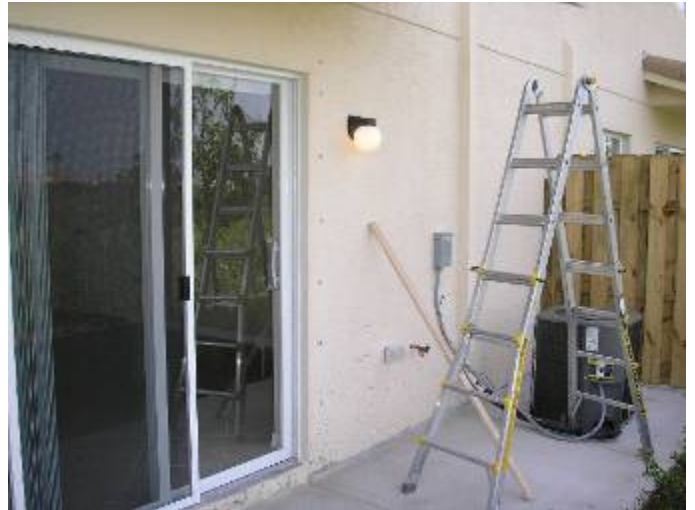
We recommend core sampling to verify the thickness of the exterior stucco & compliance with ASTM C 926.
