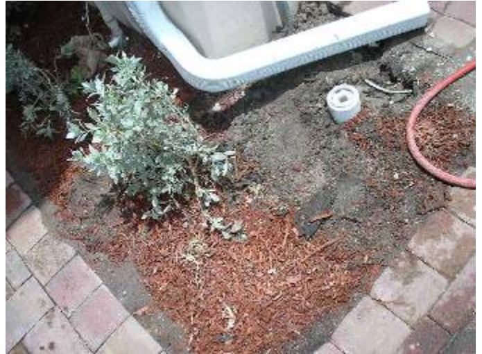
The mulch installation was incomplete.
