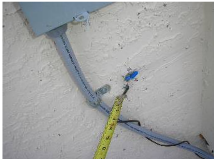
The low voltage wiring & connection are not correctly protected from damage.
