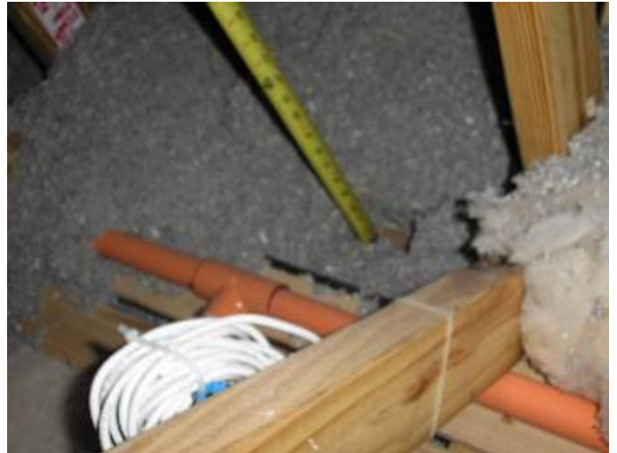
There were some locations where the attic insulation was not the correct depth.
