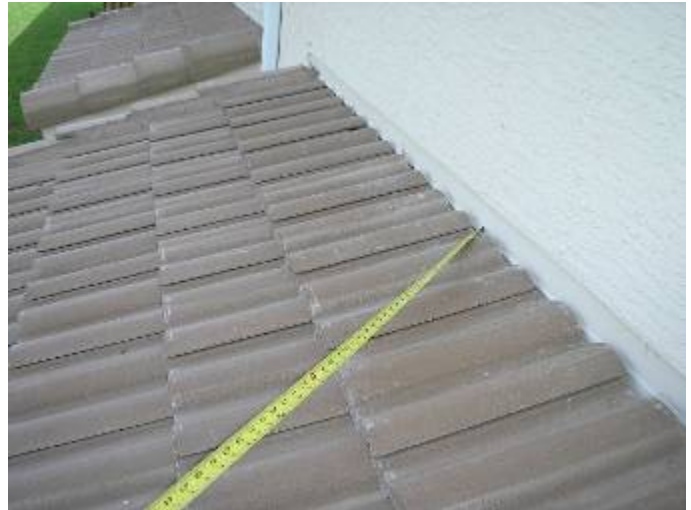
The roof wall abutments have not been correctly pointed up with mortar at the back patio. §1518.8, R118-3.13
