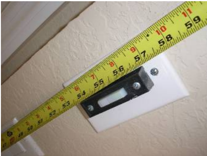
The garage door auto opener control switch is too low on the wall.
