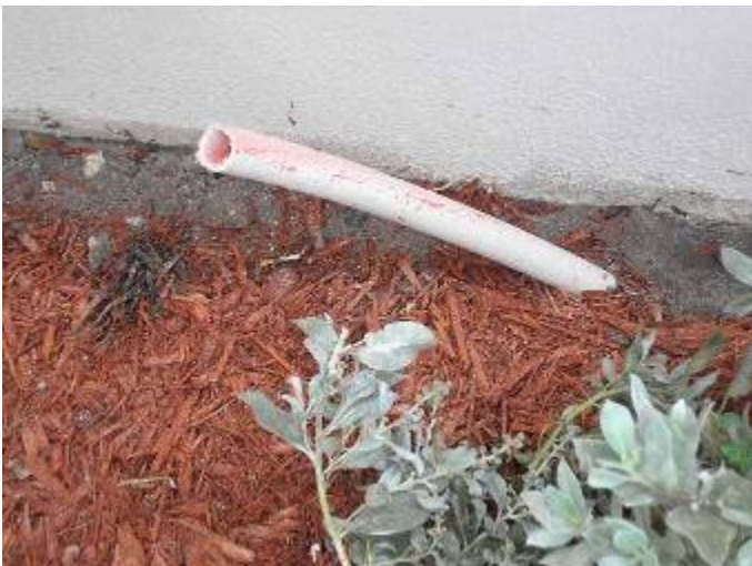
There was an open ended conduit at the front entry way. What is this pipe for?
