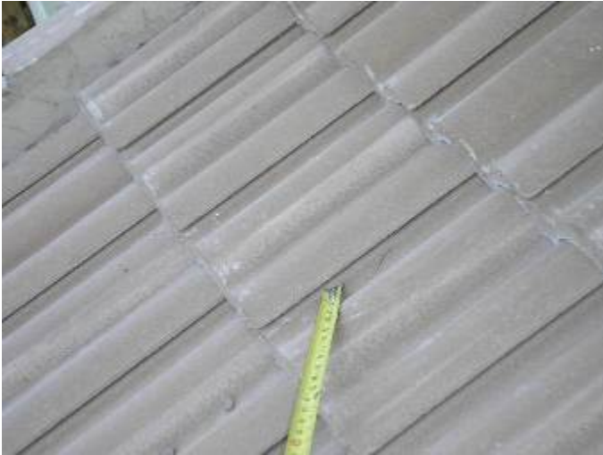
There were several broken tiles on the roof over the rear patio. There should not be any broken tiles on the new roof. The tiles need to be removed & replaced.
