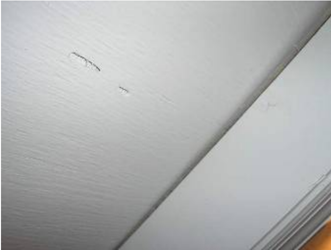
There was damage at the attic access cover.
