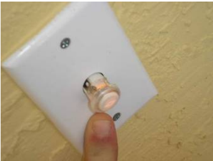
The door bell switch was loose at the wall.
