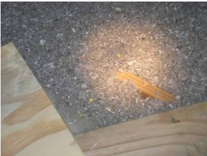
There were some locations where the attic insulation was not the correct depth. Less than 4 inches at this location.
