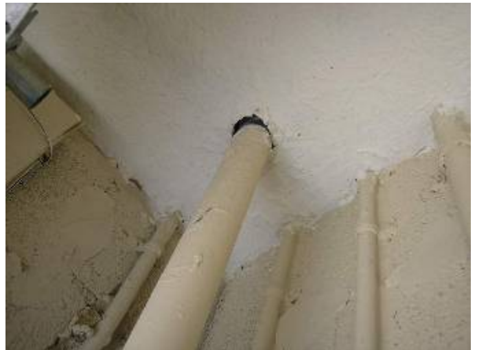
The drywall is not correctly sealed around the sprinkler system piping at the garage ceiling.
