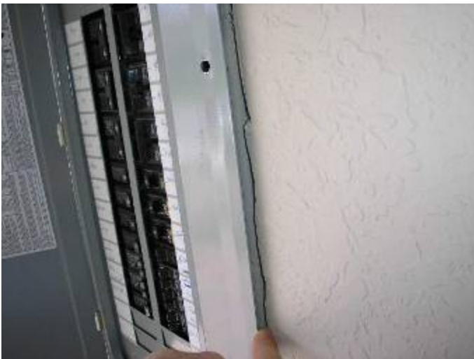
Several screws were missing from the electric panel cover in the garage.
