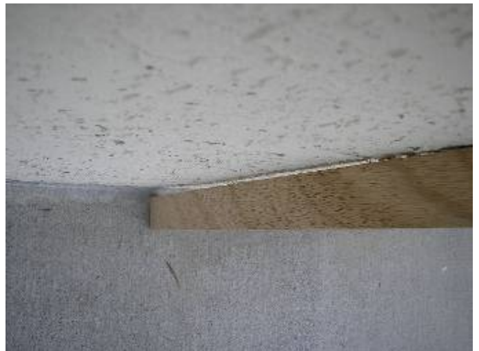
The stucco at some at the walls is concave or curved in & does not appear to be the correct thickness. §2509.1.1, ASTM C 926
