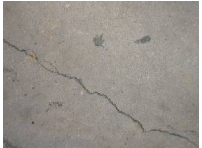
There is a crack in the concrete at the garage floor. The crack should be sealed & monitored for signs of further settlement.
