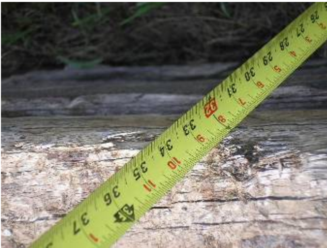
The railroad tie wall is almost 3 feet high, has no railing & presents a tripping/safety hazard at the back of the building. FBC §1617.4.4
