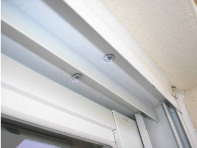
Some of the screw anchors not completely set & not sealed to prevent water & pest intrusion at the sliding glass door frame. FBC §13-606.1.ABC.1.2., §1707.4.4.1
