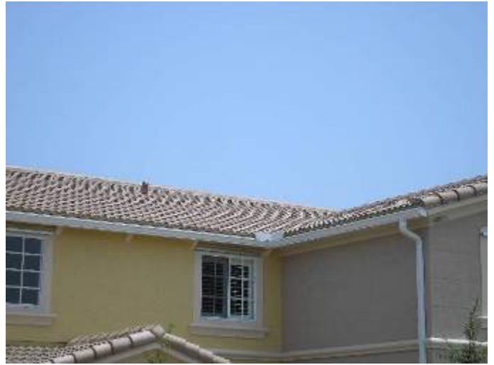
We were not permitted to go on or view the roof from a ladder. We recommend a complete review of the roof after closing.
