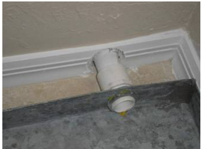
The wall is not completely sealed around the washer over flow pipe.
