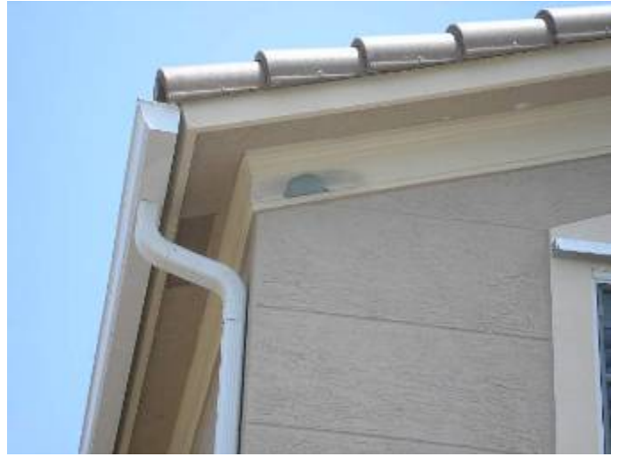
There were areas in need of touch-up & finish paint.
