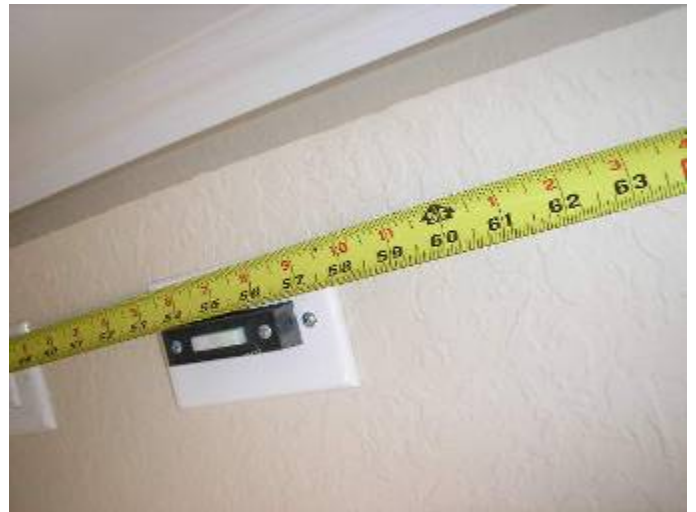
The switch is required to be at least 5 feet above the floor.
