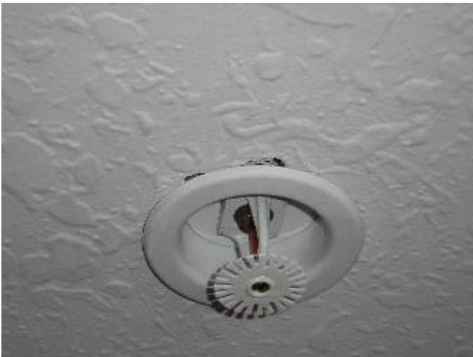
The drywall is not completely sealed around some of the sprinkler heads.
