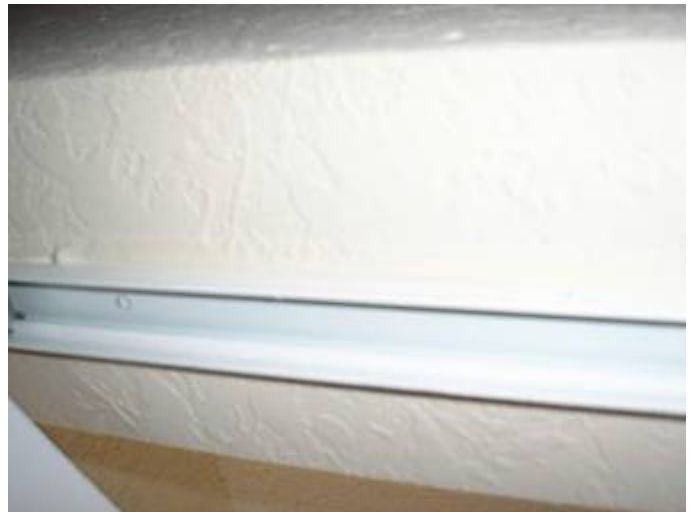
Some of the screws have not been installed at the closet door top tracks.
