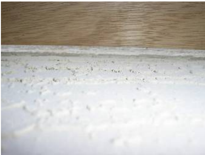
Some of the stucco work appears to be uneven, curved in/concave & not the proper depth. ASTM C 926, §2504.2 §1403.1.3
