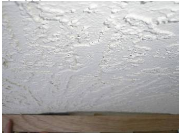
We recommend core sampling to verify the thickness of the exterior stucco & compliance with ASTM C 926.
