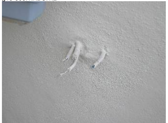
There were unconnected, low voltage wires at the wall at the front entryway.
