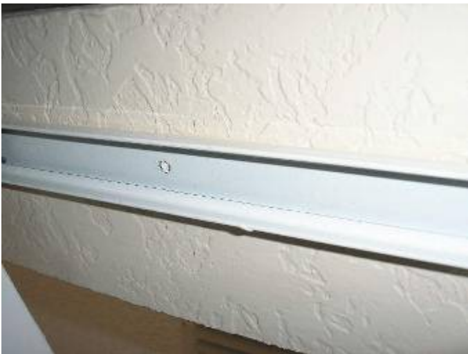
Some of the screws have not been installed at the closet door top tracks.
