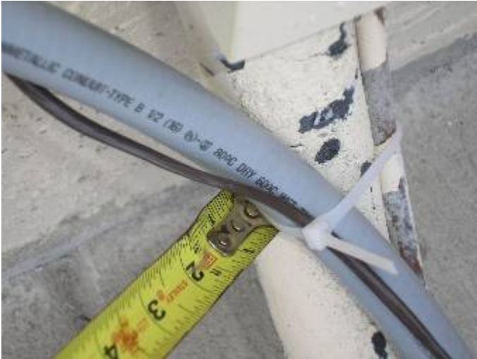
The clear or white plastic tie straps are not designed for use at exterior locations. The straps will be damaged by the U.V. sunlight.
