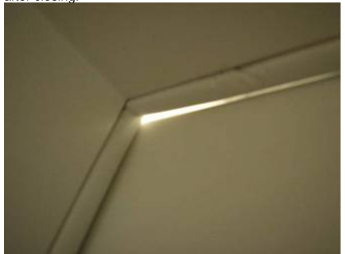
There are gaps with daylight & AC loss at the front door & frame. FBC §13-606.1.ABC.1.2
