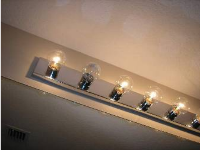
Some of the bulbs are not installed or burnt out.
