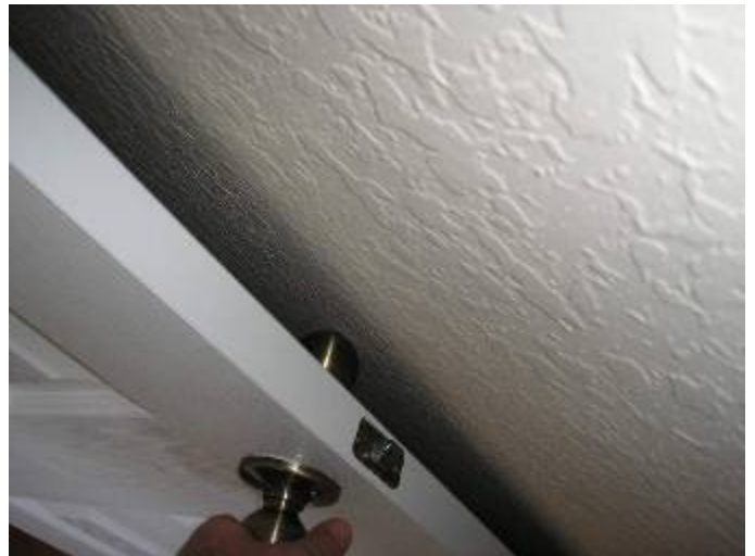
Some of the door stops are not working or installed correctly.
