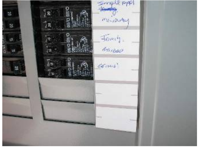
The circuits are not all completely identified to indicate the location of service. 2002 NEC225.37
