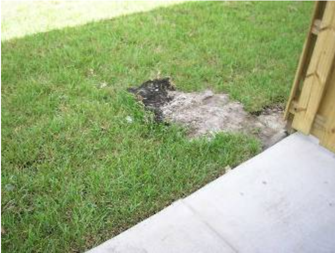
The sod installation was incomplete.
