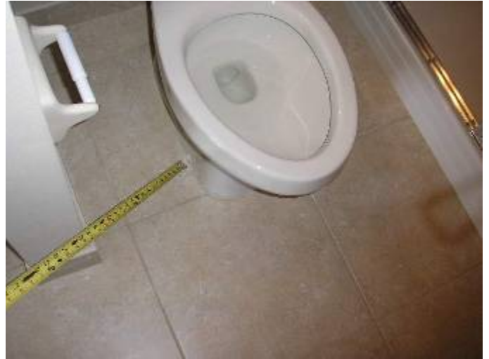
The toilet is loose & not correctly secured or sealed at the 2 nd floor guest bathroom floor.
