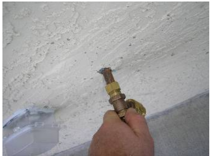
The wall is not correctly sealed around the hose bibb supply piping. FBC §13-606.1.ABC.1.2
