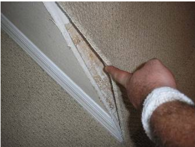
The drywall is not finished & the carpet is not correctly secured in the master bedroom closet.
