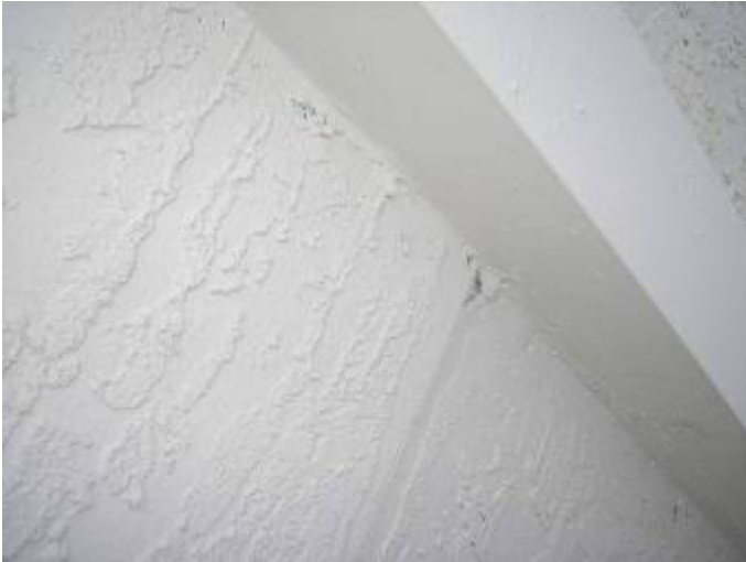
Some of the stucco work appears to be uneven, curved in/concave & not the proper depth. ASTM C 926, §2504.2 §1403.1.3
