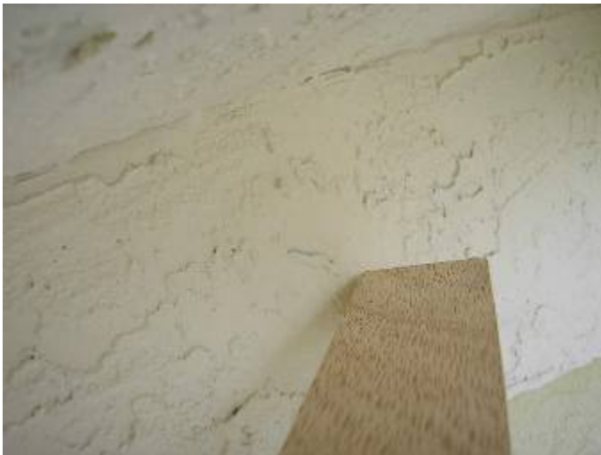
There is stucco visible & not completely painted at areas of the exterior.
