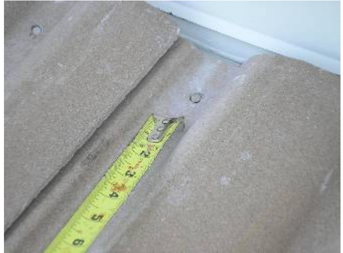
There are exposed nails at the wall abutment tiles. The nails should be covered to prevent expansion & contraction from the heat of the sun.
