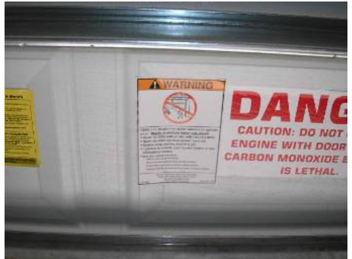
The warning label needs to go on the wall by the auto door opener switch §M304.1
