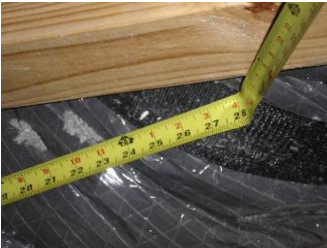
Some of the AC ductwork is not correctly installed or supported in the attic. The ducts are sagging & also need to be supported within 18" of connections or fittings.
