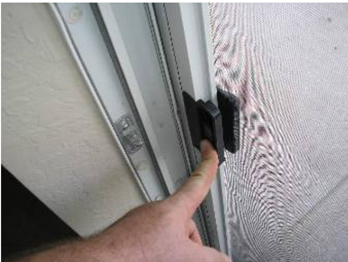
The sliding screen door sticks at the lock/latch.
