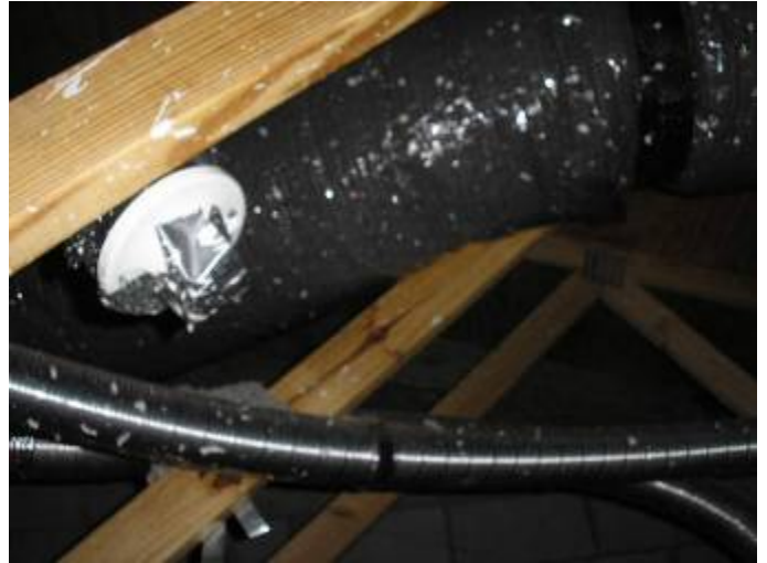
There was duct tape over the light fixture in the attic.
