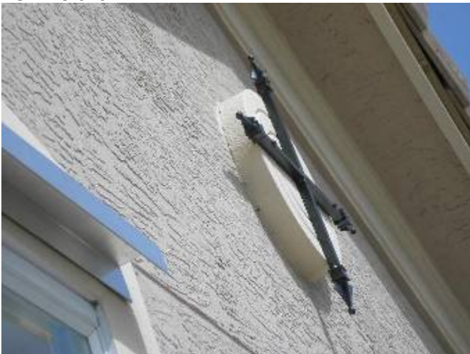
The ornamental trim is not completely sealed at the exterior wall to prevent water & pest intrusion. FBC §13-606.1.ABC.1.2
