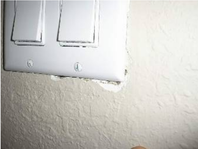
The drywall is not completely sealed around some of the switch & outlet covers.
