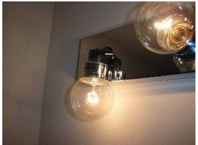
The bulb is hanging by the electrical wiring at the 2 nd floor guest bathroom light fixture.
