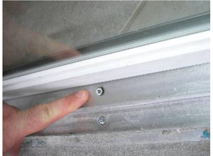
Some of the screw anchors not completely set & not sealed to prevent water & pest intrusion at the sliding glass door frame. FBC §13-606.1.ABC.1.2., §1707.4.4.1 Florida Building Code (FBC)
