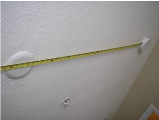
The smoke detector is located too close to the ceiling fan junction box in the bedroom. 3' clearance from the fan blade tips should be allowed.
