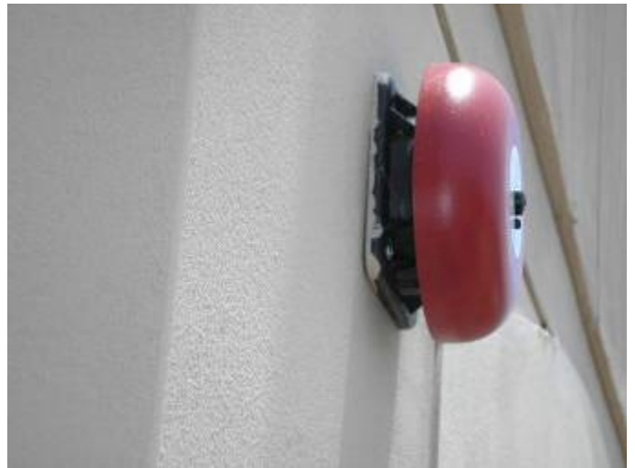
The base of the fire alarm bell is not correctly sealed at the exterior wall to prevent water & pest intrusion. FBC §13-606.1.ABC.1.2
