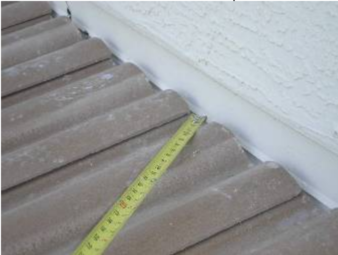
The roof wall abutments have not been correctly pointed up with mortar at the back patio. §1518.8, R118-3.13
