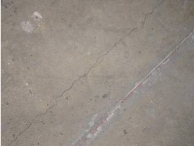
There is a crack in the concrete at the garage floor. The crack should be sealed & monitored for signs of further settlement.
