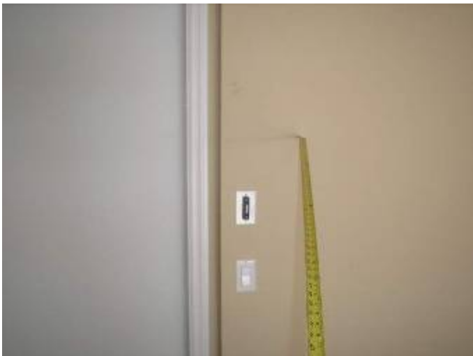
The warning label needs to go on the wall by the auto door opener switch §M304.1
