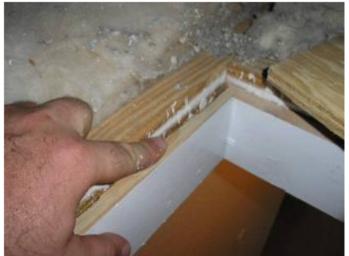
The attic access hatch is not sealed or gasketed as required. §13-606.1.ABC.1.2.3
