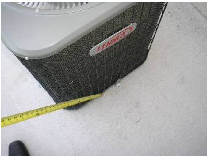
The A/C condenser is not secured properly. There are not enough straps at the base of the unit. FBC M301.13.1
