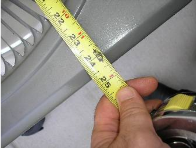
The A/C condenser is not secured properly. There are not enough straps at the base of the unit. FBC M301.13.1
