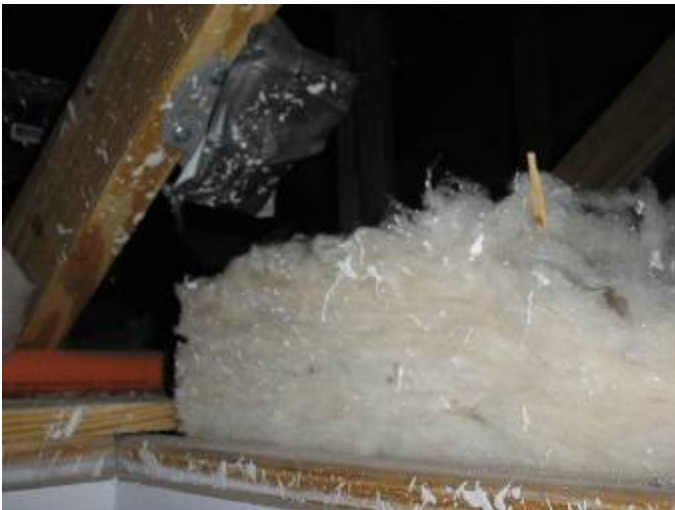
There was duct tape over the light switch in the attic.
