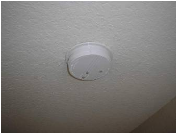
The smoke detector was chirping, indicating it needs a new battery.
