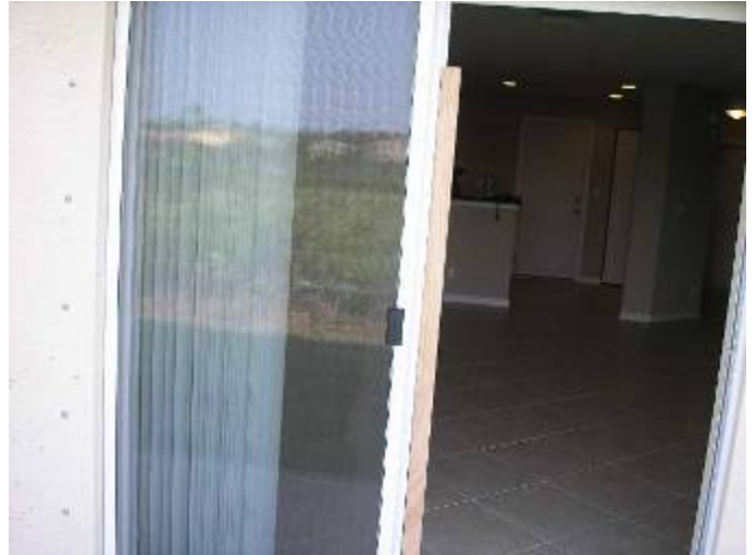
A straight edge was verified at the sliding door & used to check the exterior walls.
