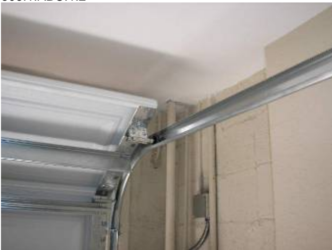
The drywall is not correctly sealed around the sprinkler system piping at the garage ceiling.
