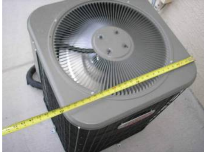
The A/C condenser is not secured properly. There are not enough straps at the base of the unit. FBC M301.13.1
