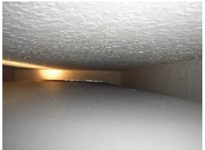
Some of the drywall was not painted or correctly finished inside the AC mechanical closet.
