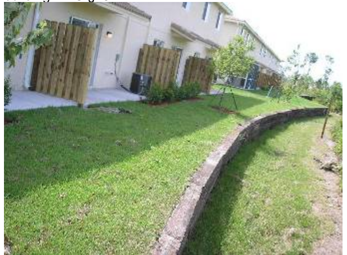
The railroad tie wall is almost 3 feet high, has no railing & presents a tripping/safety hazard at the back of the building. FBC §1617.4.4
