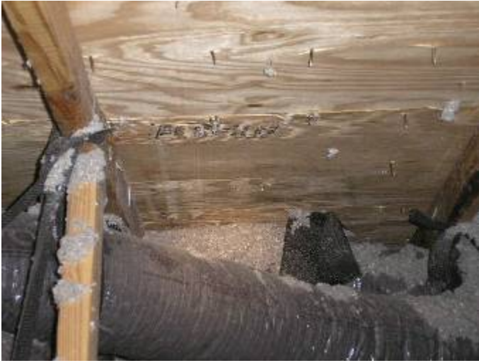
The AC duct appears to be wedged against the roof sheathing and tile nails. We were not permitted to leave the ladder to verify this & other conditions.
