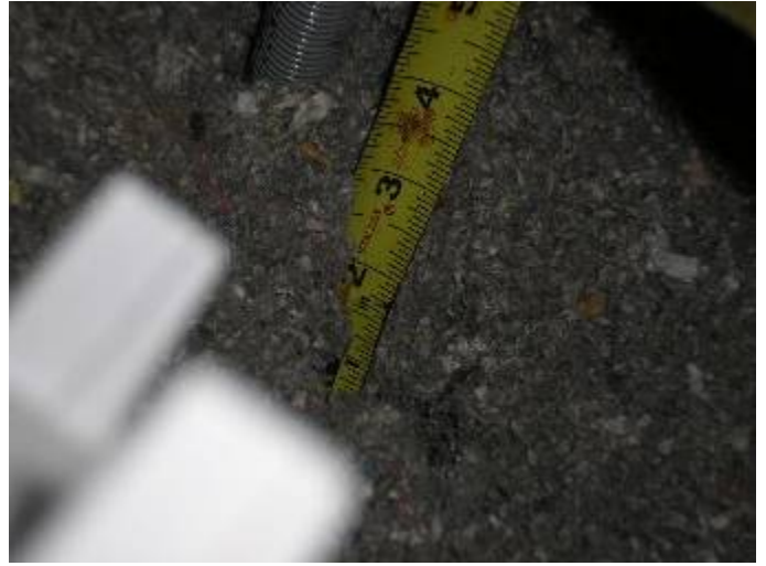
There were some locations where the attic insulation was not the correct depth.
