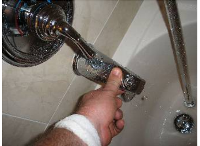
The tub spout is loose or not correctly secured at the wall.
