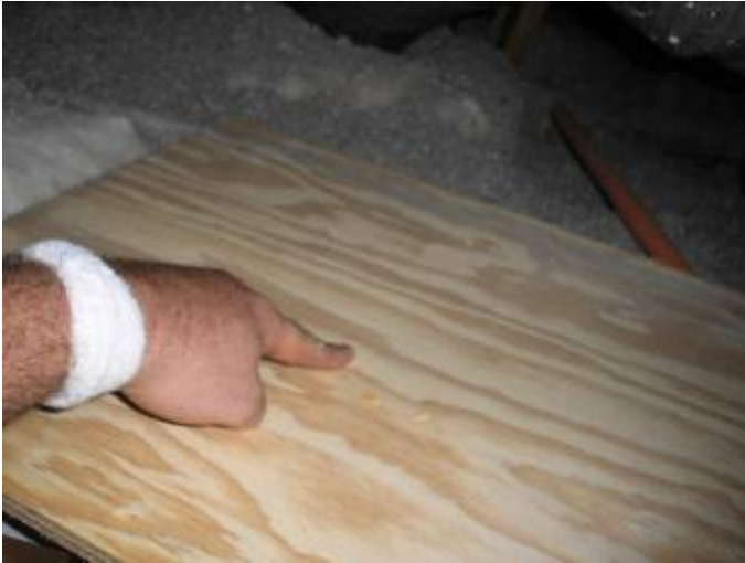
There is no insulation at the back of the attic hatch cover.
