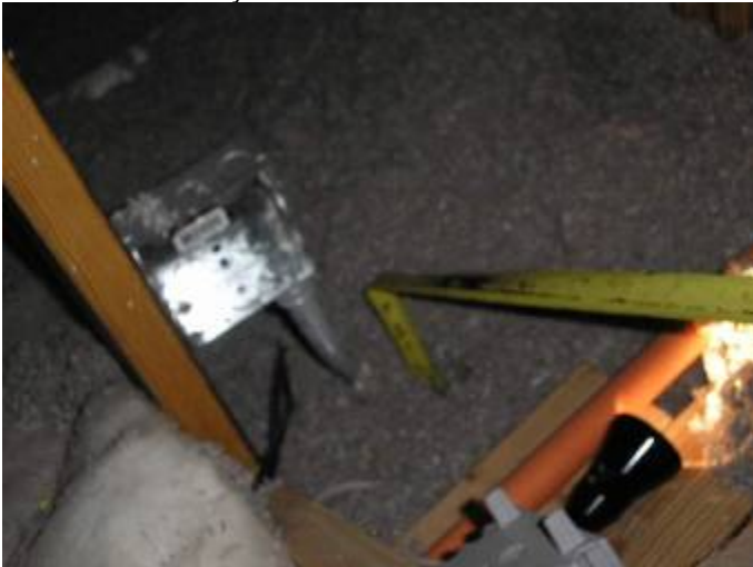
There were some locations where the attic insulation was not the correct depth.
