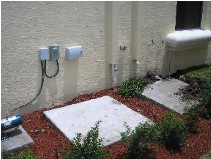
The AC units were not in place.
