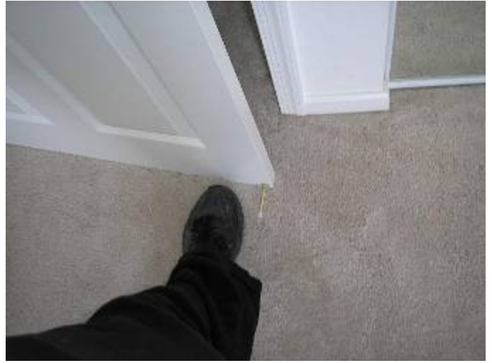
The door drags on the carpet & needs to be adjusted or undercut.
