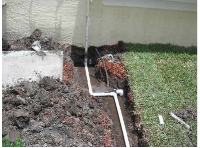
Some of the water piping installation was not completed at the time of the inspection.
