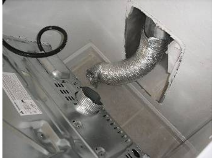
The foil dryer vent duct material is a fire hazard per UL & manufacturer. Replace with rigid or heavy flex duct material in accordance with manufacturer's instructions.
