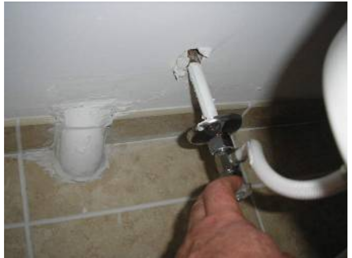
Why is the plumbing waste line coming through the wall & floor? Verify this installation with the architects drawings.
