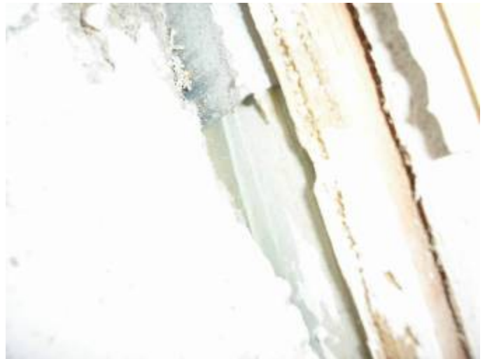
The trim is not correctly sealed at the bottom at locations around the wall in the garage. §13-606.1.ABC.1.2
