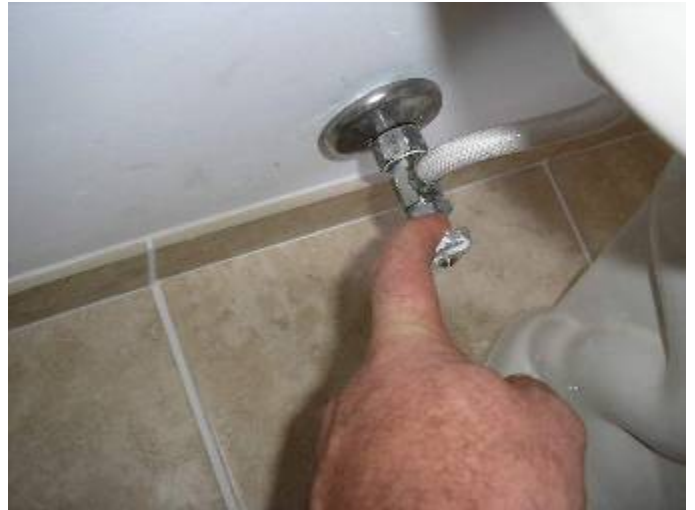
Some of the plumbing supply piping is loose & not correctly secured at the sink cabinets & behind the walls at the water closets (toilets).
