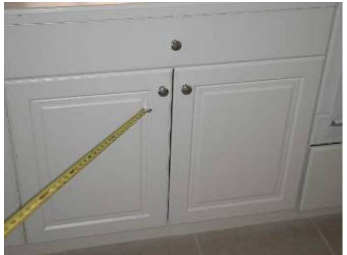
Some of the gaps between the cabinet doors are uneven or different in size from adjacent cabinets.
