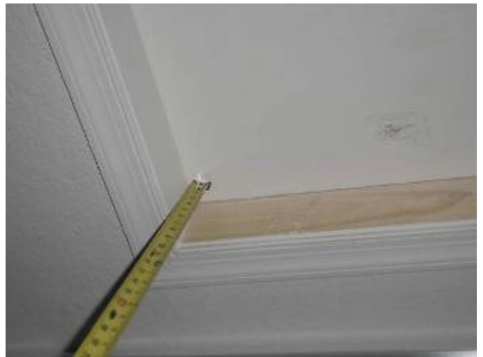
There is no air tight seal or gasket at the attic access opening as required.
