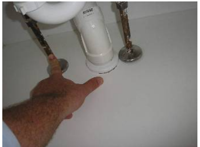
The supply piping is not correctly secured & the opening in the bottom of the cabinet shelving is not correctly covered by the escutcheon.
