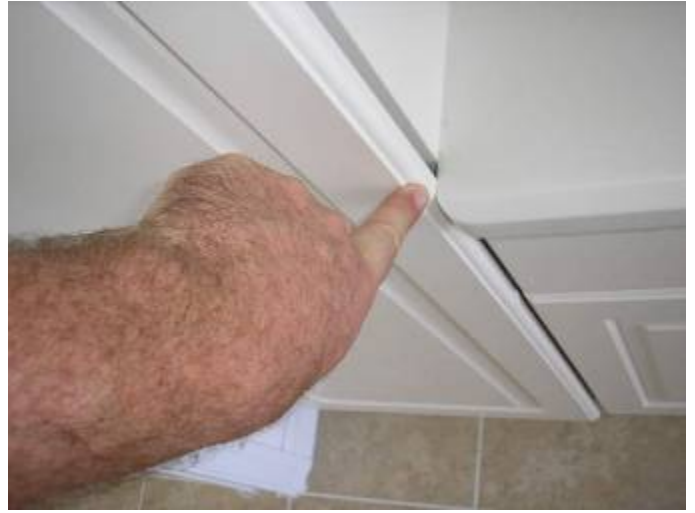
The cabinet door sticks & rubs against the lavatory sink counter top in the guest bathroom.
