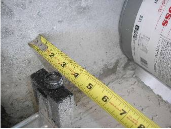
The garage vehicle photo eye sensors are located too close to the floor. The photo eyes should be 6" above the floor per manufacturer's installation instructions.
