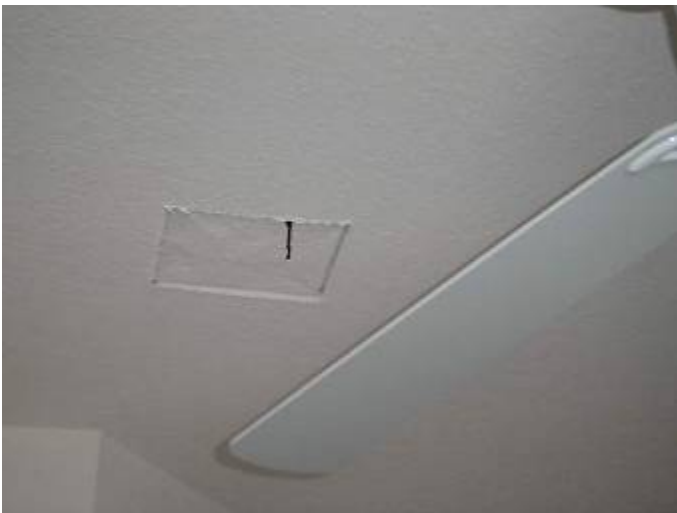
Some of the AC vent registers were not yet installed at ceiling locations.
