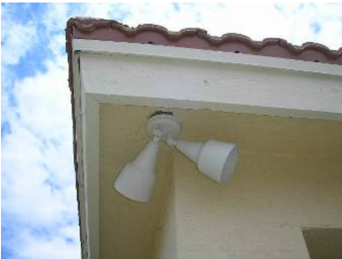
The exterior light fixtures are not completely sealed or gasketed at the base as required and there are openings into the wiring boxes & exterior wall cavities. NEC 410.4
