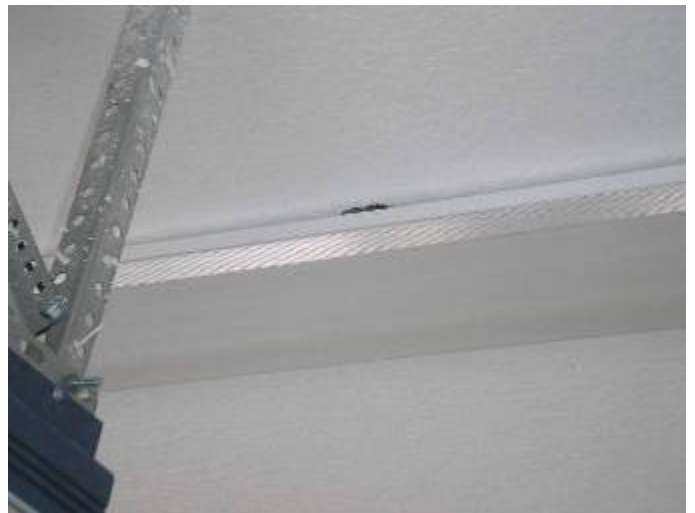
The drywall is not correctly sealed around the junction box for the garage light fixture.
