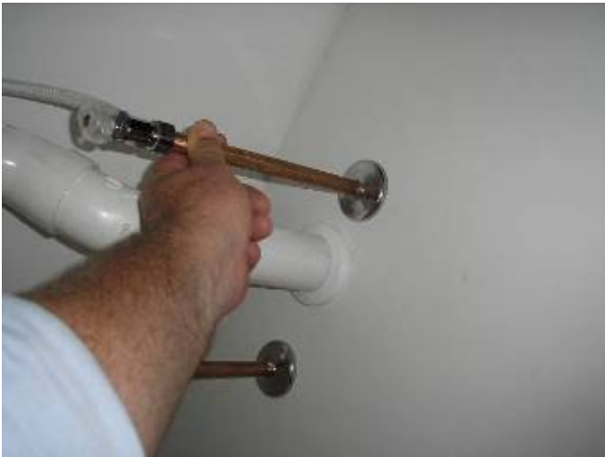
Some of the plumbing supply piping is loose & not correctly secured at the sink cabinets & behind the walls at the water closets (toilets).
