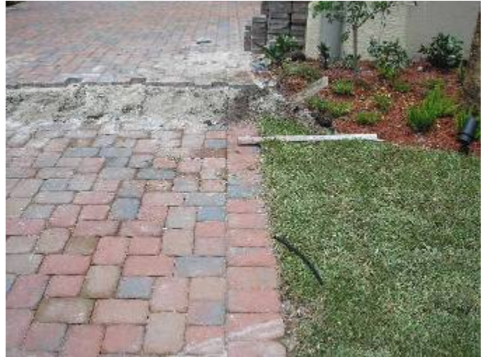
Some of the driveway has been taken up for plumbing/sprinkler line installation.
