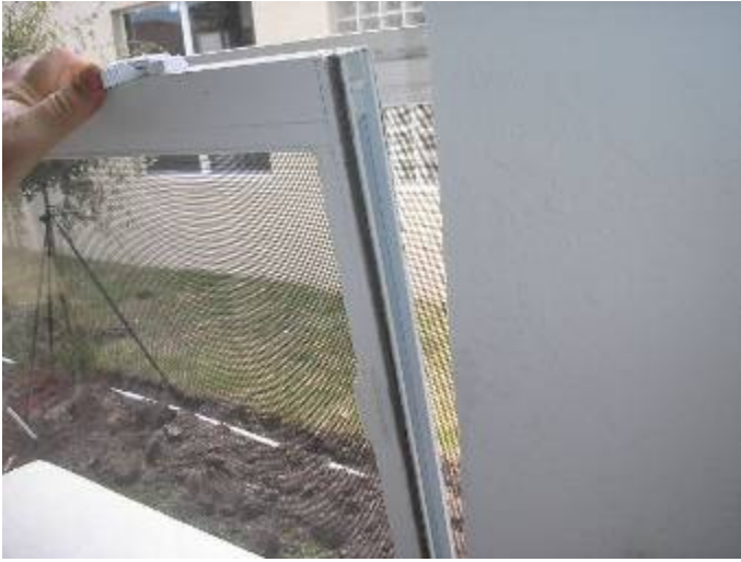
The window is not correctly secured in the frame at the front entryway.
