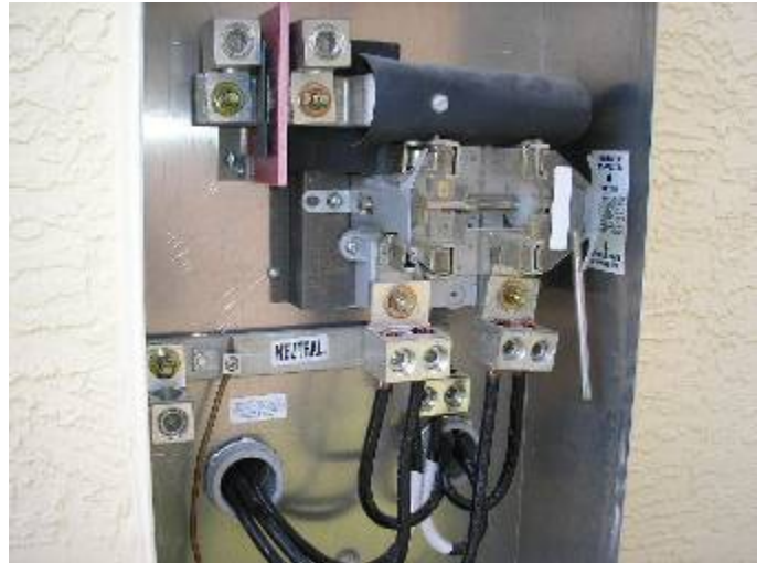
The meter has not been installed. There was no electrical power at the time of the inspection.
