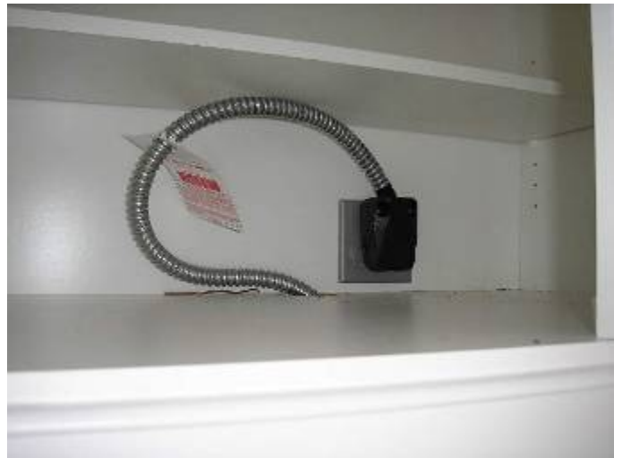
A plug & receptacle are not permitted for the wall oven electric supply. §M304.1
