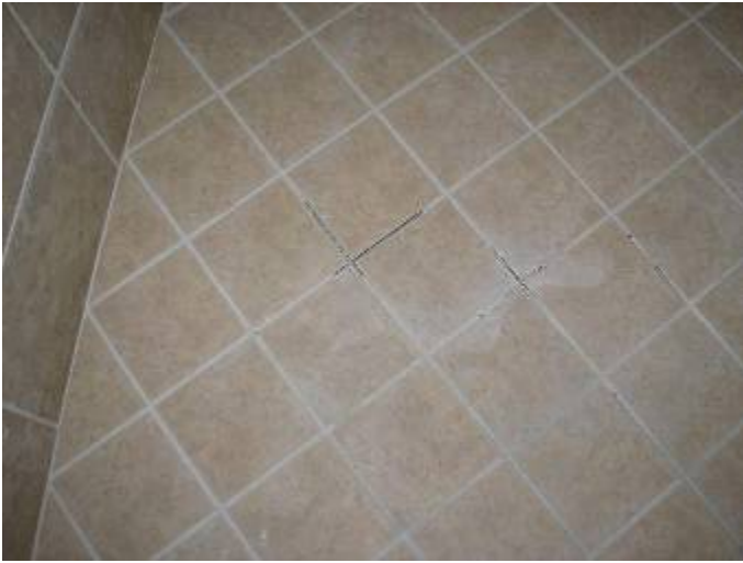
Some of the tile grout has not been installed at the shower floor & walls.
