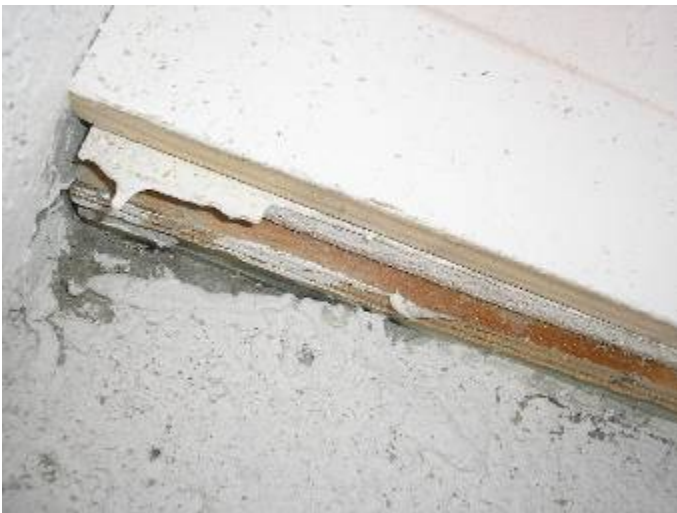
The trim is not correctly sealed at the bottom at locations around the wall in the garage. §13-606.1.ABC.1.2
