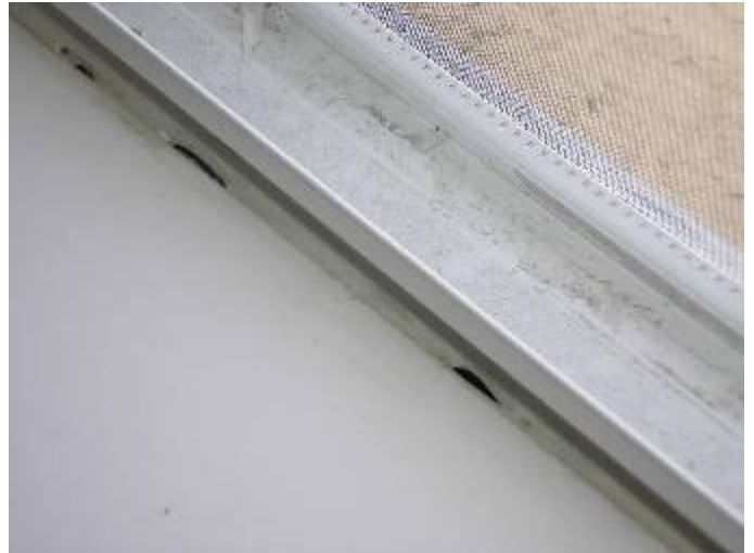
Some of the window sills have not been correctly sealed around the frames.
