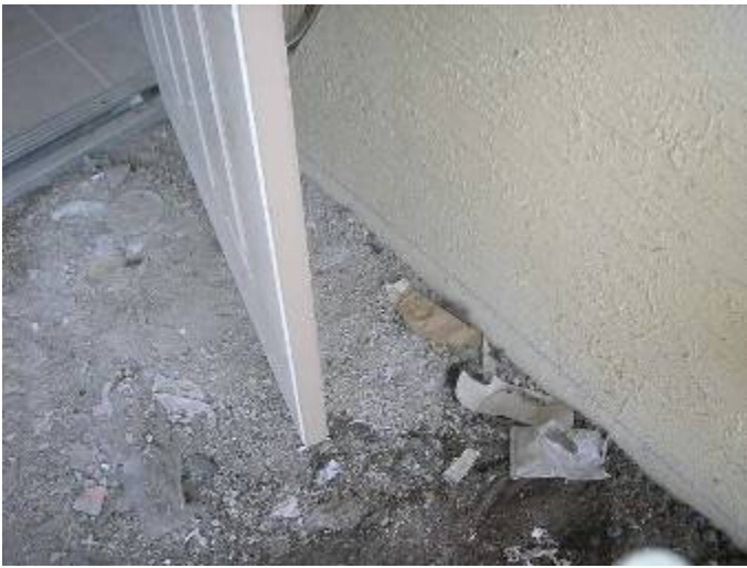
There are no door stops installed at the front entryway.
