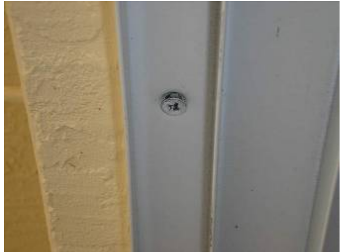
Some of the screw anchors & frames are not correctly set or sealed to prevent water & pest intrusion around the sliding glass doors. §13-606.1.ABC.1.2
