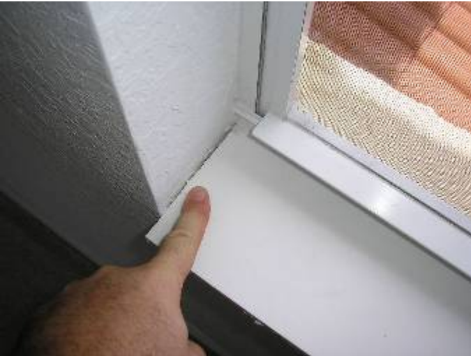
Some of the window sills are not completely sealed at the window frames & side walls.
