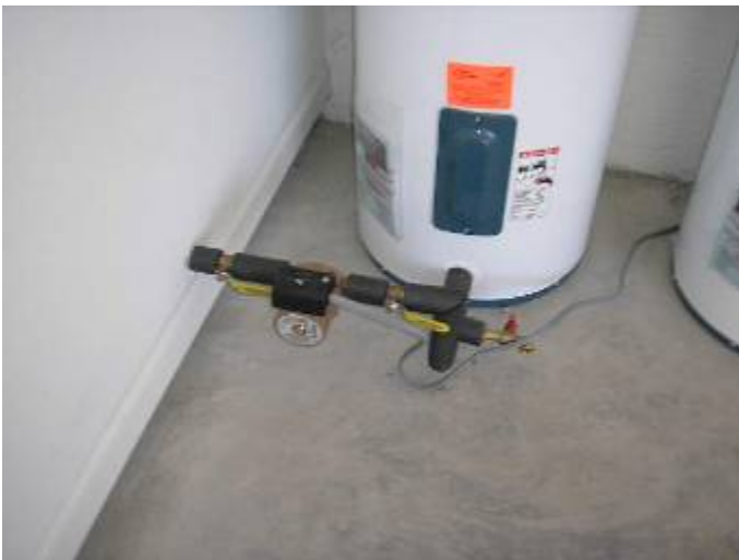
The circulating pump & piping are not correctly supported at the water heater.
