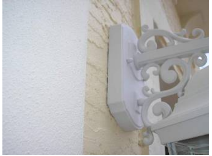
The exterior light fixtures are not completely sealed at the base as required or gasketed and there are openings into the wiring boxes & exterior wall cavities. NEC 410.4
