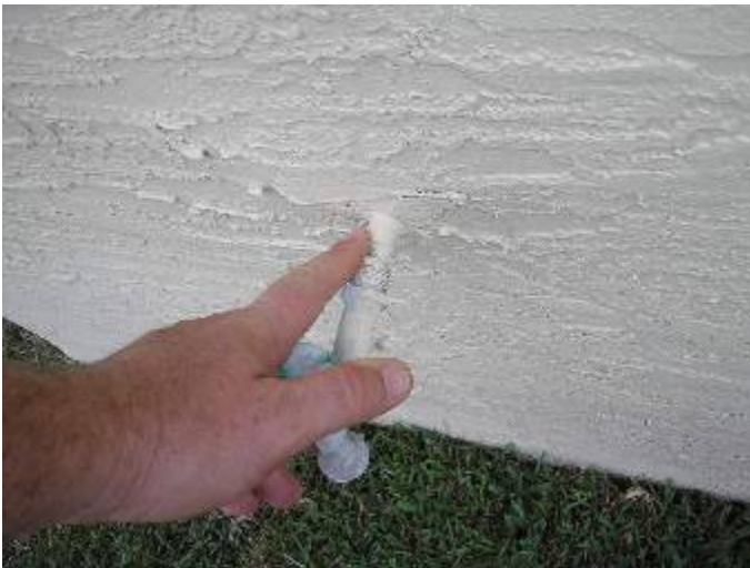
The hose bib supply piping was not correctly secured or sealed at the wall. Sheathing is required to protect the copper piping & was not visible. §P305.1
