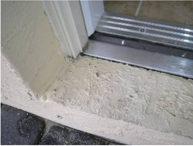
The wall stucco, door frame & threshold are not correctly sealed to prevent water & pest intrusion at the rear exterior hinged door. §13-606.1.ABC.1.2, §1403.1.3
