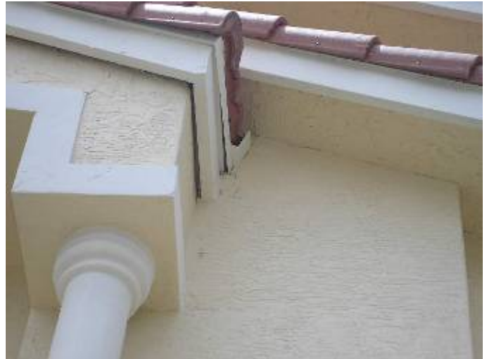
The flashing does not appear to be correctly sealed at the stucco wall.
