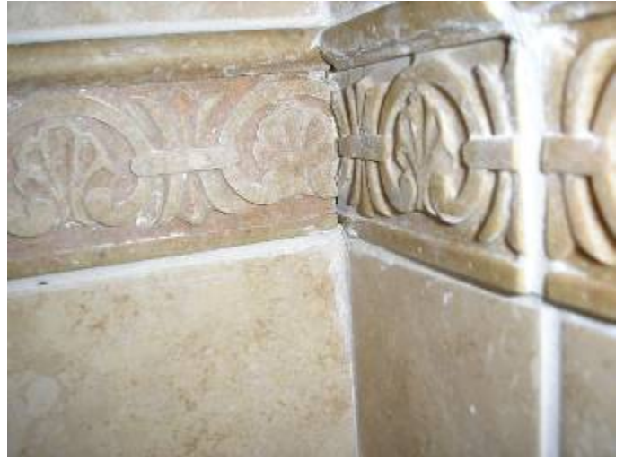
Some of the tile grout has not been installed at the shower floor & walls.
