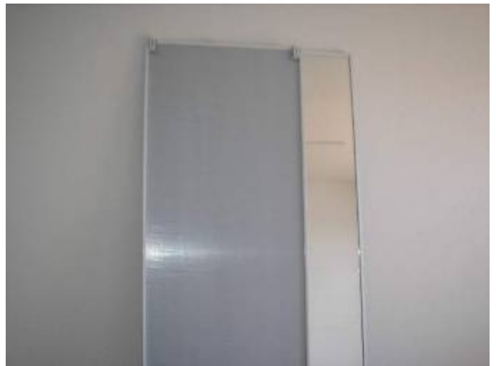
Some of the interior room & closet doors have not yet been installed.
