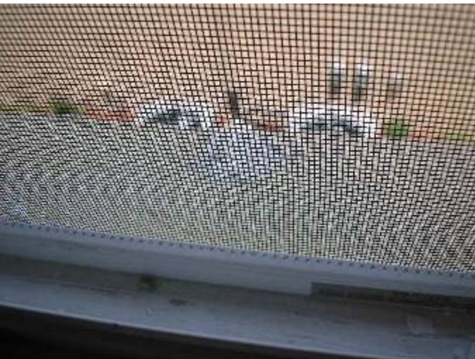
There is construction debris that needs to be removed on the exterior window sills.
