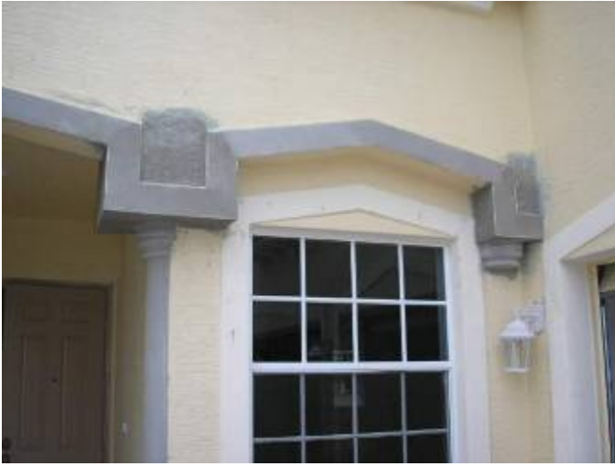
The paint work was incomplete at the time of the inspection.
