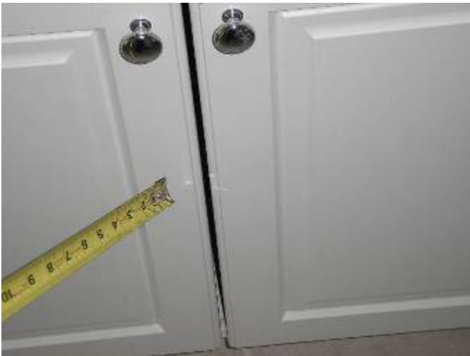
Some of the gaps between the cabinet doors are uneven or different in size from adjacent cabinets.
