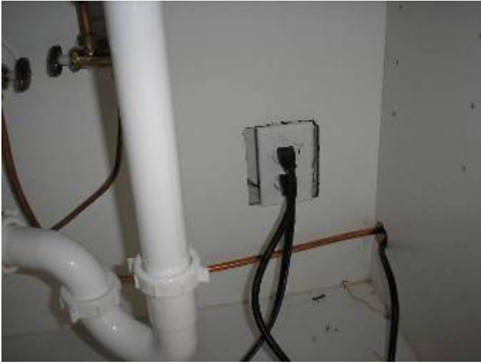
The back of the cabinet is not correctly cut for the electrical outlet junction box in the kitchen under the sink.
