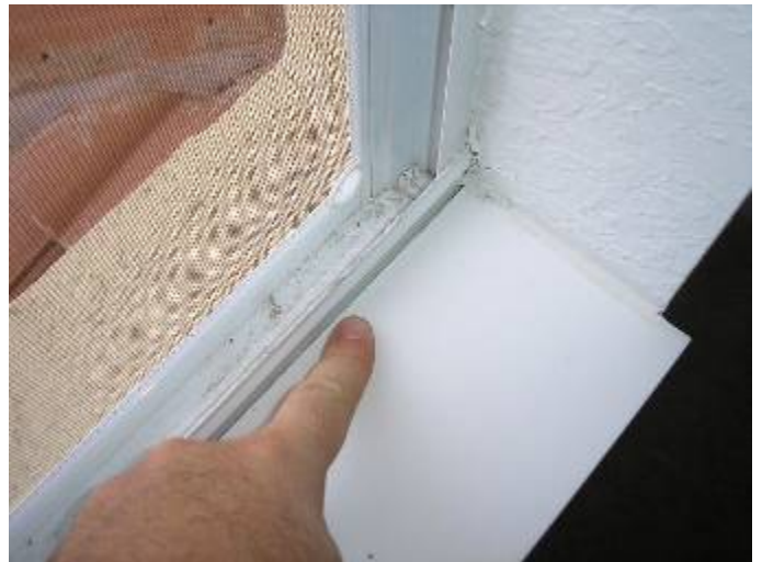
Some of the window sills are not completely sealed at the window frames.
