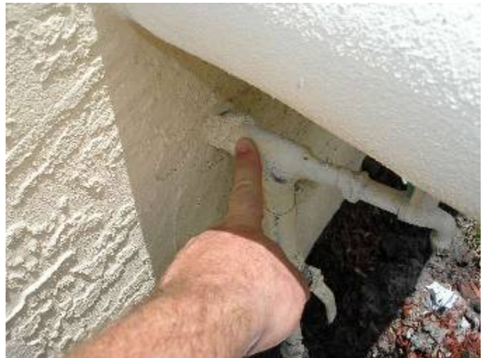
The main water supply piping was not correctly sealed at the wall. Sheathing is required to protect the copper piping & was not visible. §P305.1
