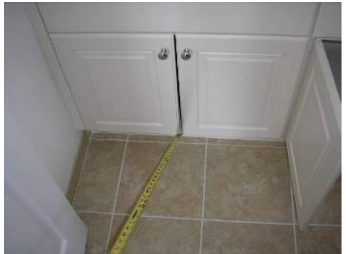
Some of the gaps between the cabinet doors are uneven or different in size from adjacent cabinets.
