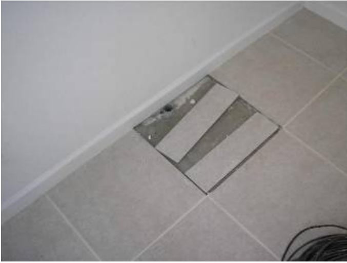
There is an open ended conduit & the floor tile has been removed at this location...
