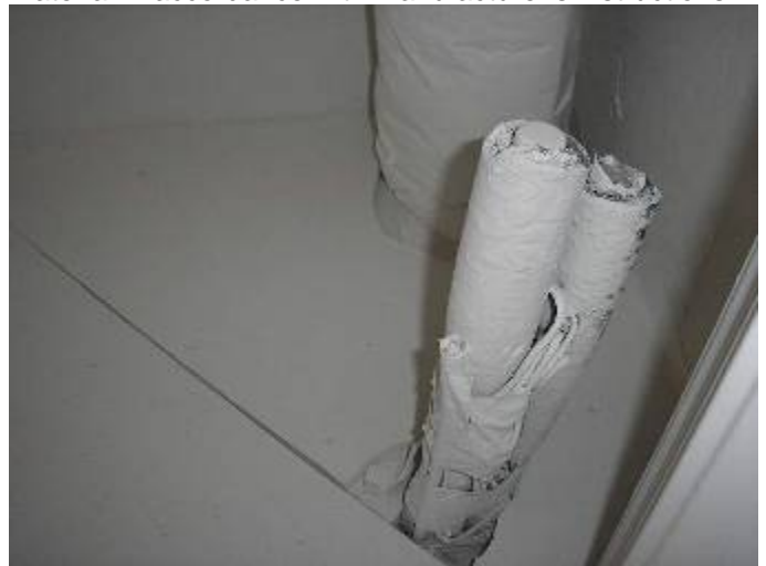
The AC mechanical closets are not completely sealed as required. The air handlers have not yet been installed.
