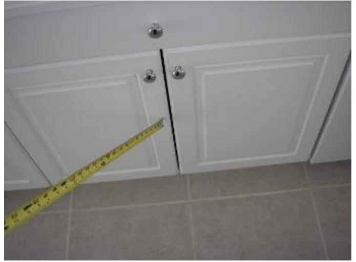
Some of the gaps between the cabinet doors are uneven or different in size from adjacent cabinets.
