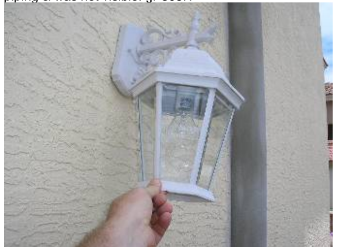
The fixture is not correctly secured or sealed at the exterior wall at the front of the house. 2002 NEC 410.4
