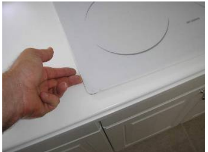
The cook top is not correctly secured to the countertop.
