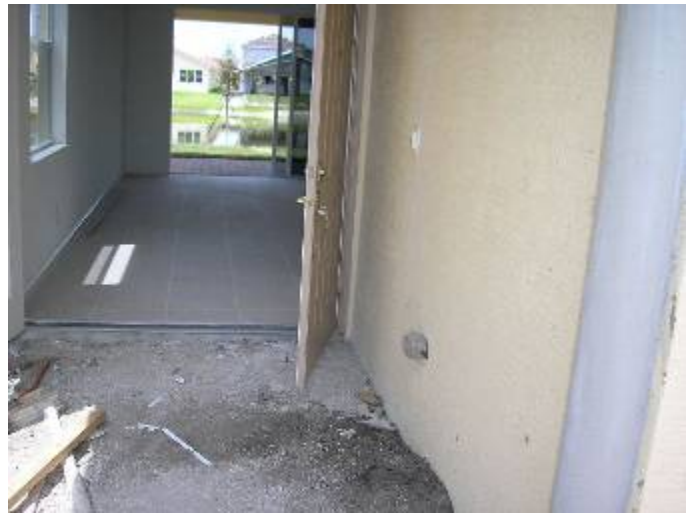
There are no door stops installed at the front entryway.
