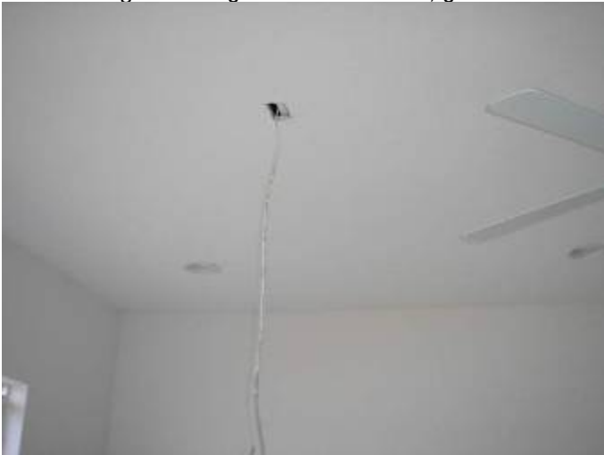
Some of the electrical fixtures have not been installed.
