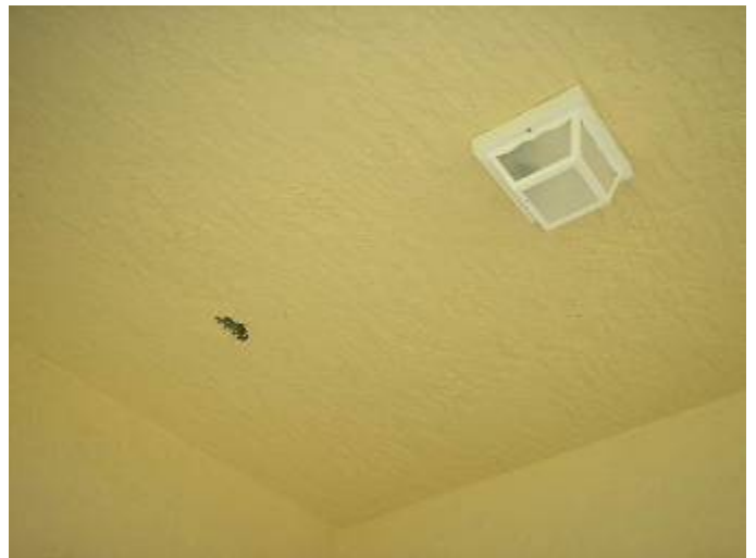
The cover is not installed at the junction box at the exterior ceiling. The light fixture is not completely sealed or gasketed at the base. 2002 NEC 410.4
