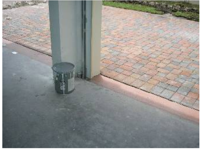
The garage vehicle photo eye sensors are located too close to the floor. §M304.1
