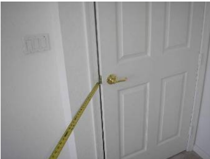
Some of the doors did not latch correctly at the 2 nd floor bedrooms.
