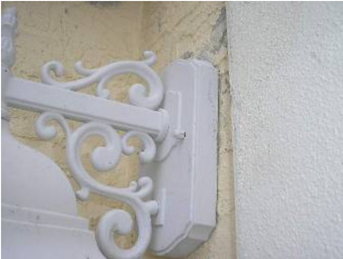
The exterior light fixtures are not completely sealed or gasketed at the base as required and there are openings into the wiring boxes & exterior wall cavities. NEC 410.4 2002 National Electric Code (NEC)
