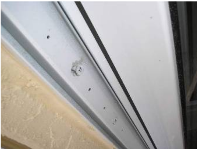
Some of the screw anchors & frames are not correctly set or sealed to prevent water & pest intrusion around the sliding glass doors. §13-606.1.ABC.1.2
