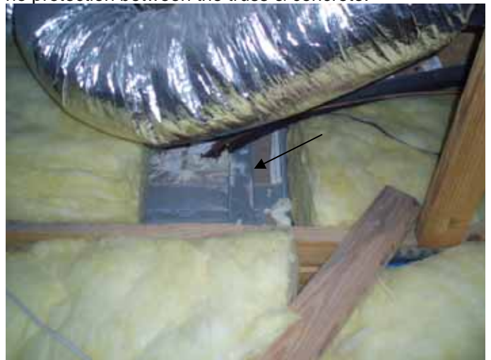
There were areas of the attic with displaced or missing insulation.
