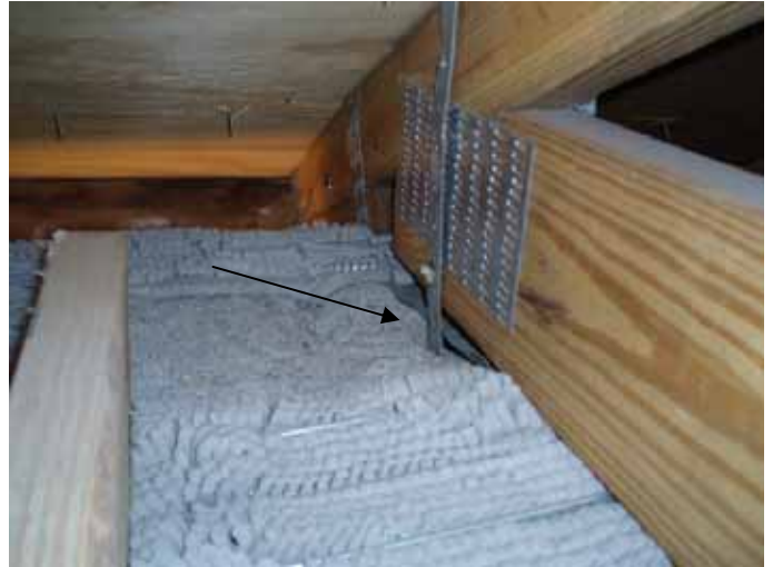
There were trusses that do not have 3 " bearing on a grout filled masonry cell or concrete at multiple locations. §2319.3
