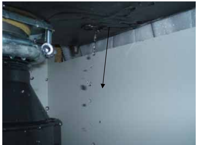
Most of the water was leaking from the right side of the kitchen sink.
