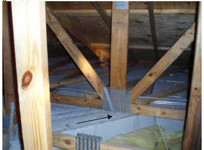
Location of the previous photos over the front entryway. There were trusses bearing on the concrete beams with no protection between the truss & concrete.
