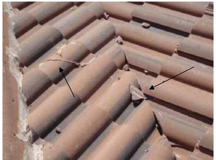
The broken roof tiles should be removed & replaced, not "glued" back together. All construction debris should be removed from the roof.
