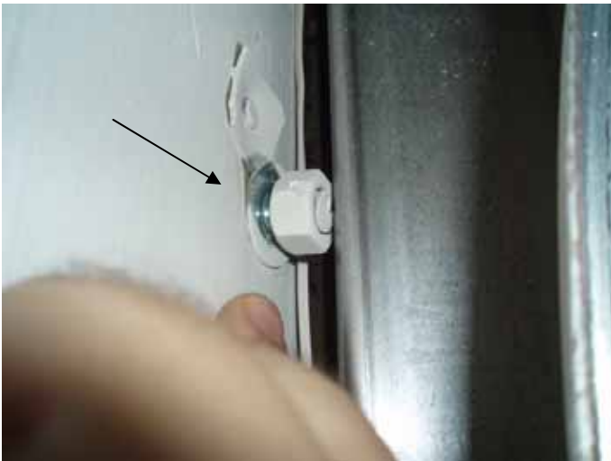
Some of the anchor nuts were loose at the garage door wood bucks.
