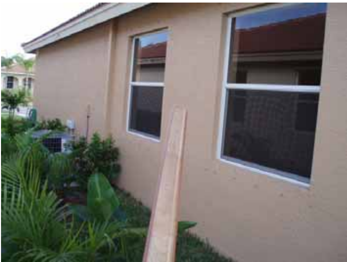
We recommend core sampling at these locations to verify the thickness of the exterior stucco & compliance with ASTM C 926.
