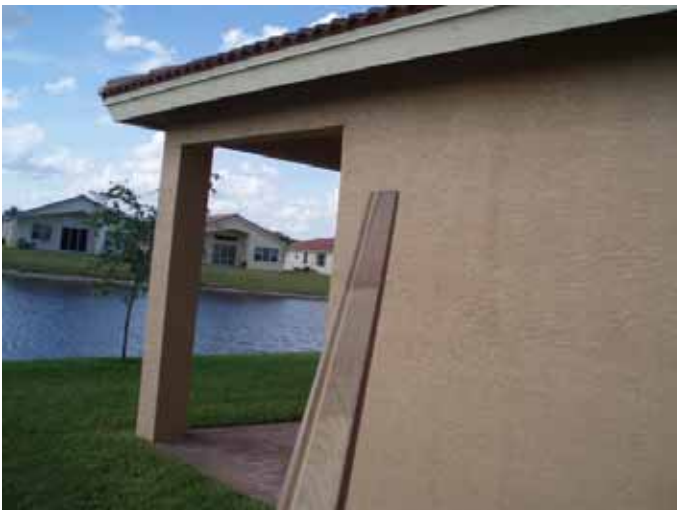
We recommend core sampling at these locations to verify the thickness of the exterior stucco & compliance with ASTM C 926.
