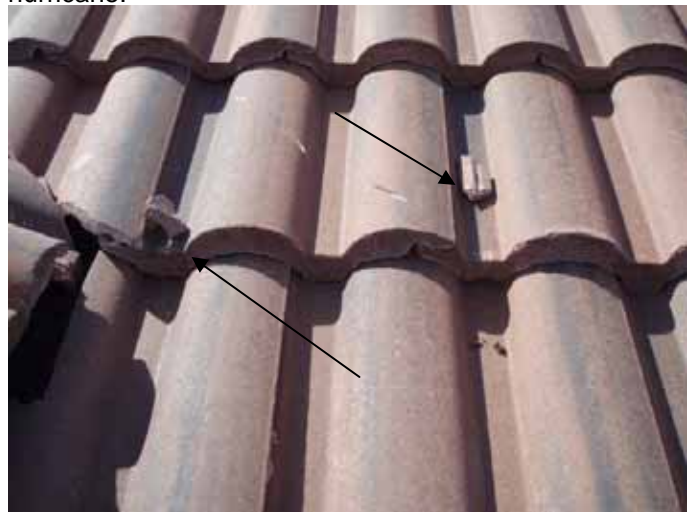
All nails & construction debris should be removed from the roof.
