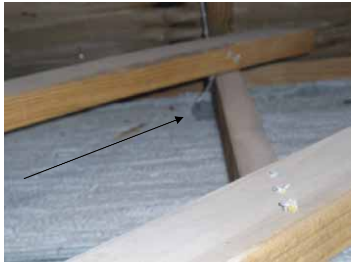
Many of the truss anchor straps were not correctly installed. The straps were offset too far from the trusses.
