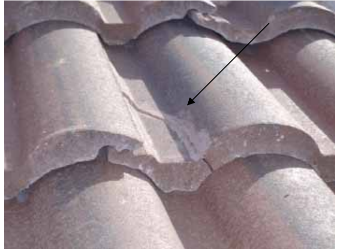
There were broken tiles that were incorrectly "glued" back together on the roof.
