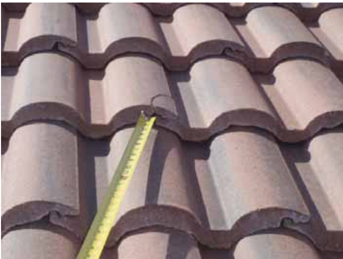
There were broken tiles that were incorrectly "glued" back together on the roof. The broken roof tiles should be removed & replaced, not "glued" back together.
