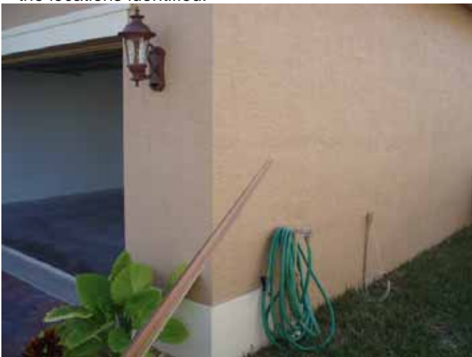
Location of the previous photo. We recommend core sampling to verify the thickness of the exterior stucco & compliance with ASTM C 926.
