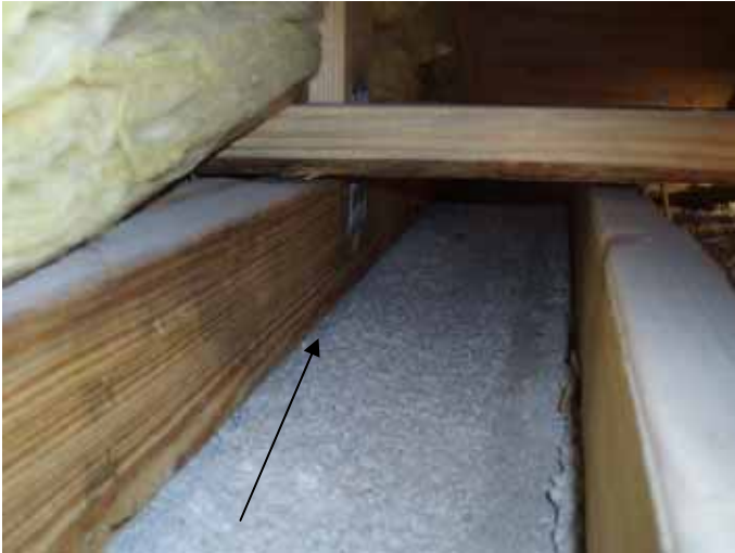
There were trusses bearing on the concrete beams with no protection between the truss & concrete.
