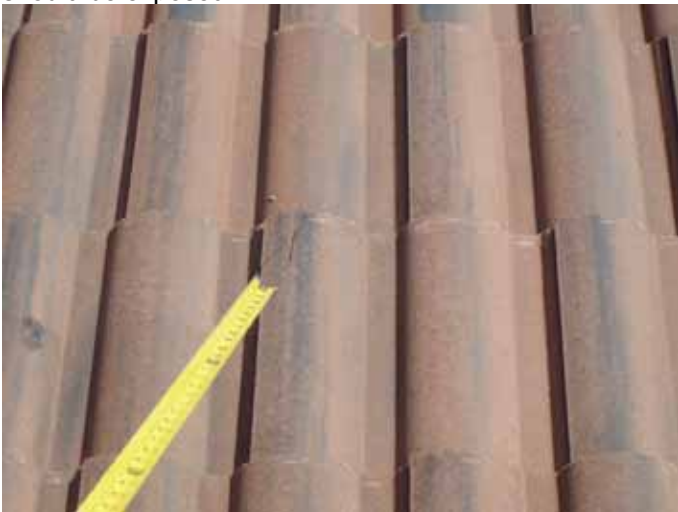
There were broken tiles that were incorrectly "glued" back together on the roof. The broken roof tiles should be removed & replaced, not "glued" back together.
