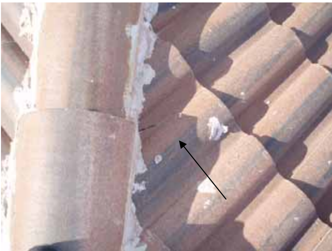
Loose & incorrectly installed roof tiles & construction debris can become windborne projectiles during a hurricane.
