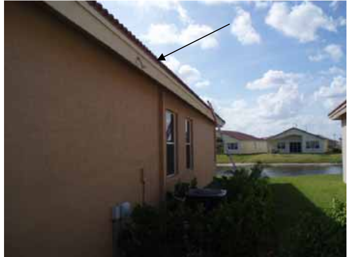
Location of the previous photo. The rain sensor was loose &/or not correctly installed to operate properly. The rain sensor should be parallel to the ground.
