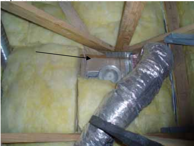
There were areas of the attic with displaced or missing insulation. All attic areas over conditioned space are required to be insulated. §13-604.1.A.1
