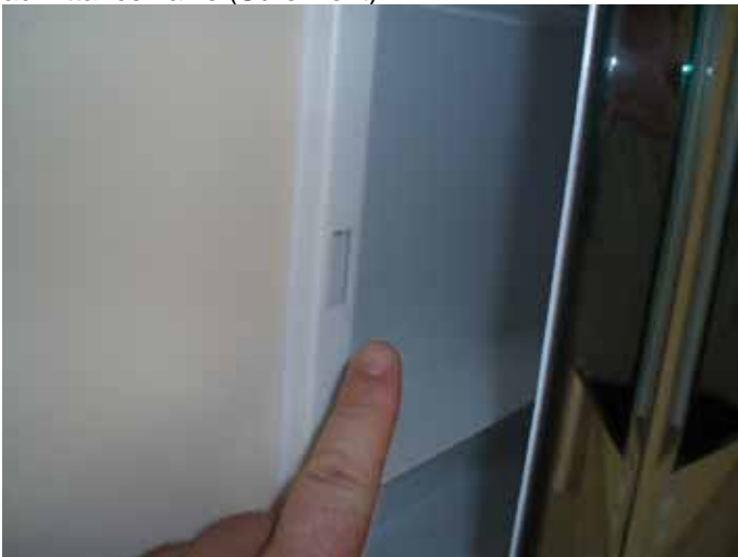
There was no magnetic latch at the medicine cabinet in the master bathroom.
