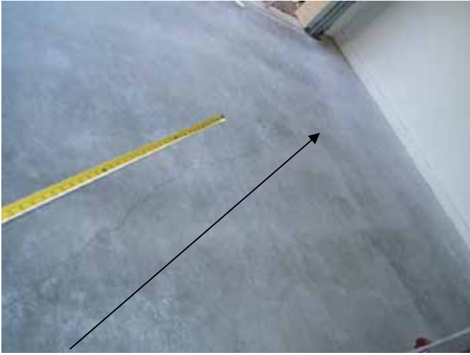
The cracks should be sealed & monitored for further shrinkage &/or settlement.
