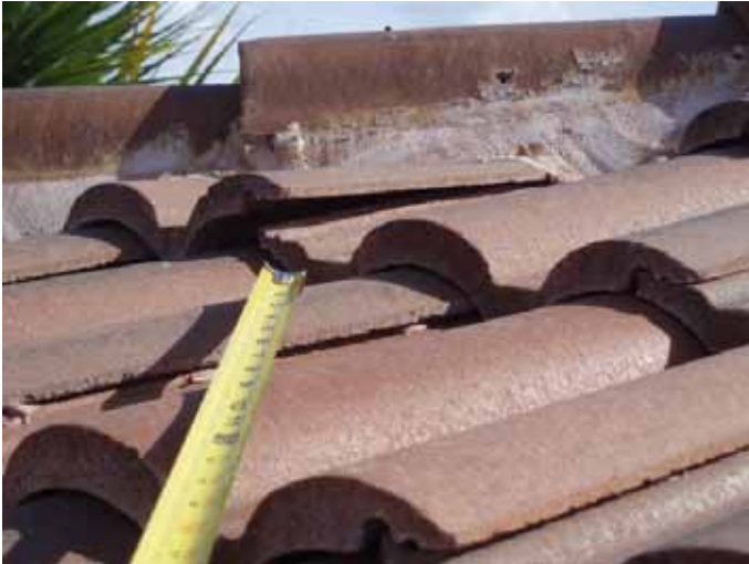
There were tiles that were not correctly set in place on the roof.
