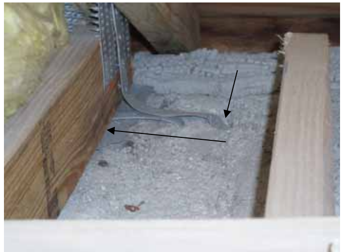
There should not be any slack in the truss anchor straps. Some of the straps were embedded 4" or more from the trusses.
