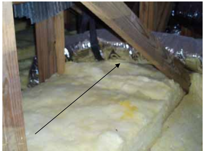
We recommend supporting the ductwork up off the attic insulation to help prevent problems associated with condensation.
