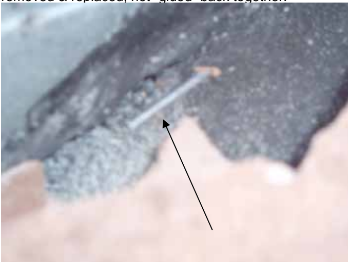
All nails & debris should be removed from the roof.
