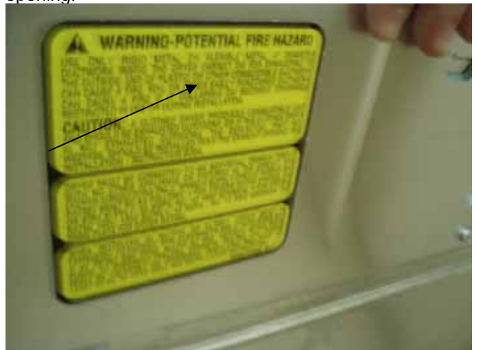
The manufacturer states the use of this duct can be a fire hazard. We recommend replacing the duct with a semi-rigid duct as per the CSPC article below.
