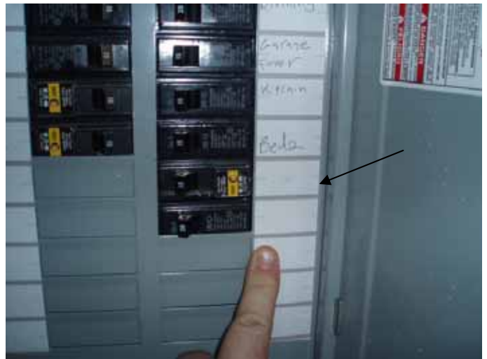
Some of the electrical circuits were not identified. All of the circuits in the main distribution panel should be correctly identified in the panel directory.
