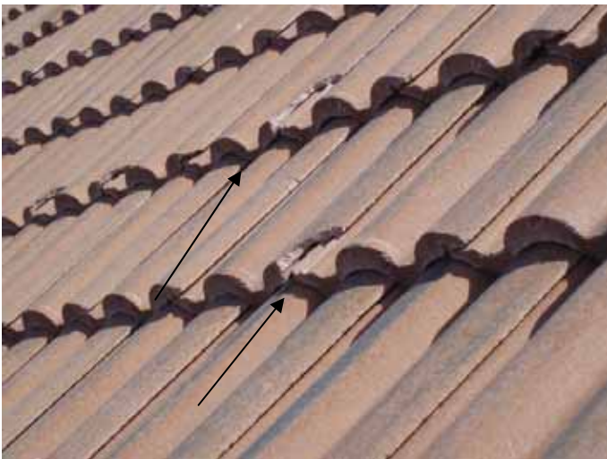
Loose & incorrectly installed roof tiles & construction debris can become windborne projectiles during a hurricane.
