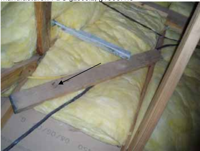
All construction debris should be removed from the attic.
