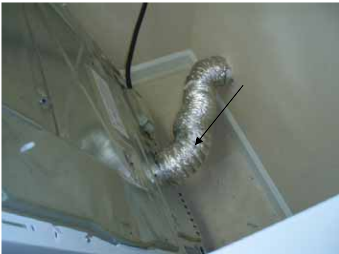
A thin foil vent duct was installed behind the dryer.
