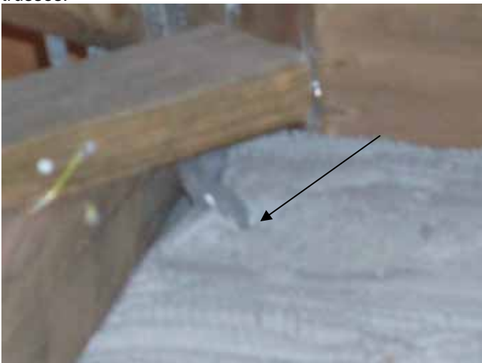
Many of the truss anchor straps were not correctly installed. The straps were offset too far from the trusses.
