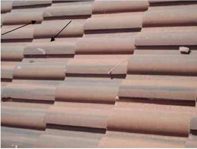
There were broken & incorrectly repaired tiles on the roof at multiple locations.
