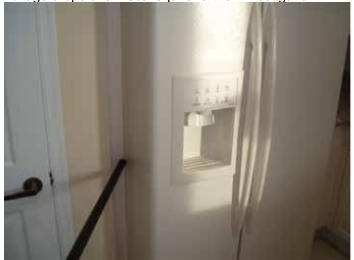
We were unable to view the area behind the refrigerator because it was wedged in & stuck between the trimmed opening.
