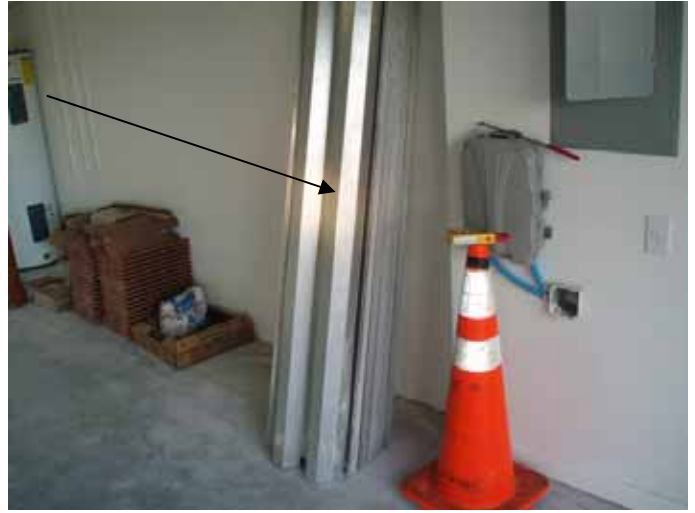
The storm shutter panels were not correctly secured in place. – Potential Hazard.
