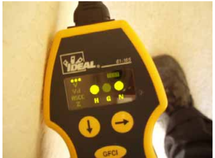
There were several receptacle outlets that tested loose or open ground in the master bedroom.
