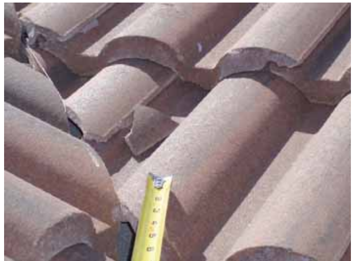
Loose & incorrectly installed roof tiles & construction debris can become windborne projectiles during a hurricane.
