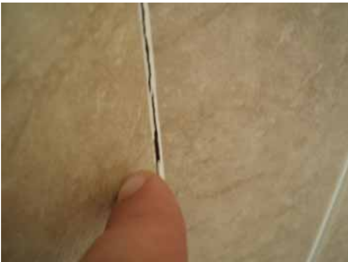
There were cracks & unsealed openings in the tile grout in the master bathroom.
