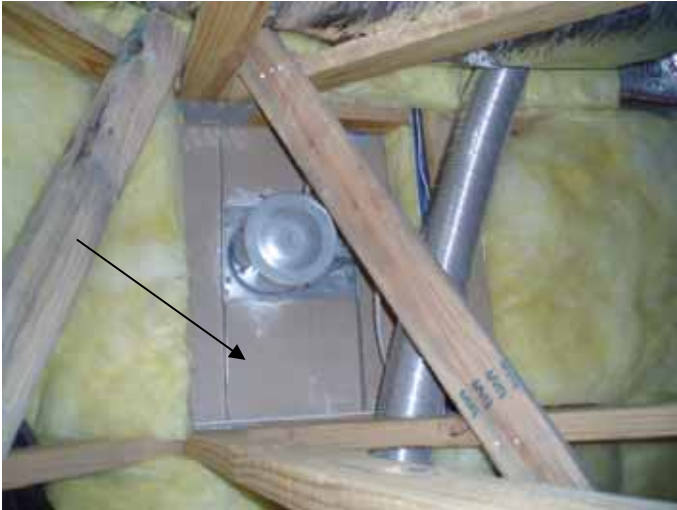
There were areas of the attic with displaced or missing insulation. All attic areas over conditioned space are required to be insulated.
