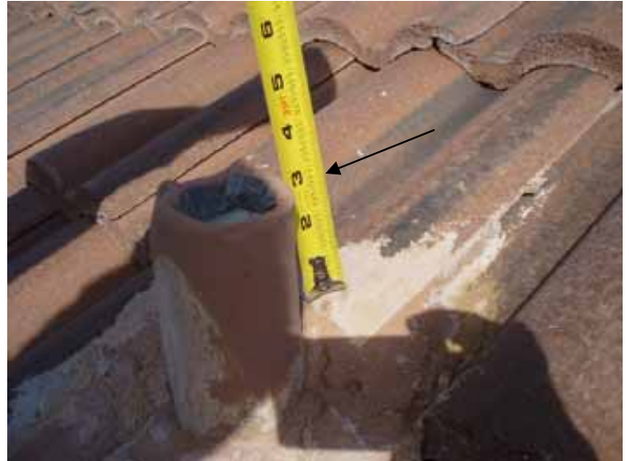
The plumbing vent stack was not the correct height. The vent stack should terminate at 6 inches minimum above the roof. §P904.1
