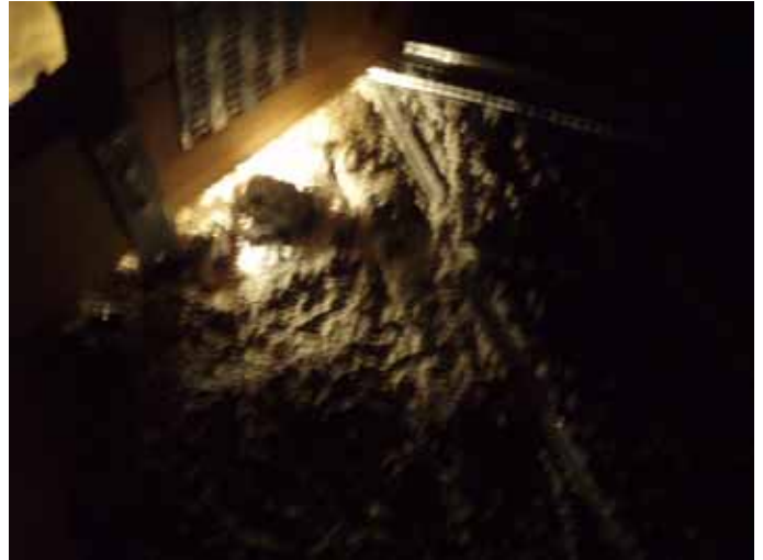
There were trusses that do not have 3 " bearing on a grout filled masonry cell or concrete at multiple locations. $2319.3
