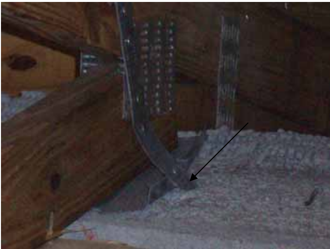
Many of the truss anchor straps were not correctly installed. The straps were offset 2" or more from the trusses.
