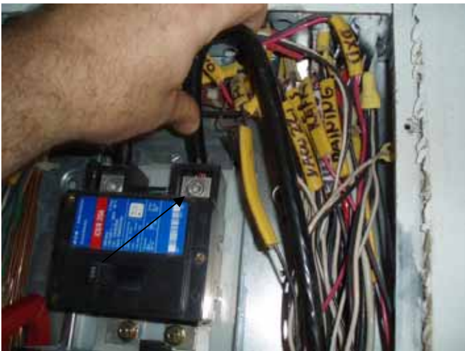
The terminal lug was loose & not correctly secured at the (HOT) ungrounded entrance conductor at the right side of the main distribution panel.
