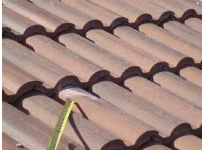
There were broken tiles that were incorrectly "glued" back together on the roof.
