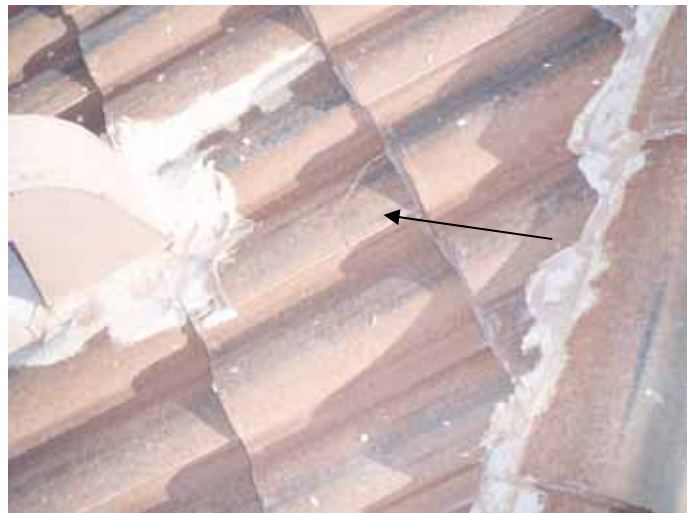
The broken roof tiles should be removed & replaced, not "glued" back together.
