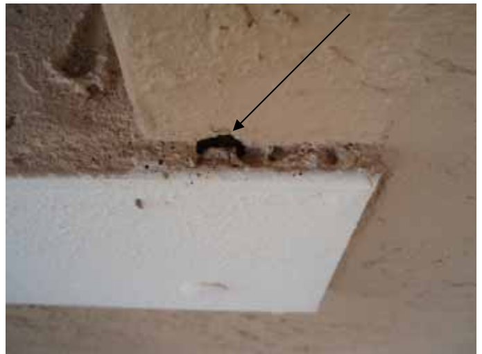
There were exposed areas with missing stucco at the window trim. These locations should be correctly sealed to prevent water & pest intrusion.
