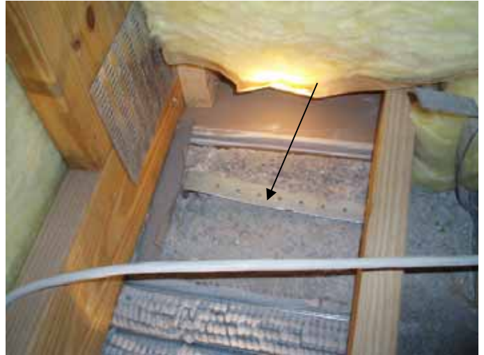
Many of the truss anchor straps were not correctly installed.
