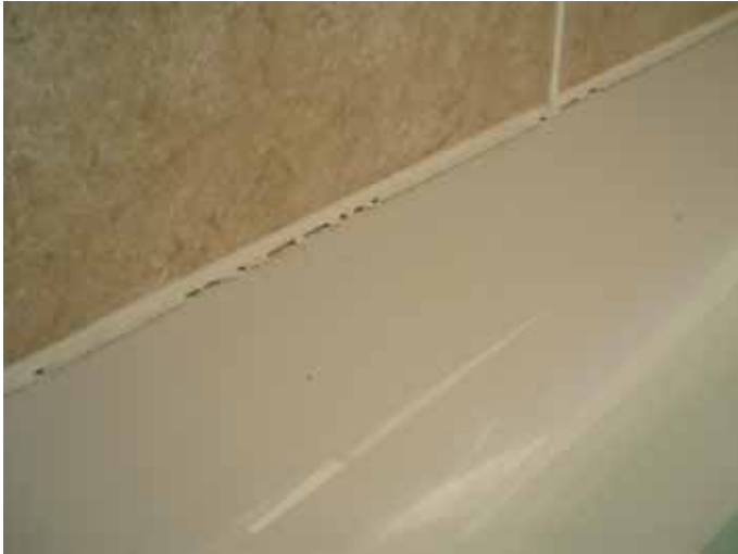
There were cracks & unsealed openings in the caulk around the tub in the master bathroom.
