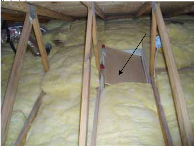
The back of the master attic access hatch cover was not insulated.
