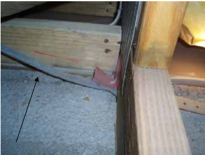
Many of the truss anchor straps were not correctly installed. The straps were not attached or nailed to the trusses.
