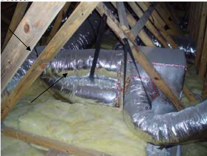
Some of the ducts were not correctly supported. Some of the support straps were twisted. We recommend the ducts be supported off other ducts & insulation.
