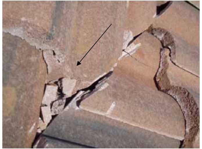
All construction debris should be removed from the roof.
