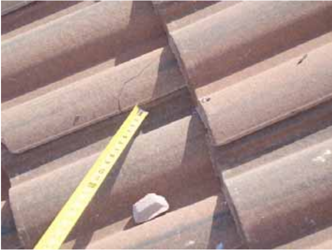
There were cracked & broken tiles on the roof at multiple locations.
