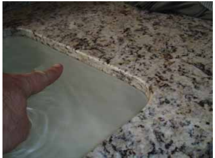
The sink was not correctly sealed at the counter top.
