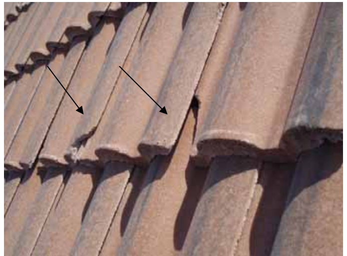
The broken roof tiles should be removed & replaced, not "glued" back together.
