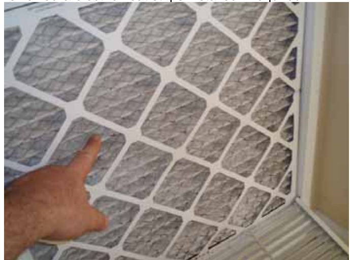
Note: the AC filters were installed backwards. There was rust &/or corrosion on the wire mesh on the filters.
