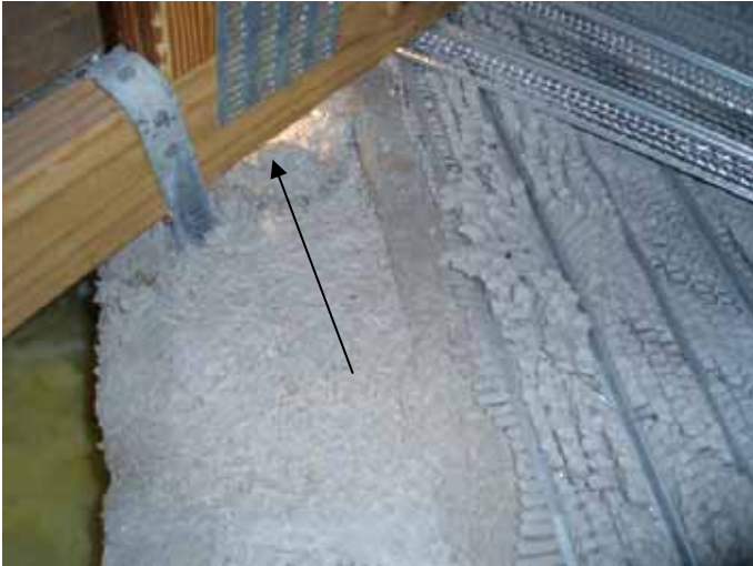
There were trusses bearing on the concrete beams with no protection between the truss & concrete.
