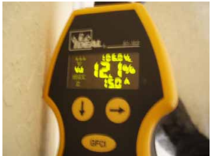
The voltage drop at some of the outlets exceeds 10%. 2002(NEC) 210.19 Conductors. We believe that any voltage drops over 10% require further investigation.
