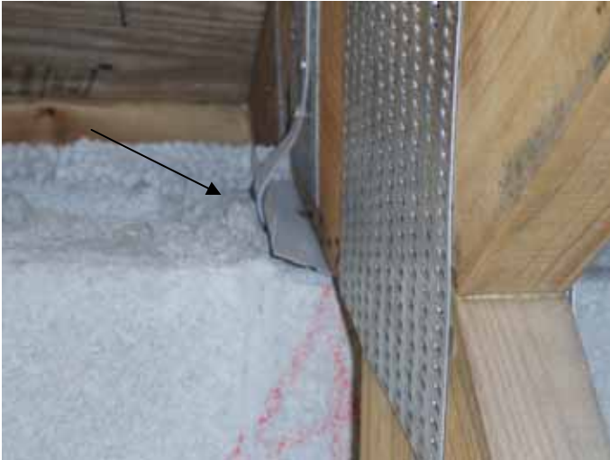
Many of the truss anchor straps were not correctly installed. The straps were offset 2" or more from the trusses.
