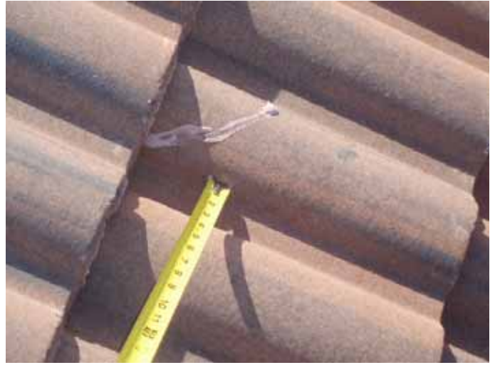
There were broken tiles that were incorrectly "glued" back together on the roof.
