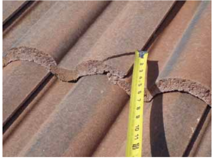
There were broken tiles that were incorrectly "glued" back together on the roof at multiple locations.
