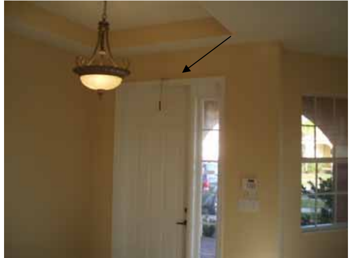
The top of the front door frame was not correctly sealed. §13-606.1.ABC.1.2.1
