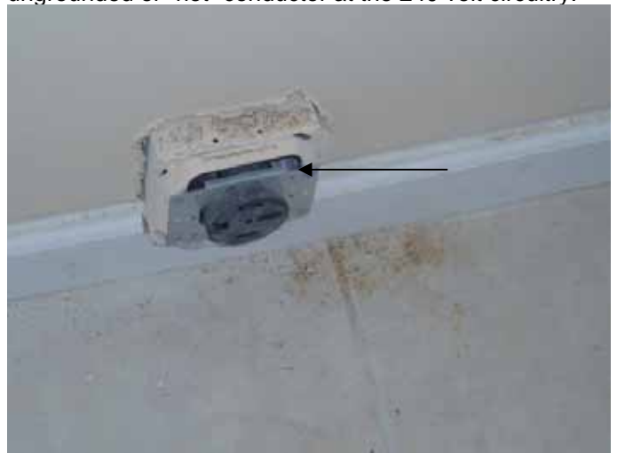
The junction box for the range receptacle outlet was not fully covered.
