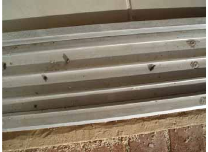
There was no gasket or seal installed to prevent pest intrusion at the right side sliding screen door at the back patio.
