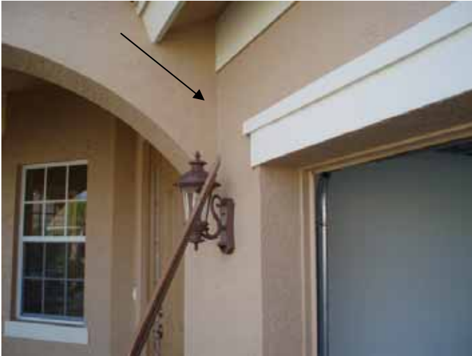
Location of the previous photo. All cracks & openings in the exterior should be sealed to prevent water & pest intrusion.
