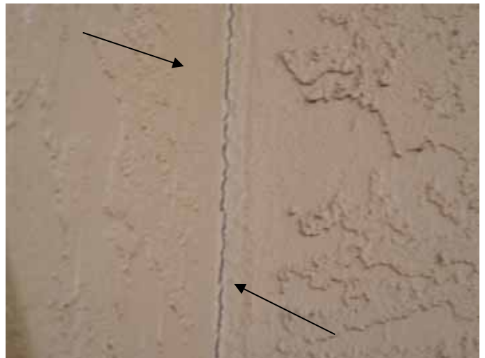
There were unsealed cracks & openings in some of the exterior stucco walls.
