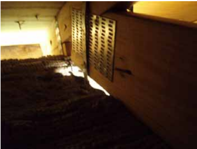
There were trusses that do not have 3 " bearing on a grout filled masonry cell or concrete at multiple locations. §2319.3
