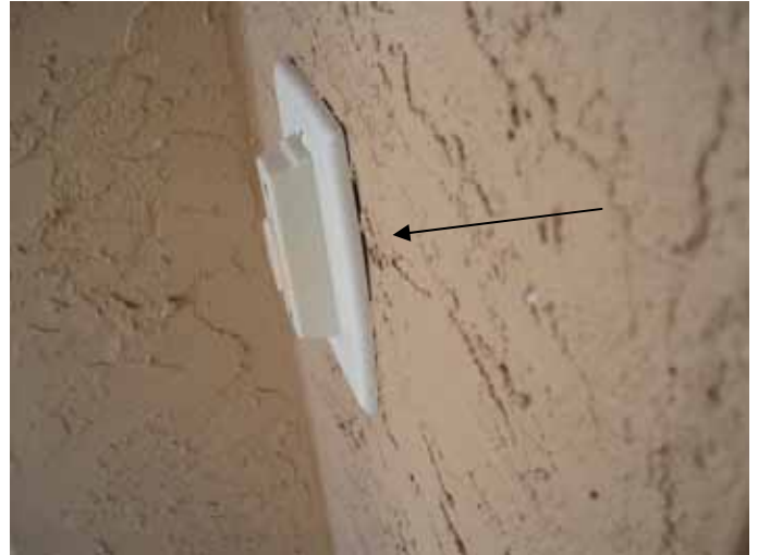
The doorbell cover was not correctly sealed as required. 2002 NEC 410.4, §13-606.1.ABC.1.2
