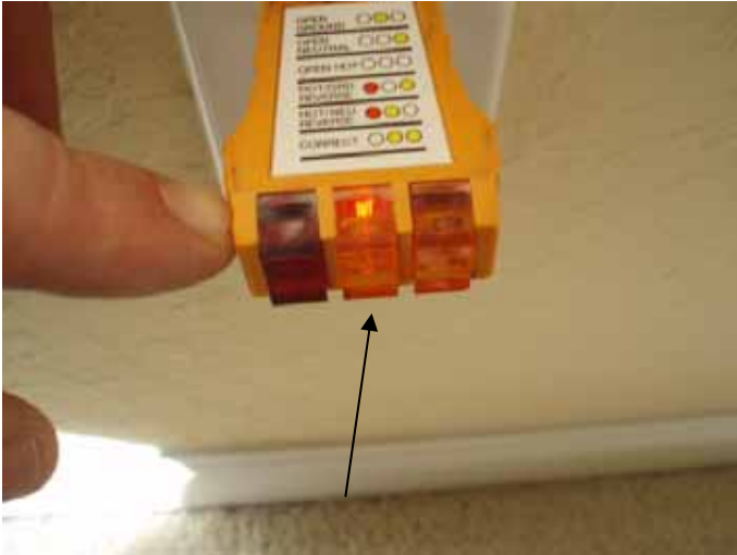
There were several receptacle outlets that tested loose or open ground in the master bedroom.
