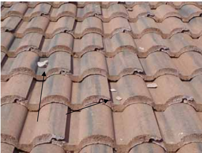
Loose & incorrectly installed roof tiles & construction debris can become windborne projectiles during a hurricane.
