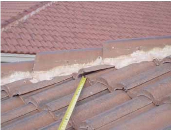
There were tiles that were not correctly set in place on the roof at multiple locations.
