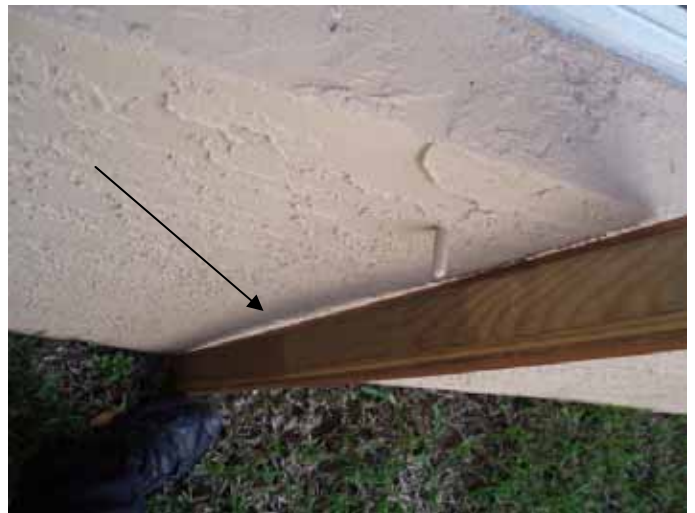
The stucco at some at the walls was concave or curved in & does not appear to be the correct thickness. §2509.1.1, ASTM C 926
