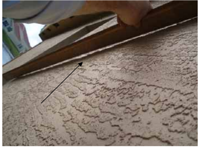
The stucco at some at the walls was concave or curved in & does not appear to be the correct thickness. §2509.1.1, ASTM C 926
