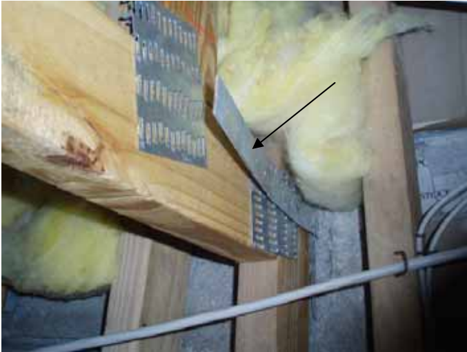
The straps were not attached or nailed to the trusses at multiple locations.
