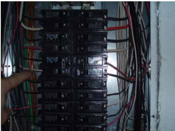
The white insulated wiring needs to be permanently marked or color coded to indicate it is being used as an ungrounded or "hot" conductor at the 240 volt circuitry.
