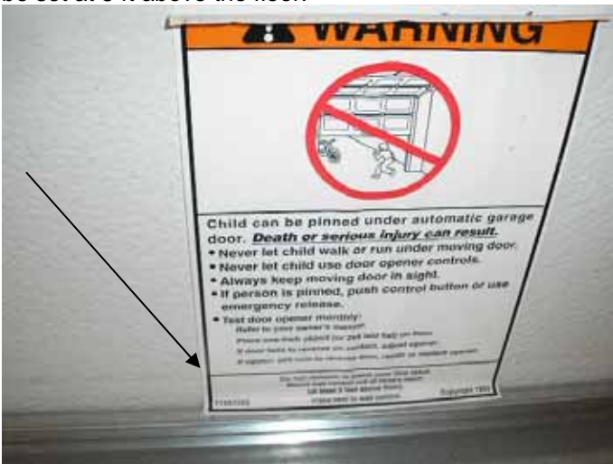
A warning label like this one needs to go on the wall by the auto door opener switches §M304.1
