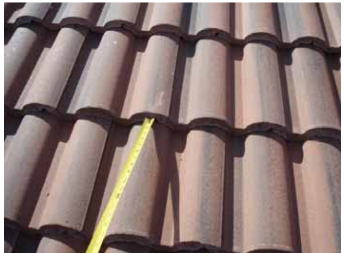
The broken roof tiles should be removed & replaced, not "glued" back together.
