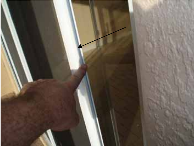
There was no gasket installed to prevent pest intrusion at the right side sliding screen door at the back patio.
