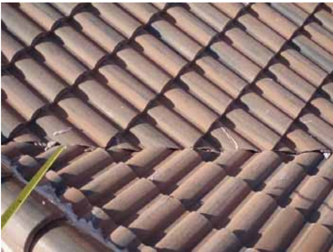
There were broken tiles that were incorrectly "glued" back together on the roof.
