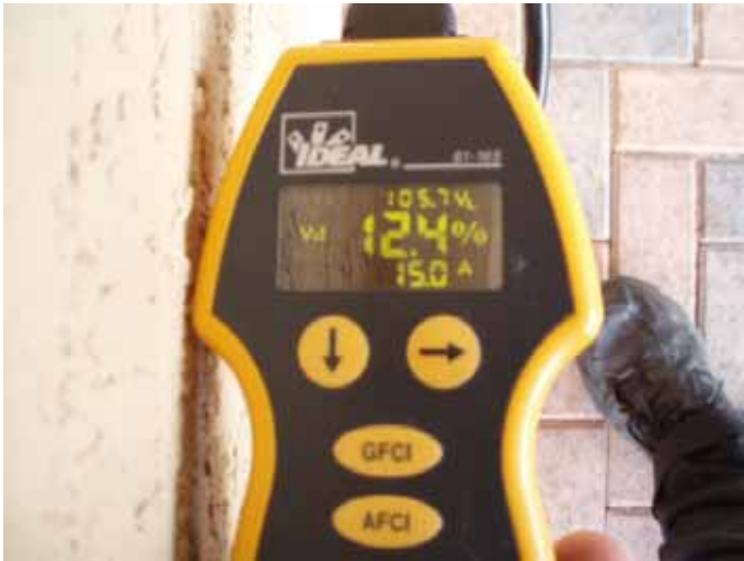
The voltage drop at some of the outlets exceeds 10%. 2002(NEC) 210.19 Conductors. Location at the back patio.
