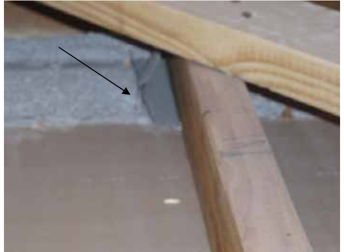
There should not be any slack in the truss anchor straps.
