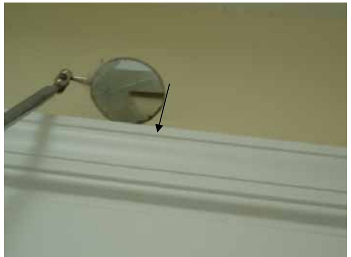
The top of the garage/laundry access door frame was not correctly sealed as required. §13-606.1.ABC.1.2.1
