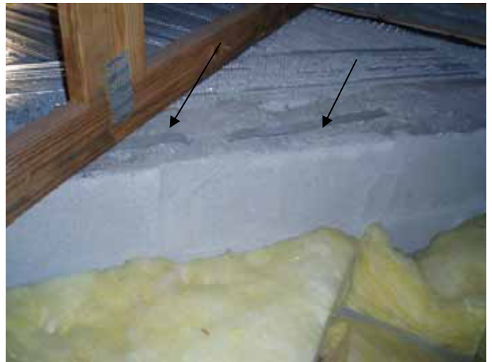
Some of the straps were not anchored to the trusses. There were trusses bearing on the concrete beams with no protection between the truss & concrete.
