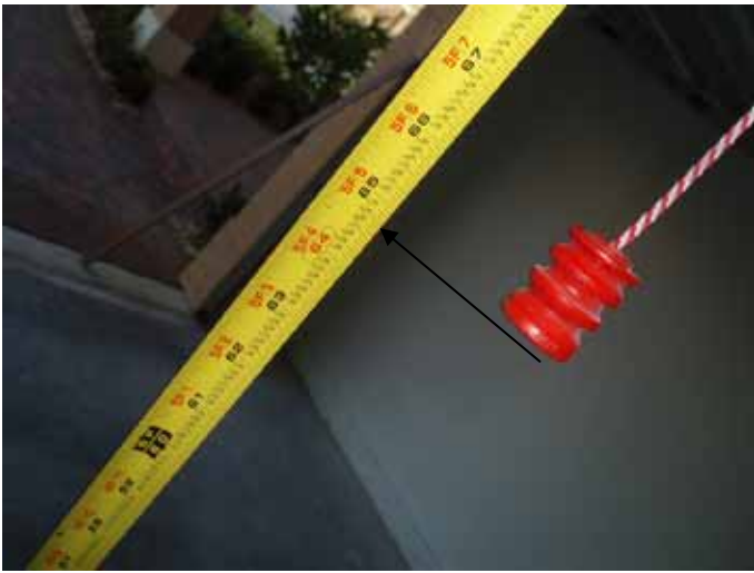
The red emergency release cord & handle were not set high enough above the garage floor. The handle should be set at 5 ft above the floor.
