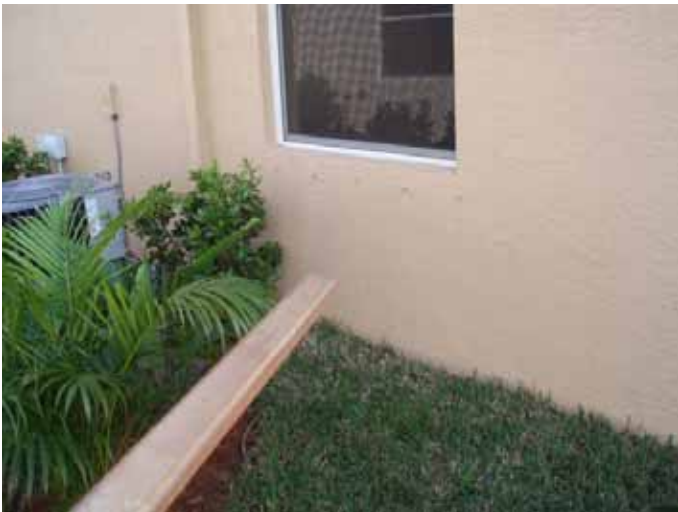
We recommend core sampling to verify the thickness of the exterior stucco & compliance with ASTM C 926 at the locations identified.
