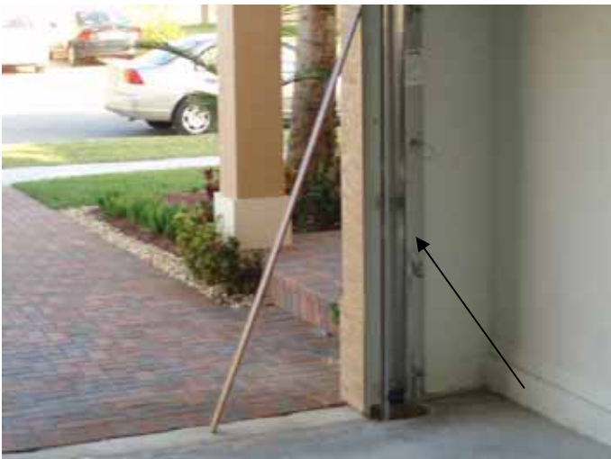
Location of the previous photos. All of the nuts & bolts for the 2"x6" garage door bucks should be correctly secured in place.
