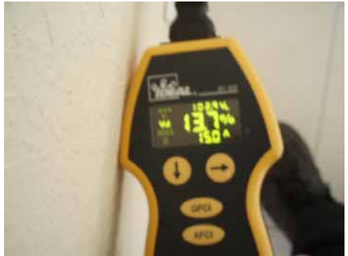
The voltage drop at some of the outlets exceeds 10%. 2002(NEC) 210.19 Conductors. We believe that any voltage drops over 10% require further investigation.
