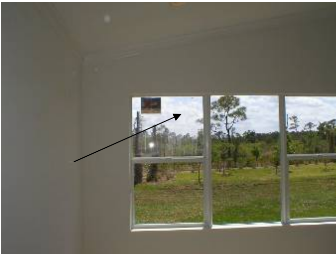
The glass is cracked at the top left window in the master bedroom.
