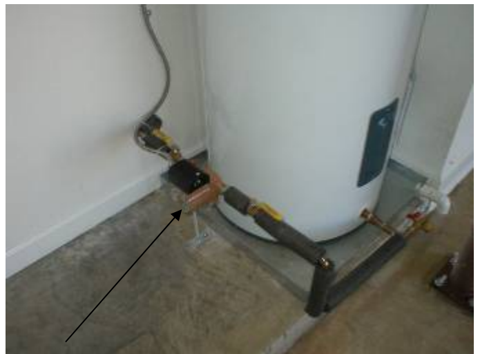
The hot water circulating pump did not operate at the time of the inspection.
