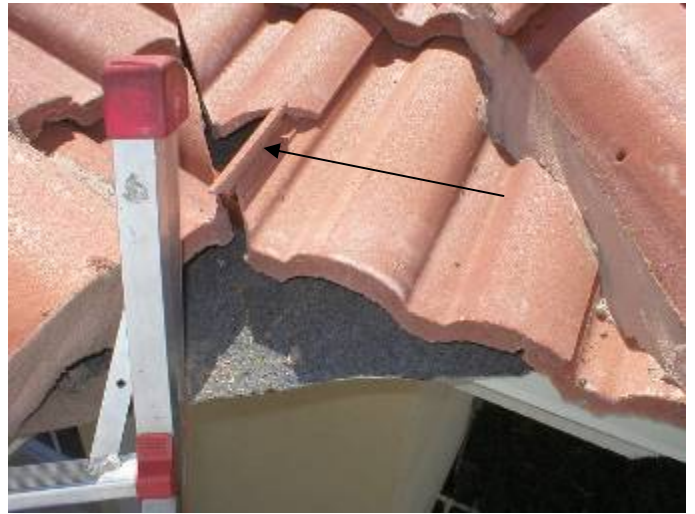
There are several broken pieces of tile & construction debris on the roof.
