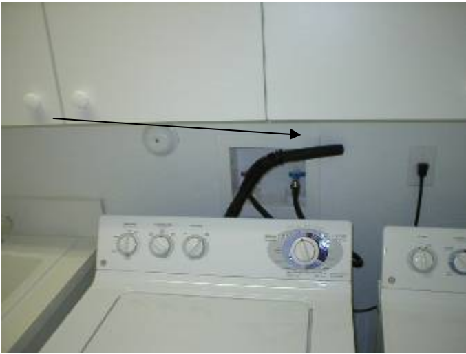
The washer drain hose has not been secured or set in place.
