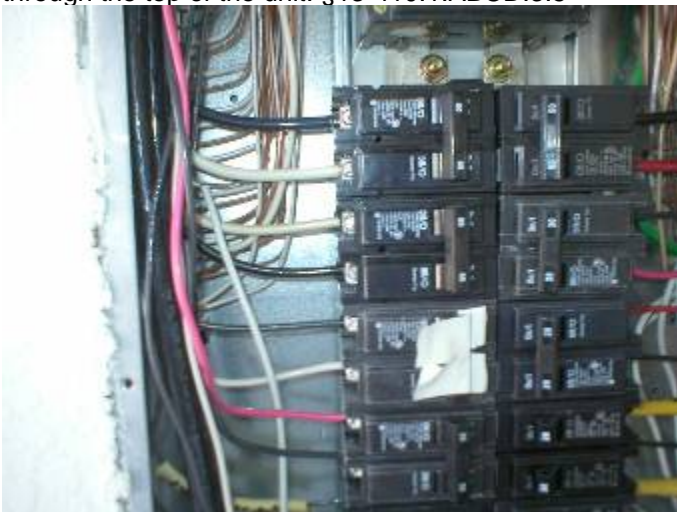
The white wires are not correctly color coded to identify them as being used as "hot" in the main panel & at the AC disconnects.
