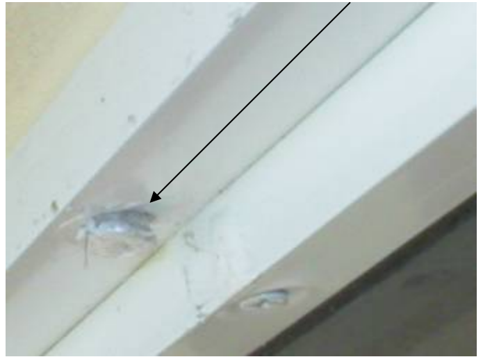
Some of the screw anchors are not correctly set or sealed to prevent water & pest intrusion around the window & door frames. §13-606.1.ABC.1.2
