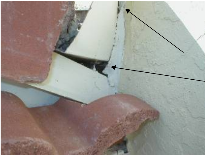
The wall is not correctly sealed at the flashing to prevent water & pest intrusion at the corner above the front of the garage. §1403.1.3
