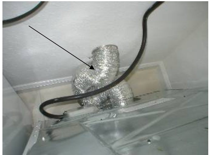
The foil dryer vent duct material is a fire hazard per UL & manufacturer. Replace with rigid or heavy flex duct material in accordance with manufacturer's instructions.
