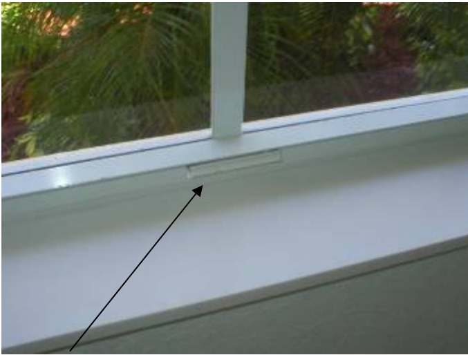
The window lock on the left window is installed at the bottom & the lock on the right side window is installed at the top.
