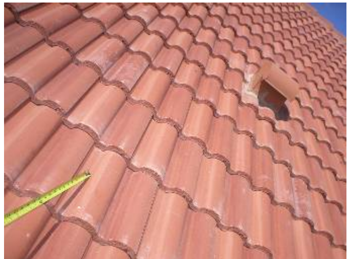
There should be no more than 13 – 13 & 1/2 inches of exposed roof tile to allow for the correct headlap.
