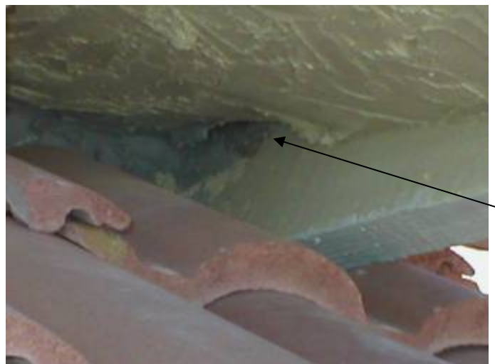
The stucco is not correctly sealed at the soffit return area to prevent water & pest intrusion above the right front side of the house. §2509.2.4.1
