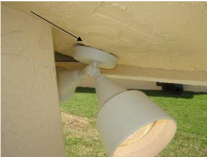
The stucco is not correctly sealed around the lighting fixture to prevent water & pest intrusion at the soffit at the SE corner of the house. §13-606.1.ABC.1.2
