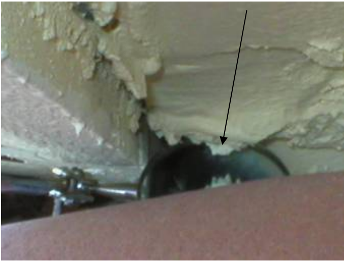
The stucco is not correctly sealed at the soffit return area to prevent water & pest intrusion at the corner above the front of the garage. §13-606.1.ABC.1.2
