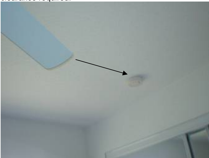
The smoke detectors are installed too close to the ceiling fan blade tips in the guest bedrooms. 3 ft horizontal clearance required.
