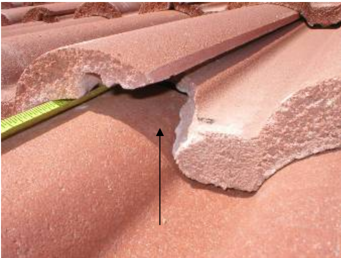
The tile is broken at the corner.
