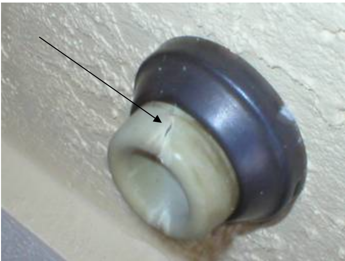
The door stop is damaged at the front entry way.
