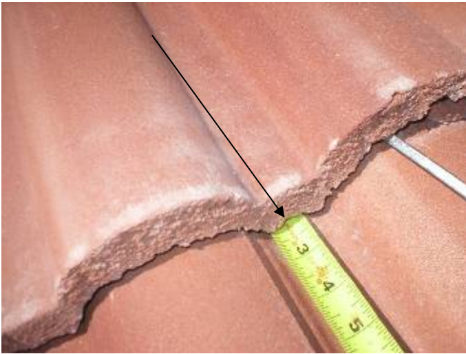
The roof tile headlaps (overlap) are incorrect at some locations. 3 inch minimum headlap should be used for wind storm uplift. 2 inch headlaps are incorrect. §1518.8.11
