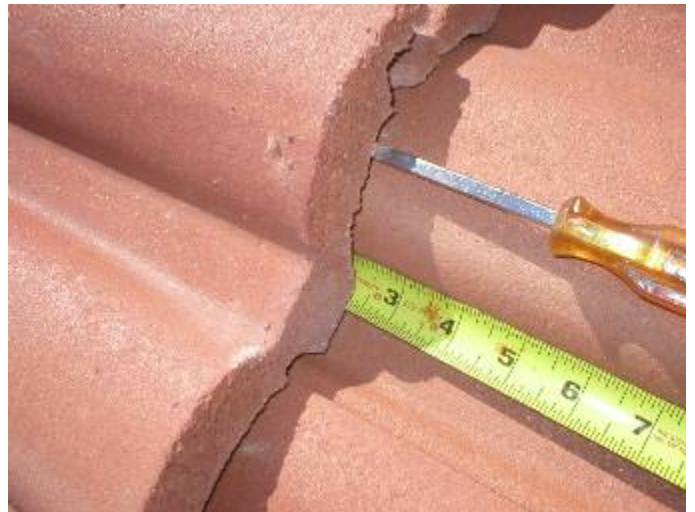
The roof tile headlaps (overlap) are incorrect at some locations. 3 inch minimum headlap should be used for wind storm uplift. 2 inch headlaps are incorrect. §1518.8.11
