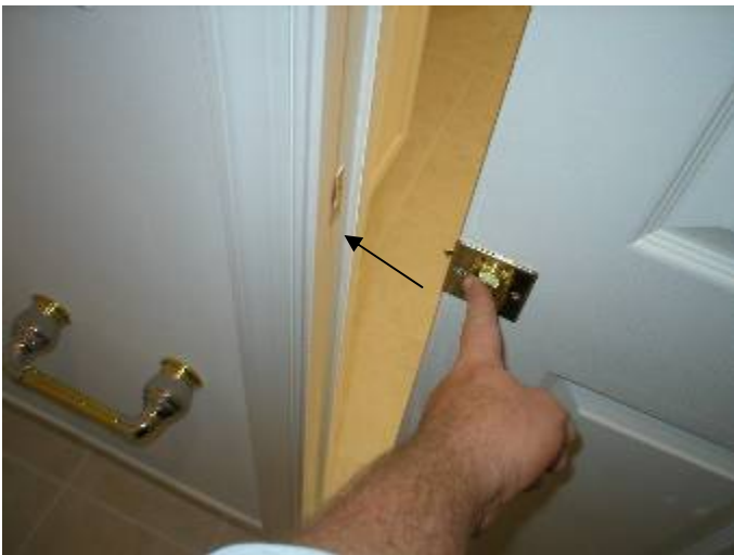
The latch did not engage correctly at the master bathroom pocket door.
