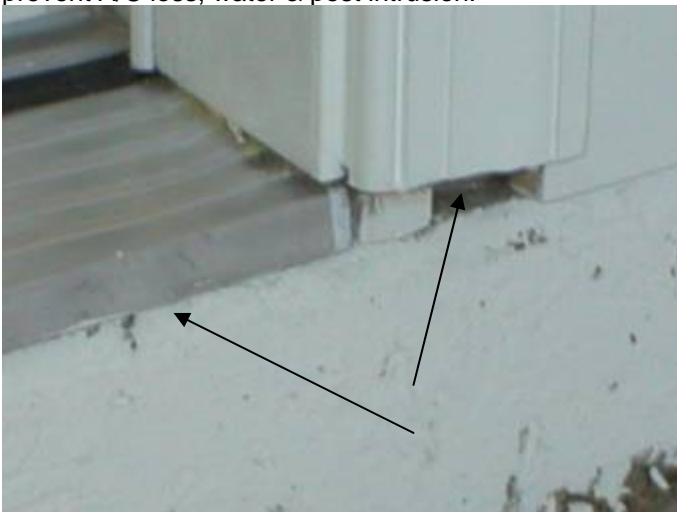
The door frame & threshold are not correctly sealed to prevent water & pest intrusion at the garage/laundry access door.
