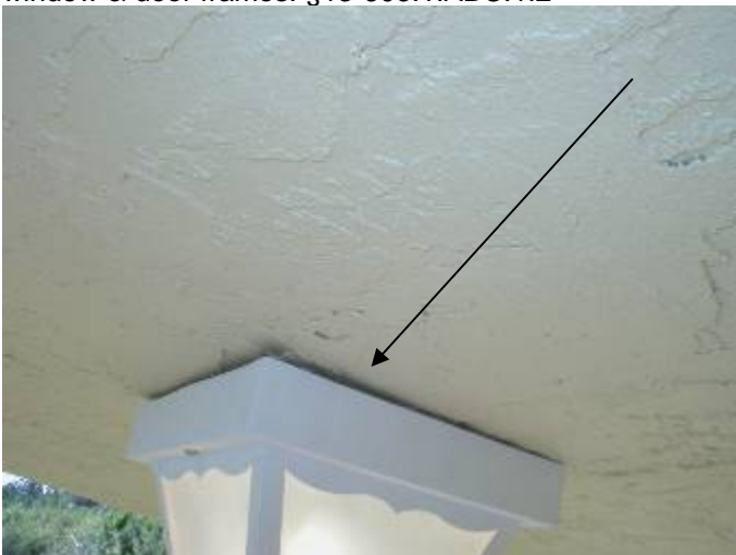
The stucco is not correctly sealed to prevent water & pest intrusion around the lighting fixture at the lighting fixture at the rear patio. §13-606.1.ABC.1.2
