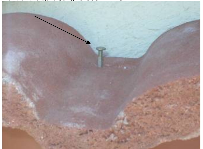
There are loose, incorrectly secured roof tiles at the front over the garage.
