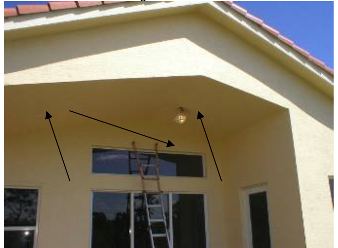
Location of the previous photos at the rear patio. The stucco is not a minimum of 1/2 inches at this location. §2509.2.4.1
