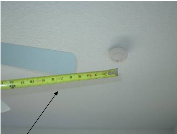
The smoke detectors are installed too close to the ceiling fan blade tips in the guest bedrooms. 3 ft horizontal clearance required.
