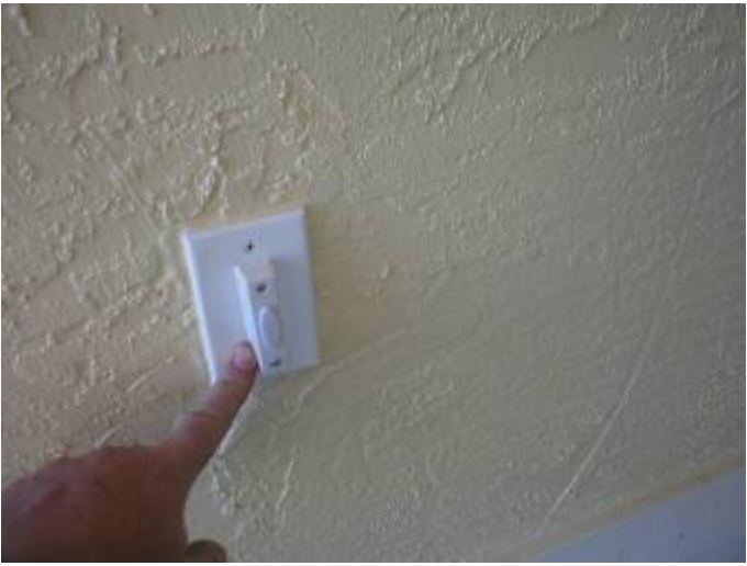
The door bell did not work.
