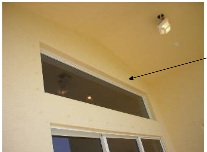
Some of the screw anchors are not correctly set or sealed to prevent water & pest intrusion around the window & door frames. §13-606.1.ABC.1.2
