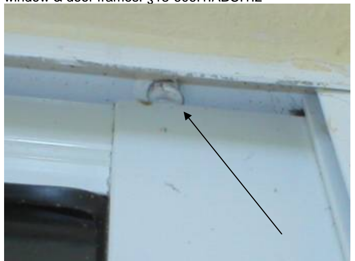
Some of the screw anchors are not correctly set or sealed to prevent water & pest intrusion around the window & door frames. §13-606.1.ABC.1.2
