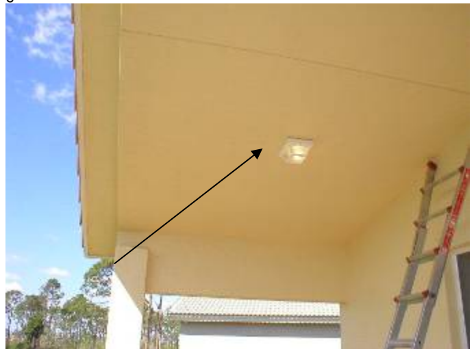
Location of the previous photo at the rear patio. The stucco is not a minimum of 1/2 inches at this location. §2509.2.4.1
