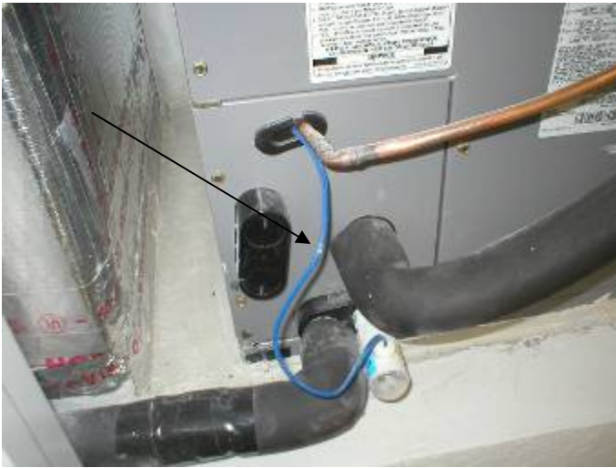
The low voltage wiring should not run through the same opening as the refrigerant line in the air handler.
