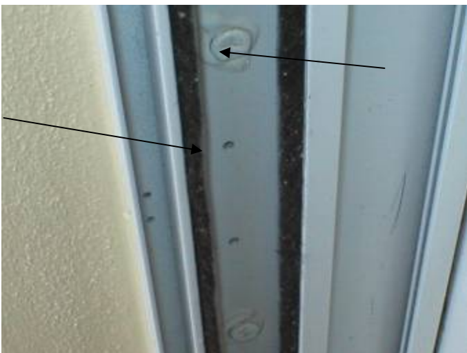
Some of the screw anchors are not correctly set or sealed to prevent water & pest intrusion around the window & door frames. §13-606.1.ABC.1.2
