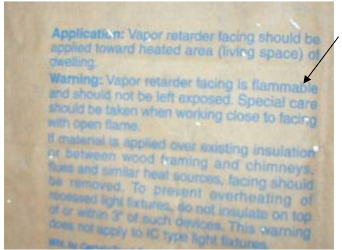
There is exposed kraft paper insulation backing in the attic. The manufacturer states the facing is flammable & should not be exposed. §M304.1
