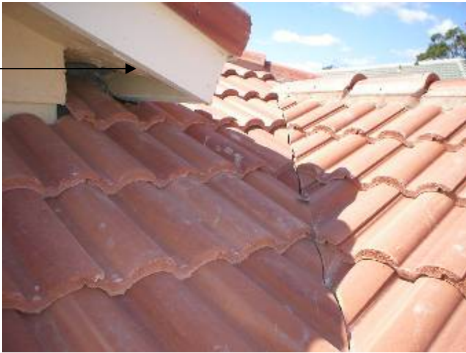
The stucco is not correctly sealed at the soffit return area to prevent water & pest intrusion above the right front side of the house.
