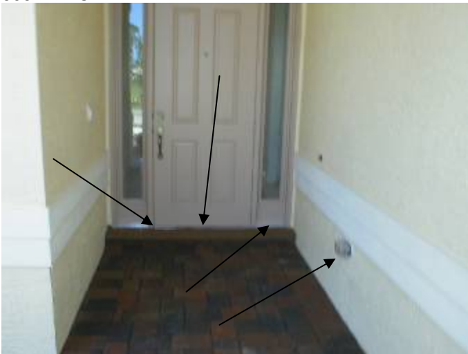
Location of the previous photos taken at the front entry way. The doors & frames should be correctly sealed to prevent A/C loss, water & pest intrusion.
