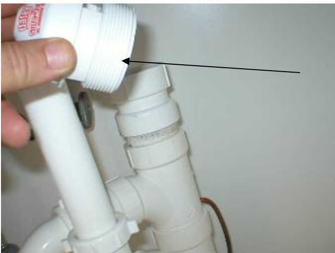
The manufacturer requires teflon tape at the threaded connection of the air admittance valves. §M304.1
