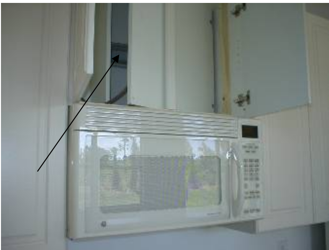
The microwave vent ductwork is not correctly connected.
