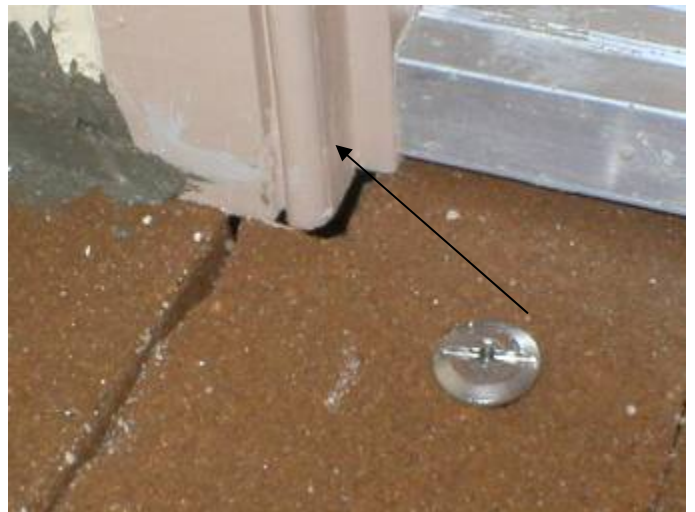
The door frame & threshold are not correctly sealed to prevent water & pest intrusion at the front entry way. §13-606.1.ABC.1.2
