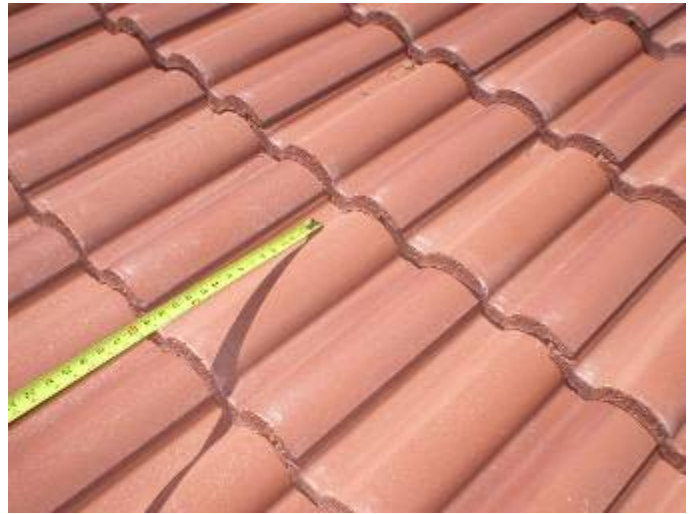
The roof tile headlaps (overlap) are incorrect at some locations. 3 inch minimum headlap should be used for wind storm uplift. 2 inch headlaps are incorrect. §1518.8.11
