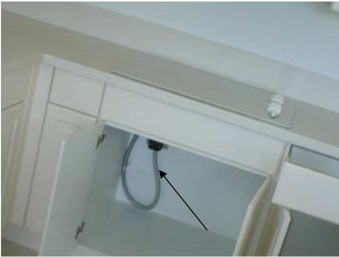
Install in accordance with manufacturer's instructions. Location in the kitchen.
