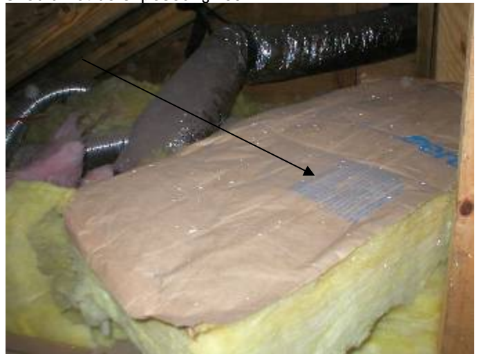
There is exposed kraft paper insulation backing in the attic. The manufacturer states the facing is flammable & should not be exposed.
