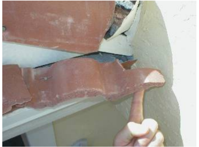
There are loose, incorrectly secured roof tiles at the front over the garage.
