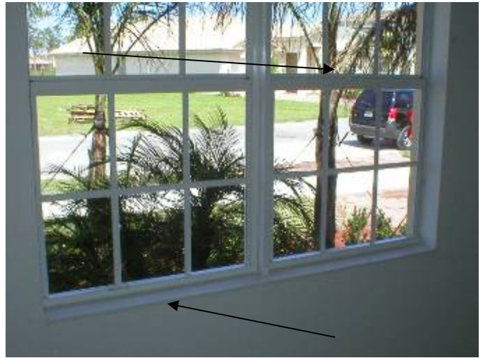
The window lock on the left window is installed at the bottom & the lock on the right side window is installed at the top at the front guest bedroom.
