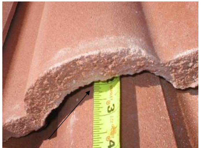
The roof tile headlaps (overlap) are incorrect at some locations. 3 inch minimum headlap should be used for wind storm uplift. 2 inch headlaps are incorrect. §1518.8.11
