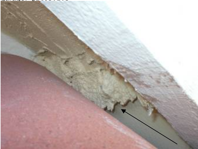
The stucco is not correctly sealed at the soffit return area to prevent water & pest intrusion at the corner above the front of the garage. §13-606.1.ABC.1.2
