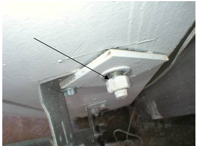
Some of the garage door wood buck anchor nuts are loose.
