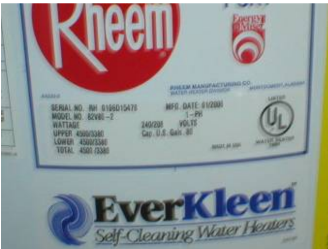
Note: Water heater information; 80 gallon electric water heater.
