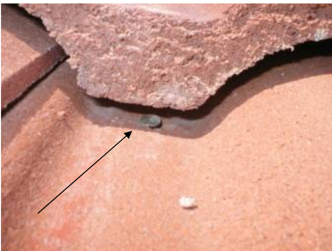
Some of the nail fasteners are visible indicating incorrect installation.
