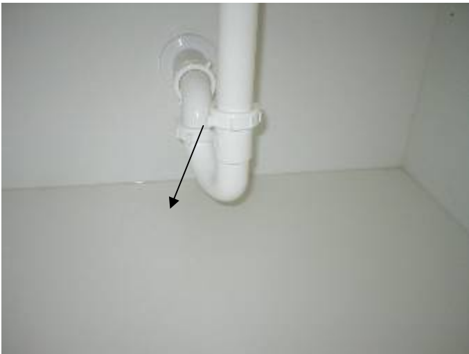
There are leaks at the plumbing drain line under the laundry room mud sink.
