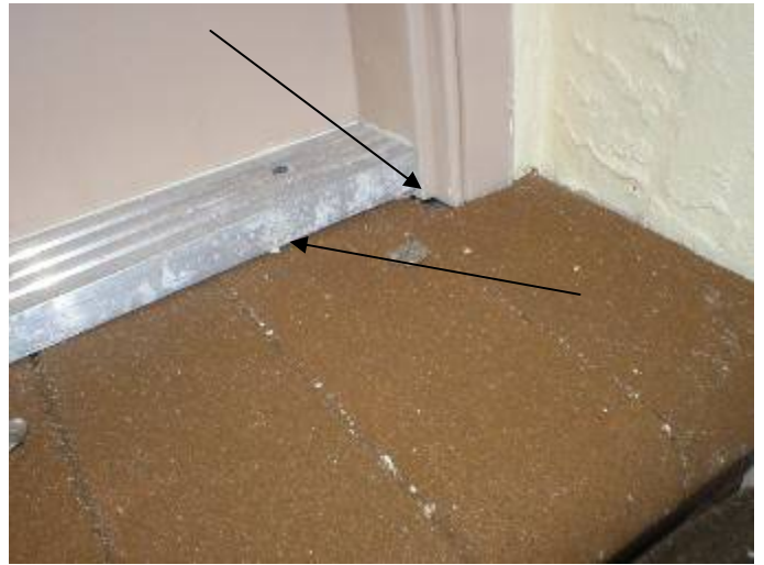
The door frame & threshold are not correctly sealed to prevent water & pest intrusion at the front entry way. §13-606.1.ABC.1.2
