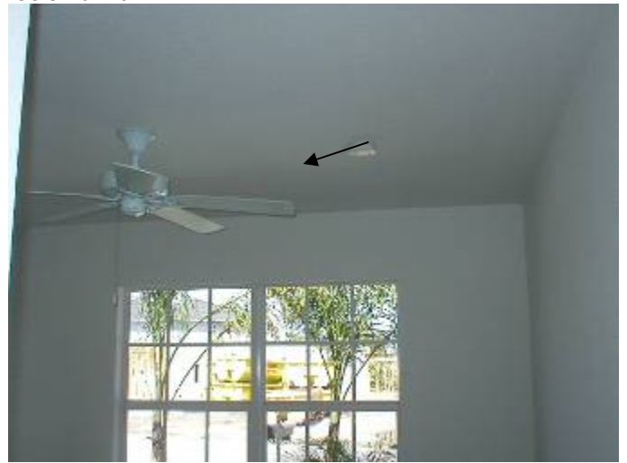
The smoke detectors are installed too close to the ceiling fan blade tips in the guest bedrooms. 3 ft horizontal clearance required.
