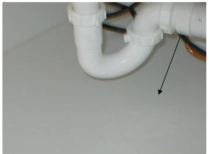
There are leaks at the plumbing drain line under the kitchen sink.
