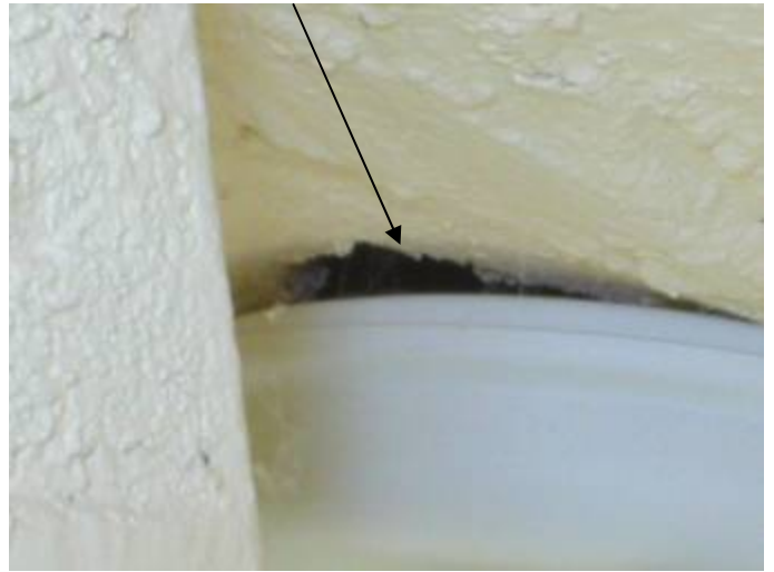
The stucco is not correctly sealed to prevent water & pest intrusion around the lighting fixture at the soffit at the SE corner of the house. §13-606.1.ABC.1.2
