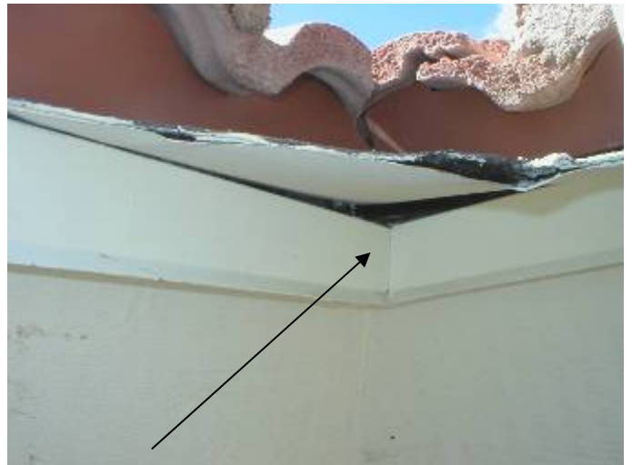
The underside of the valley end flashing is not correctly sealed to prevent water intrusion from wind driven rain.
