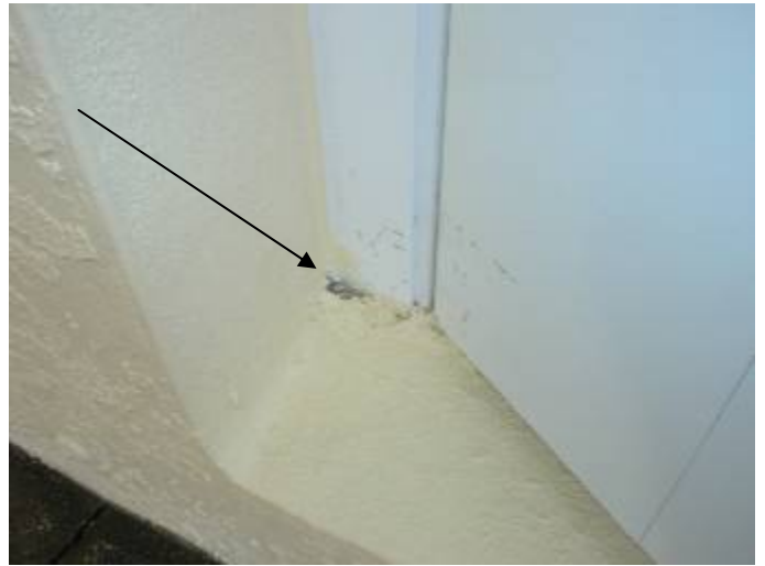
The door frame is not correctly sealed to prevent water & pest intrusion at the back patio. §13-606.1.ABC.1.2
