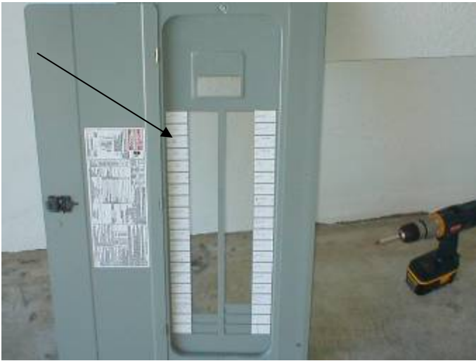
The circuit directory is not completely filled out to identify the breakers to the home owner.
