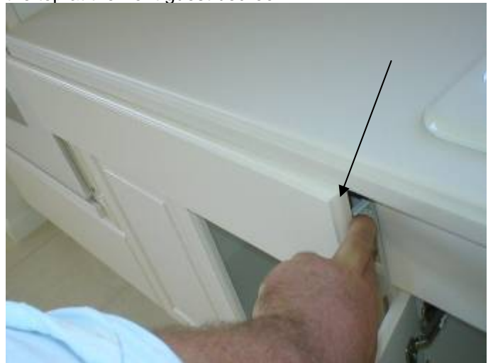
The drawer did not open correctly at the left of the kitchen sink.
