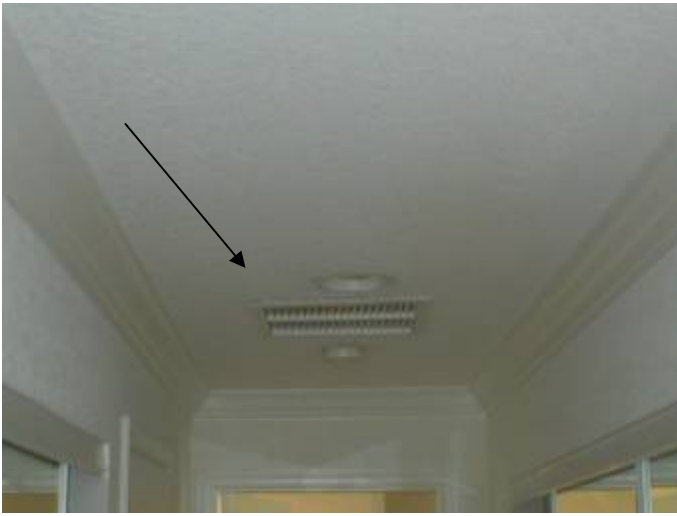
The return air grill is not correctly secured or sealed at the master bedroom hallway ceiling.
