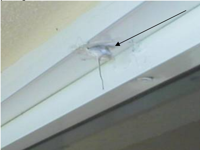
Some of the screw anchors are not correctly set or sealed to prevent water & pest intrusion around the window & door frames. §13-606.1.ABC.1.2
