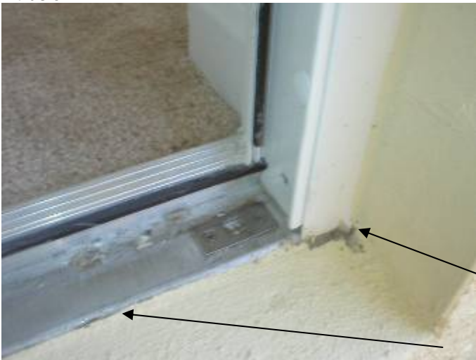
The threshold is not correctly sealed to prevent water & pest intrusion at the back patio. §13-606.1.ABC.1.2
