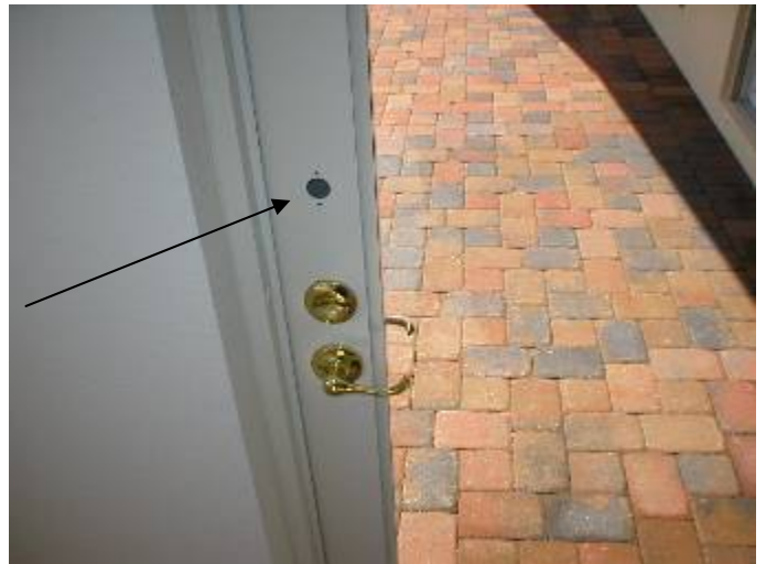
The top lockset is not installed at the master bedroom patio access door.
