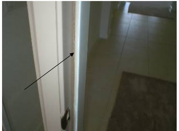
The weather seal has not been installed at the front door frame.
