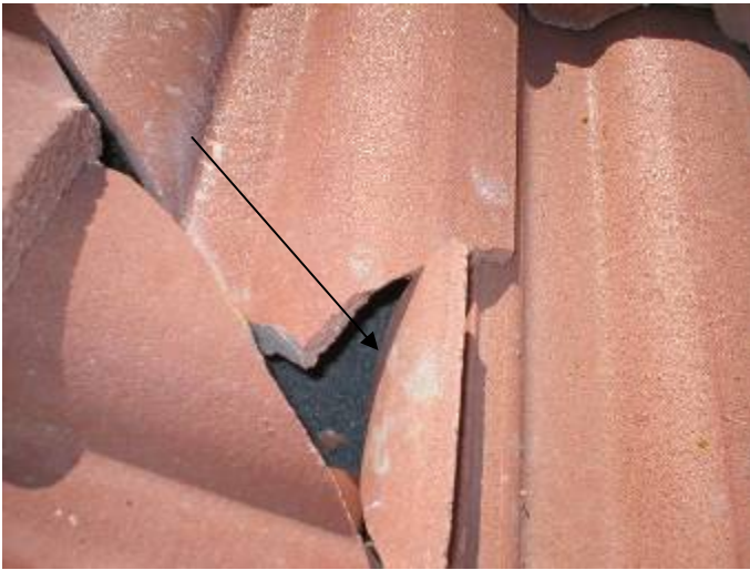
There are several broken pieces of tile on the roof.
