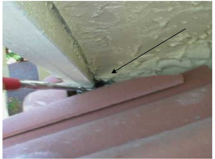
The stucco is not correctly sealed at the soffit return area to prevent water & pest intrusion at the corner above the front of the garage. §13-606.1.ABC.1.2
