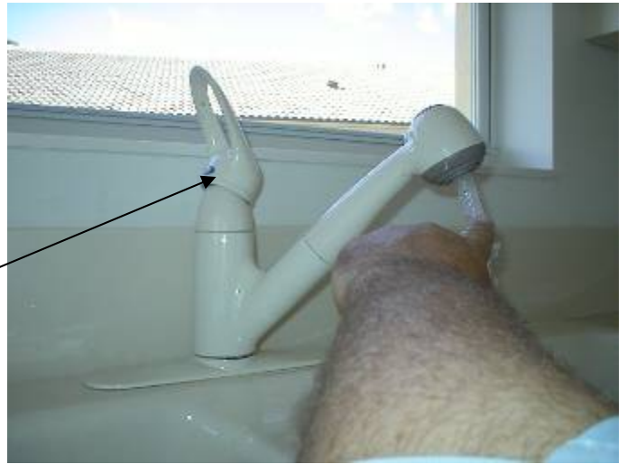
The hot water did not operate correctly at the kitchen sink faucet.
