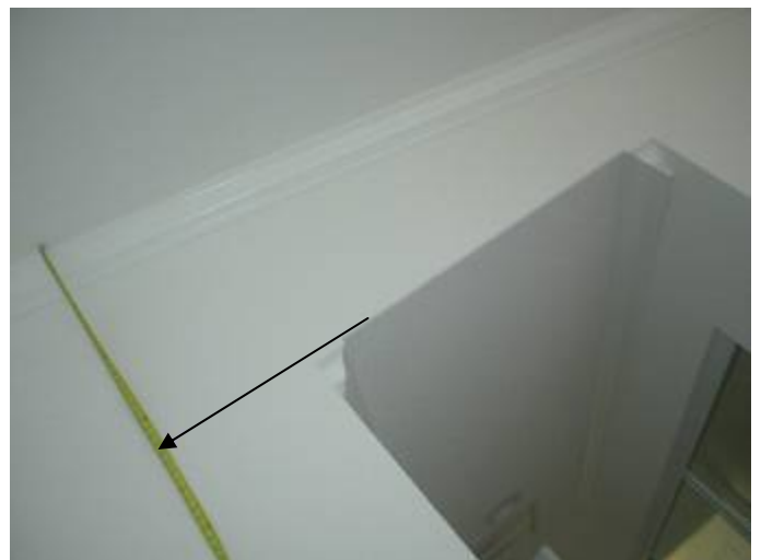
There is no access to the attic space above the master, guest bedrooms & dining area. Access is required when there is more than 24 inches of clear height. §2309.6
