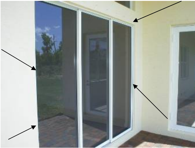
Location of previous photos. The doors & frames should be correctly sealed to prevent A/C loss, water & pest intrusion.
