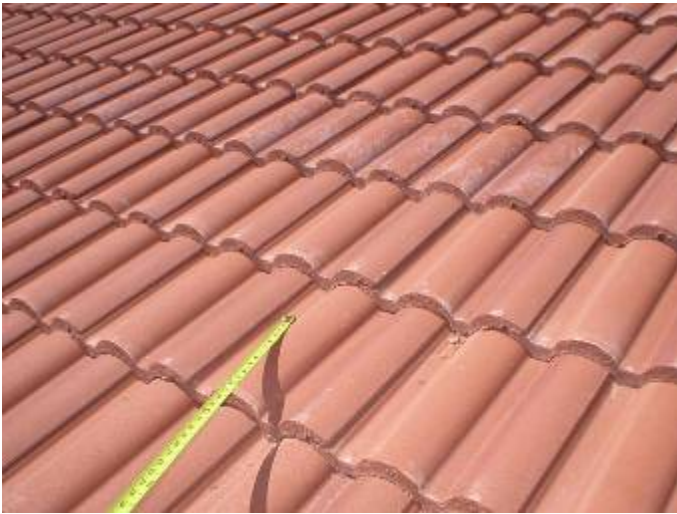
There should be no more than 13 – 13 & 1/2 inches of exposed roof tile to allow for the correct headlap.
