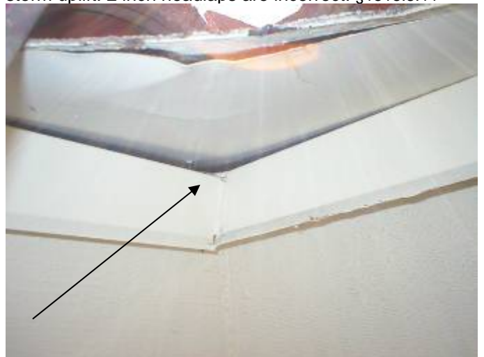
The underside of the valley end flashing is not correctly sealed to prevent water intrusion from wind driven rain.
