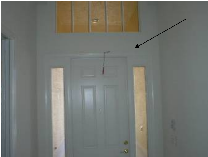
The trim at the top of the frames is not correctly sealed to prevent AC loss at the exterior doors.
