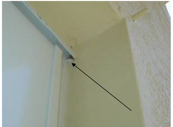
The door frame is not correctly sealed to prevent water & pest intrusion at the back patio. §13-606.1.ABC.1.2
