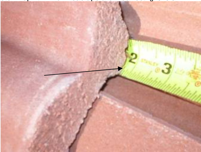
The roof tile headlaps (overlap) are incorrect at some locations. 3 inch minimum headlap should be used for wind storm uplift. 2 inch headlaps are incorrect. §1518.8.11
