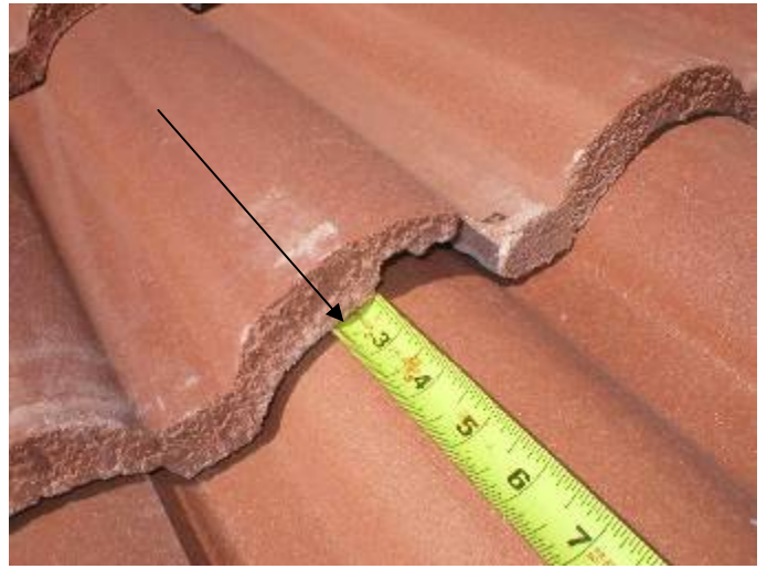
The roof tile headlaps (overlap) are incorrect at some locations. 3 inch minimum headlap should be used for wind storm uplift. 2 inch headlaps are incorrect. §1518.8.11
