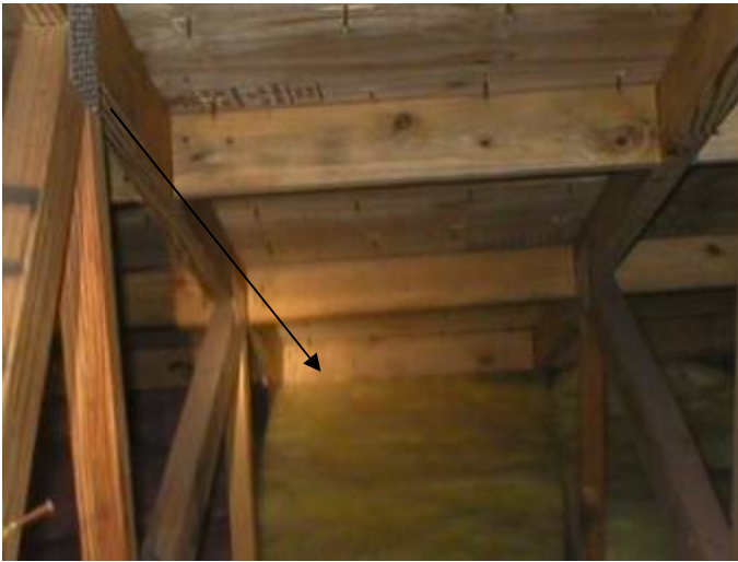
Attic insulation obstructs soffit ventilation at many locations around the perimeter of the attic. §2326.3.2
