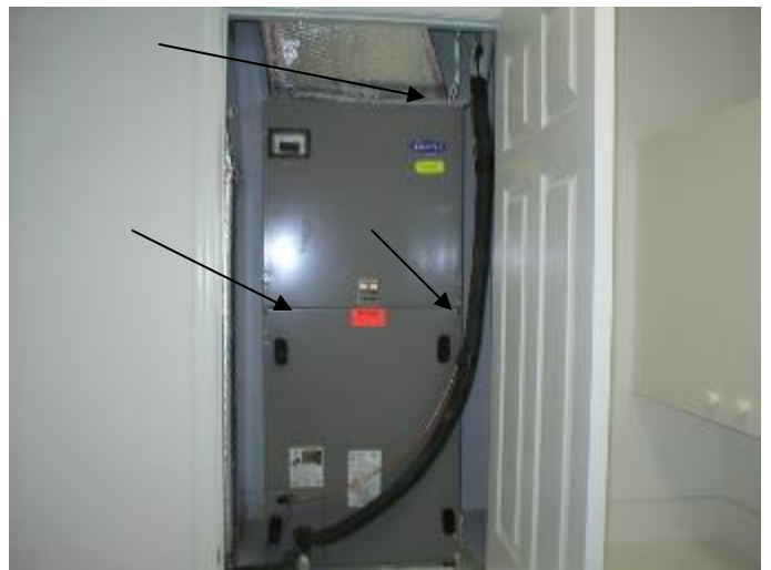
The AC air handler is not completely sealed. The AC air handler is too large for this closet space. §13-410.1.ABCD.3.7
