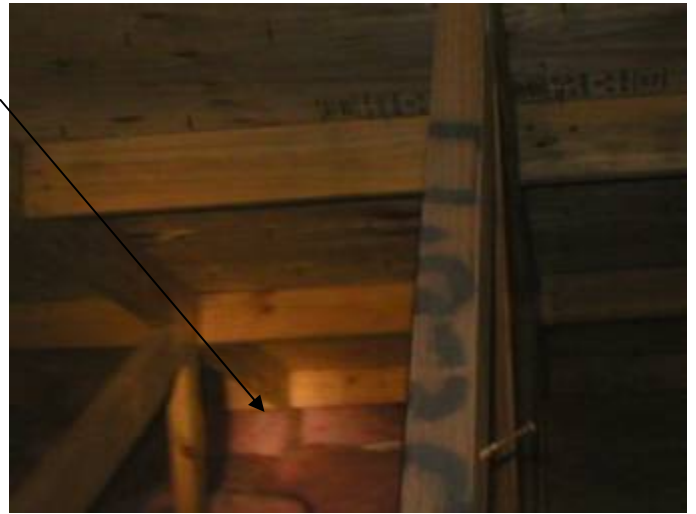
Insulation baffles should be installed to prevent blocked air flow.
