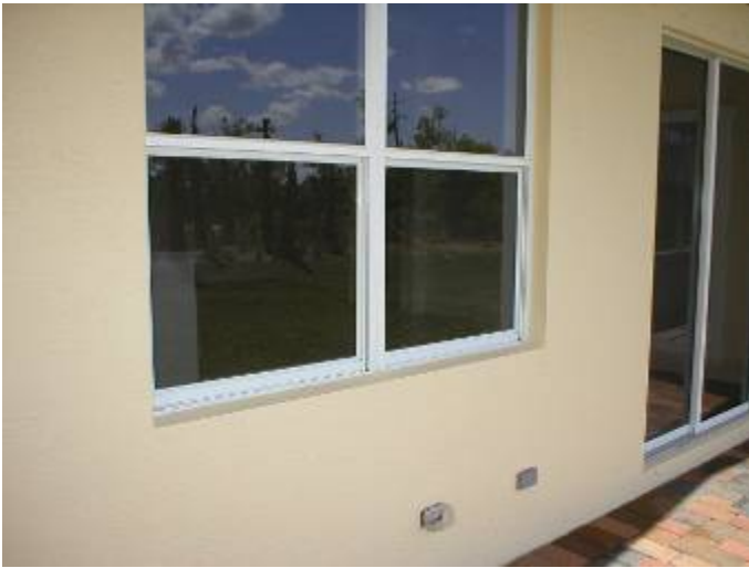
The screens have not been installed at the windows or sliding glass doors.
