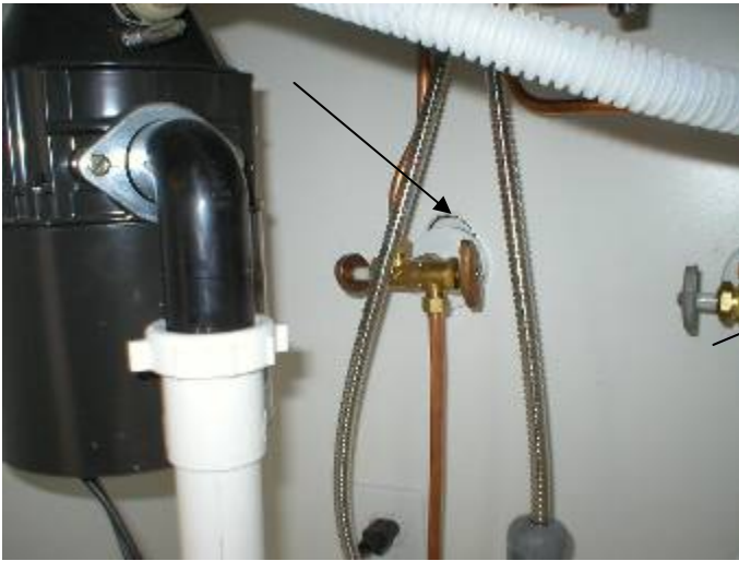
There are gaps & unprofessional looking cut outs at the back of the sink cabinets.
