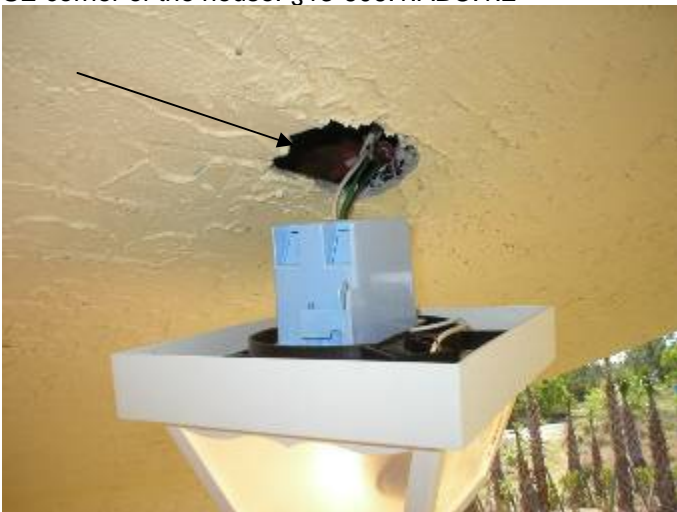
The light fixture junction box is not correctly installed or secured above the rear patio.
