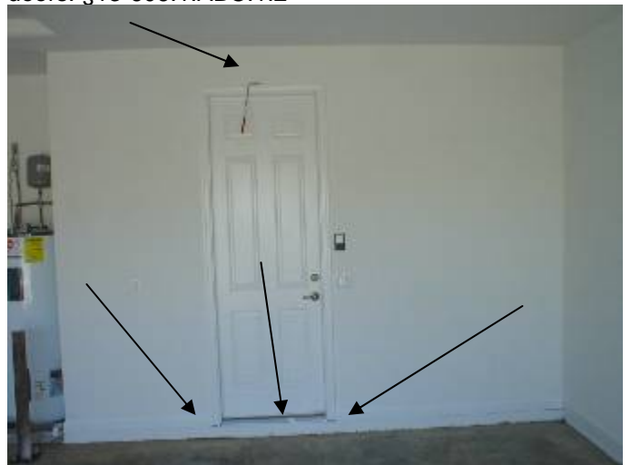
Location of previous photos. The doors & frames should be correctly sealed to prevent A/C loss, water & pest intrusion. §13-606.1.ABC.1.2
