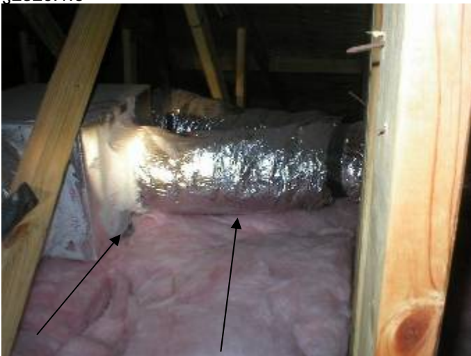
The AC ductwork & distribution boxes are not correctly supported of the insulation to prevent condensation & mold problems. §M603.11
