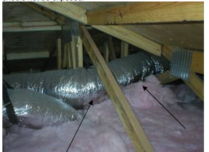
The AC ductwork & distribution boxes are not correctly supported of the insulation to prevent condensation & mold problems. §M603.11
