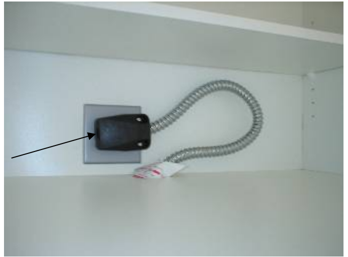
A plug & receptacle is not permitted for the oven electric supply. §M304.1
