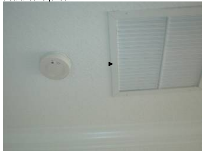
The smoke detector is installed too close to the AC return register.
