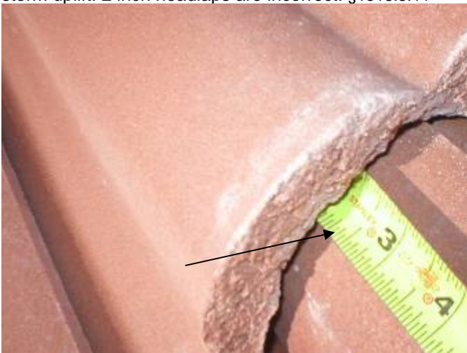
The overlap of some of the tiles is less than 2 inches.
