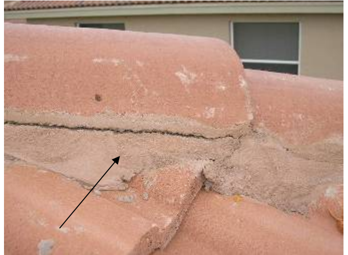
Some of the hip & ridge cap tiles are not correctly secured or bonded. §1518.8.5, §1518.8.11, 1507.4.5.2.1
