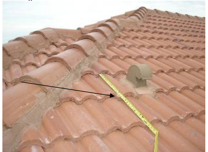
Some of the hip & ridge cap tiles are not correctly secured or bonded. §1518.8.5, §1518.8.11, 1507.4.5.2.1
