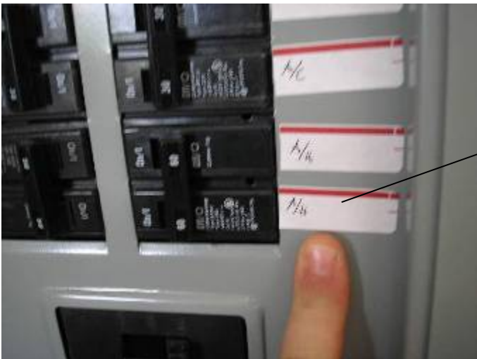
The 60 amp disconnect is too big for the 8kW heating system. A 45 amp breaker should be installed.
