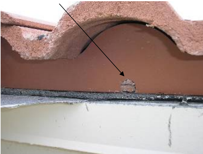
Some of the eaves closure weep holes are obstructed & not cleared through. The roof will not drain correctly. §1518.8.9
