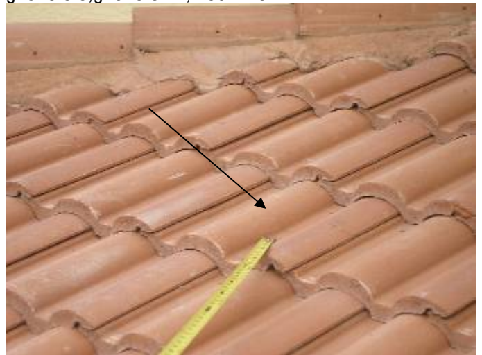
There are loose & incorrectly bonded roof tiles over the back patio. These tiles need to be correctly secured. §1518.8.5, §1518.8.11, 1507.4.5.2.1
