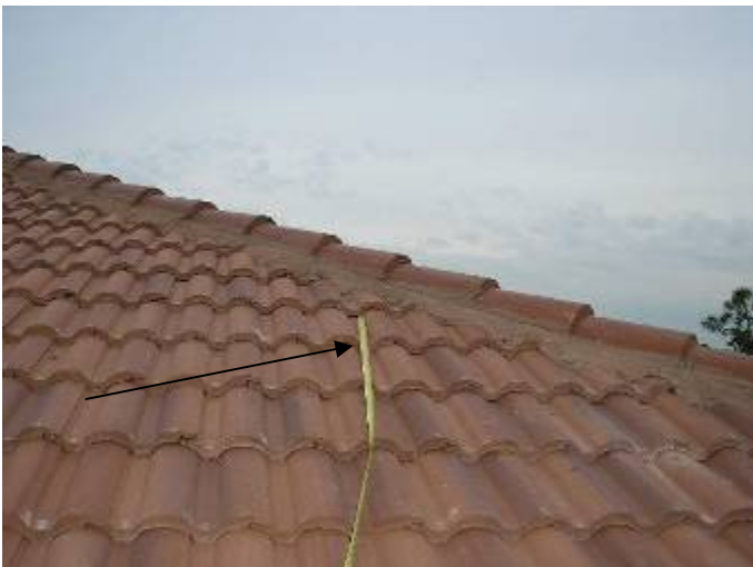
Some of the roof tile headlaps are 2 inches or less. The minimum headlap (tile overlap) is 3 inches. §1518.8.11
