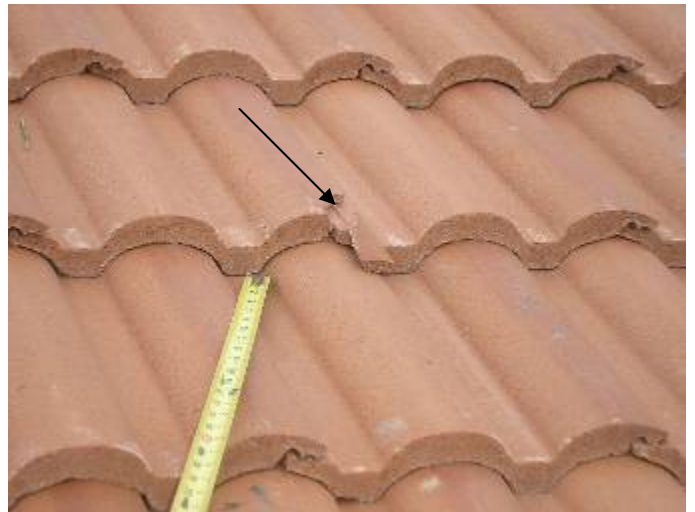
There should not be any broken tiles on the new roof. The tiles need to be removed & replaced; not "glued" back together.
