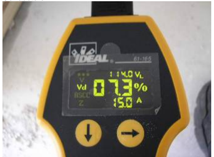
Many of the receptacle outlets had excessive voltage drops at the throughout the house. 2002(NEC) 210.19 Conductors
