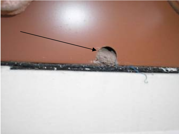
Some of the bird stop weep holes are blocked & obstructed with debris. The openings need to be cleared for correct roof drainage. §1518.8.9
