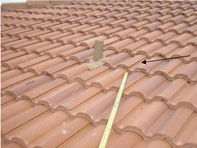
There are loose & incorrectly bonded roof tiles over the 2 nd floor. These tiles need to be correctly secured. §1518.8.5, §1518.8.11, 1507.4.5.2.1
