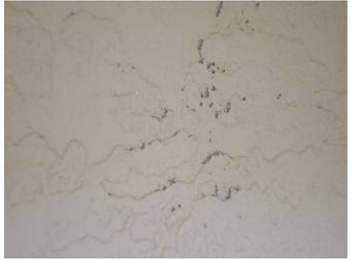
There is exposed stucco & not enough paint on some of the exterior walls. §1403.1.3
