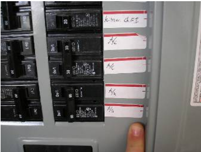
Some of the circuits have not been correctly identified in the main electric distribution panel. The labels need to indicate where the AC units provide service.
