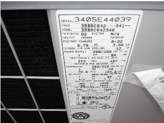
Note: Condensing unit size & information. 3 & 1/2 ton compressor.
