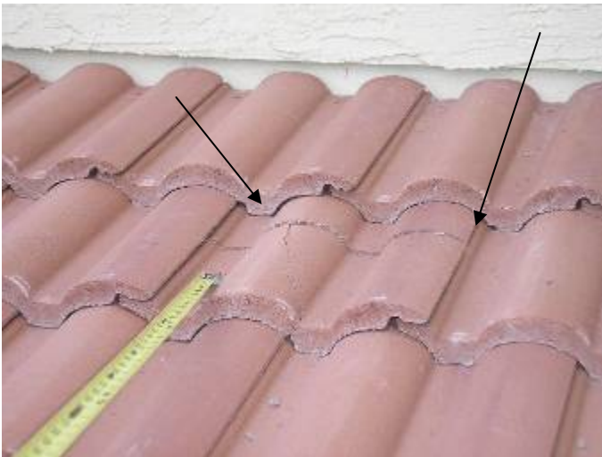
There should not be any broken tiles on the new roof. The tiles need to be removed & replaced; not "glued" back together.
