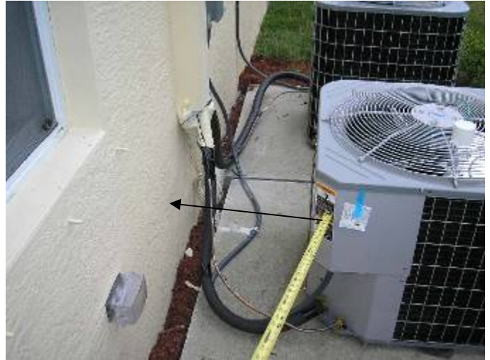
The AC condensing units are turned the wrong way. 36 " working space clearance is required at the electrical access panel covers. 2002 NEC §110.26
