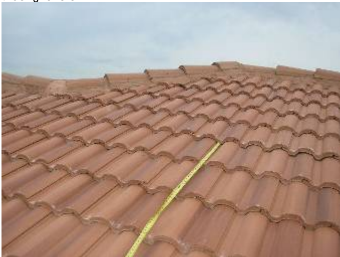
Some of the tile exposures are 14 inches or more. Note: some photos taken with zoom as the builder would not allow access to walk on the roof.
