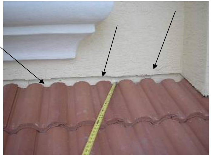
The roof wall abutments have not been correctly pointed up with mortar. R118-3.13
