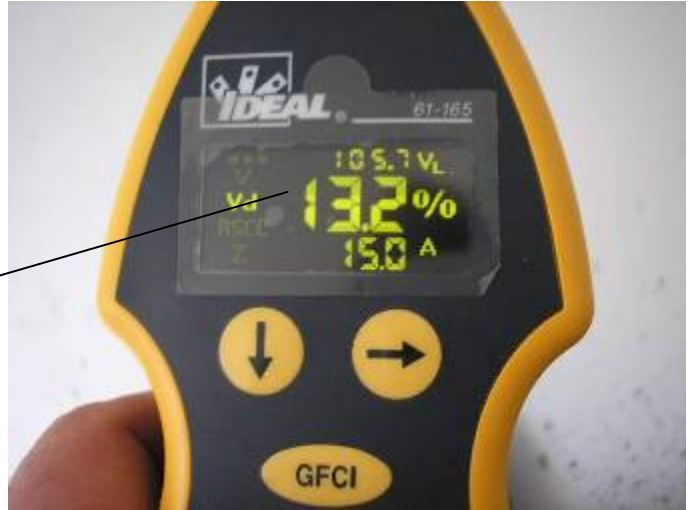
Many of the receptacle outlets had excessive voltage drops at the throughout the house. 2002(NEC) 210.19 Conductors
