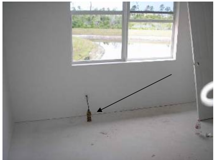
Location of the previous photos. The voltage drops should not exceed 5%. 2002(NEC) 210.19 Conductors
