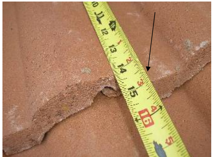
Some of the roof tile headlaps are 2 inches or less. The minimum headlap (tile overlap) is 3 inches. §1518.8.11
