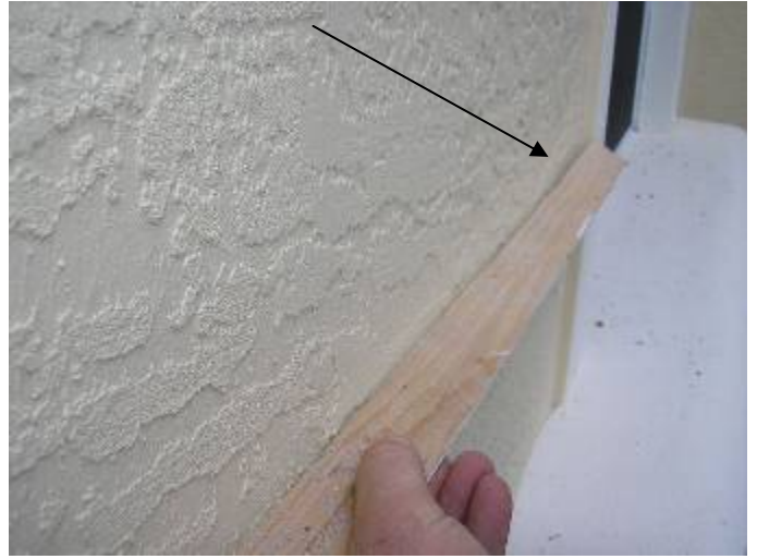
The stucco at some at the walls is concave or curved in & does not appear to be the correct thickness. §2509.1.1
