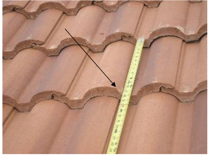
Some of the roof tile headlaps are 2 inches or less. The minimum headlap (tile overlap) is 3 inches. §1518.8.11
