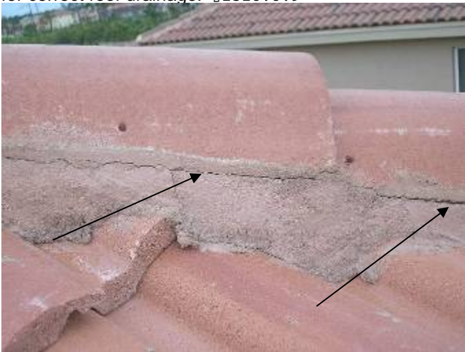
All loose tiles need to be correctly secured.
