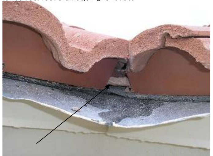
There are broken pieces of tile & debris obstructing the valleys. The roof will not drain correctly.
