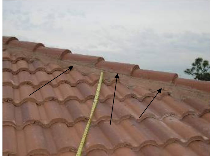
Some of the hip & ridge cap tiles are not correctly secured or bonded. §1518.8.5, §1518.8.11, 1507.4.5.2.1
