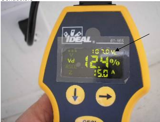
Many of the receptacle outlets had excessive voltage drops at the throughout the house. 2002(NEC) 210.19 Conductors
