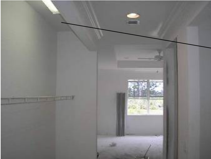
The fixtures remain energized after all of the Arc Fault breakers have been tripped.
