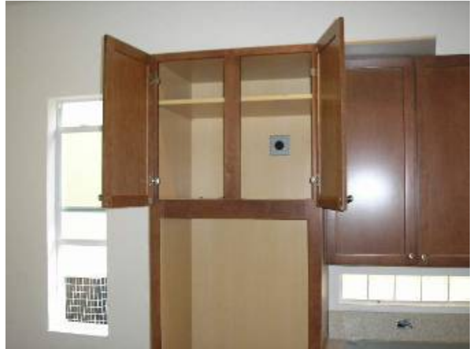
A plug & receptacle are not permitted for the wall oven electric supply. §M304.1
