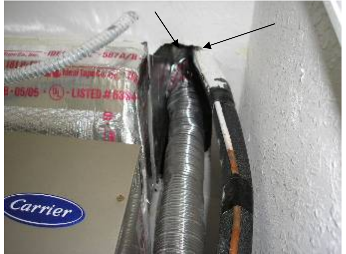
The AC mechanical closets are not completely sealed as required. §13-410.1.ABCD.3.7
