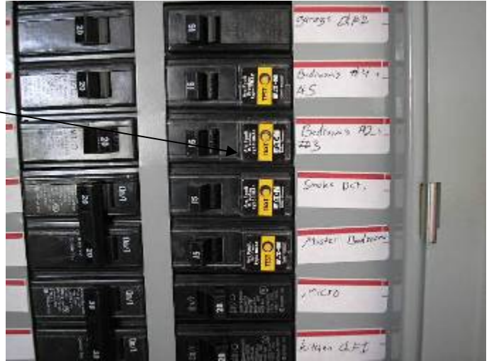
Several of the fixture outlets test non-AFCI protected in the bedrooms.
