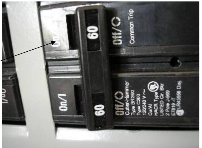
The 60 amp disconnect is too big for the 8kW heating system. A 45 amp breaker should be installed.
