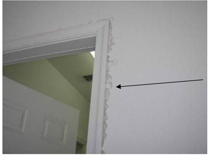
There is damage around the garage/laundry access door. Why was this method used to adjust the wall?
