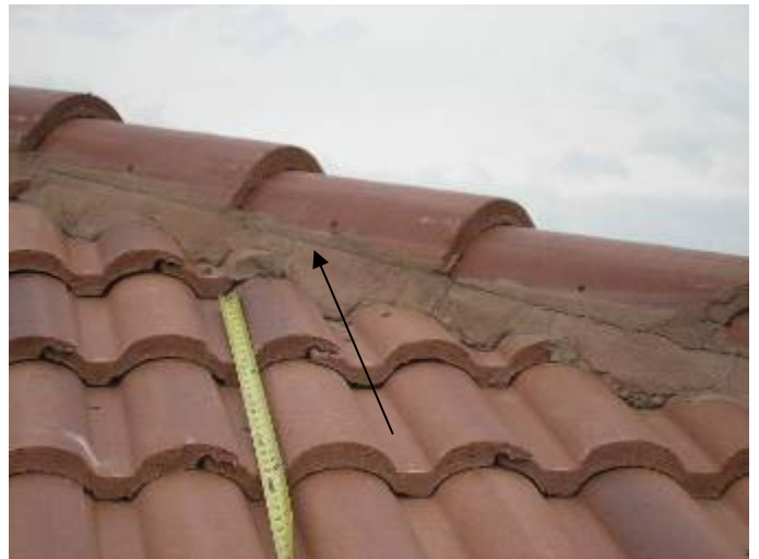
The maximum allowed tile exposure should be not more than 13 & ¼ inches. §1518.8.11
