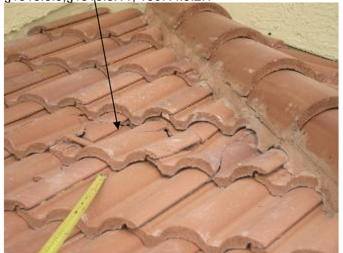
There are loose & incorrectly bonded roof tiles over the back patio. These tiles need to be correctly secured. §1518.8.5, §1518.8.11, 1507.4.5.2.1
