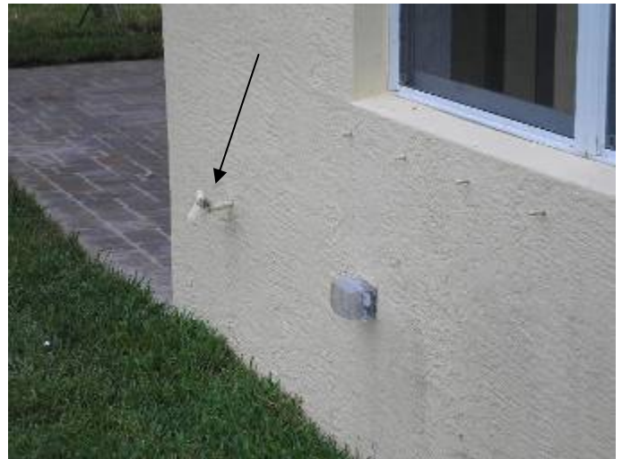
Location of the previous photo. The pipe is not correctly sealed or secured at the wall. §13-606.1.ABC.1.2
