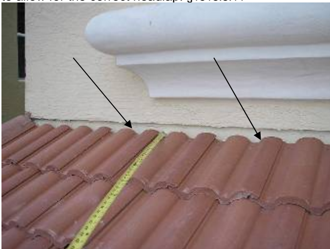
The roof wall abutments have not been correctly pointed up with mortar. R118-3.13
