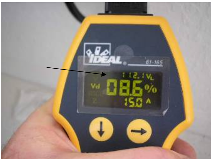
The voltage drops should not exceed 5%. 2002(NEC) 210.19 Conductors
