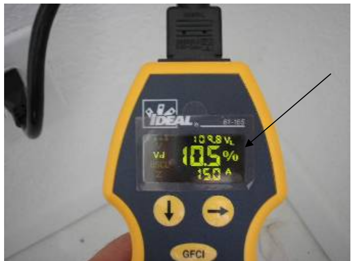
Many of the receptacle outlets had excessive voltage drops at the throughout the house. 2002(NEC) 210.19 Conductors
