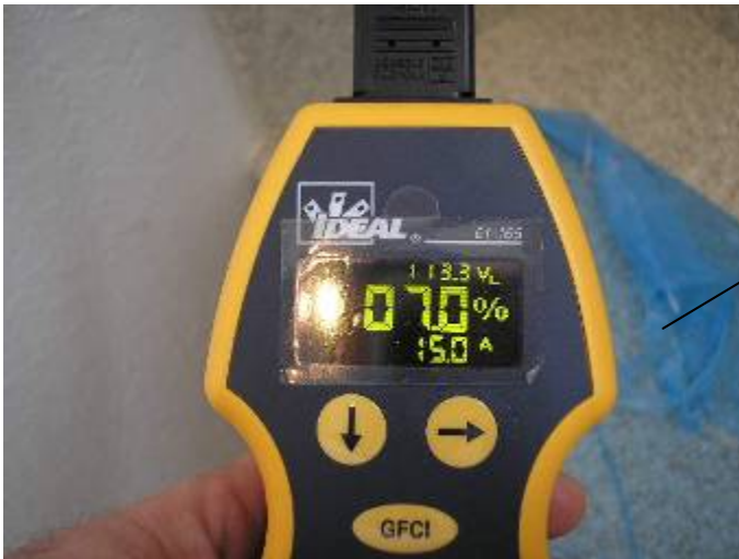
Many of the receptacle outlets had excessive voltage drops at the throughout the house. 2002(NEC) 210.19 Conductors
