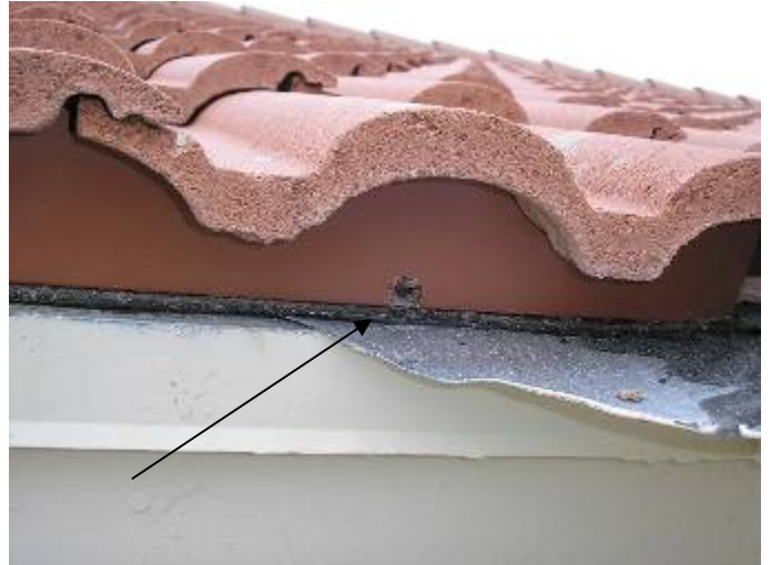
Some of the bird stop weep holes are blocked & obstructed with debris. The openings need to be cleared for correct roof drainage. §1518.8.9
