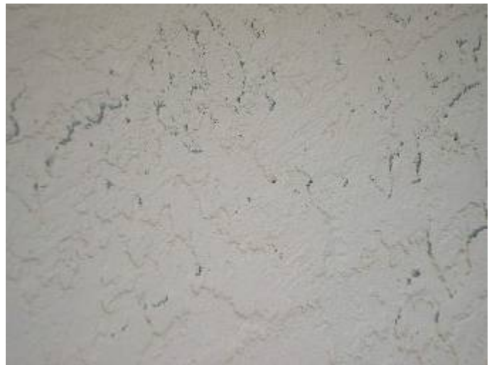
There is exposed stucco & not enough paint on some of the exterior walls.
