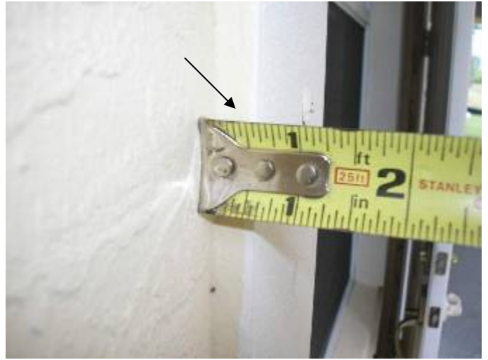
Some of the stucco work appears to be uneven & not the proper depth. ASTM C 926, §2504.2 §1403.1.3
