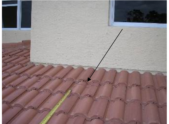
There are loose & incorrectly bonded roof tiles over the back patio. These tiles need to be correctly secured. §1518.8.5, §1518.8.11, 1507.4.5.2.1
