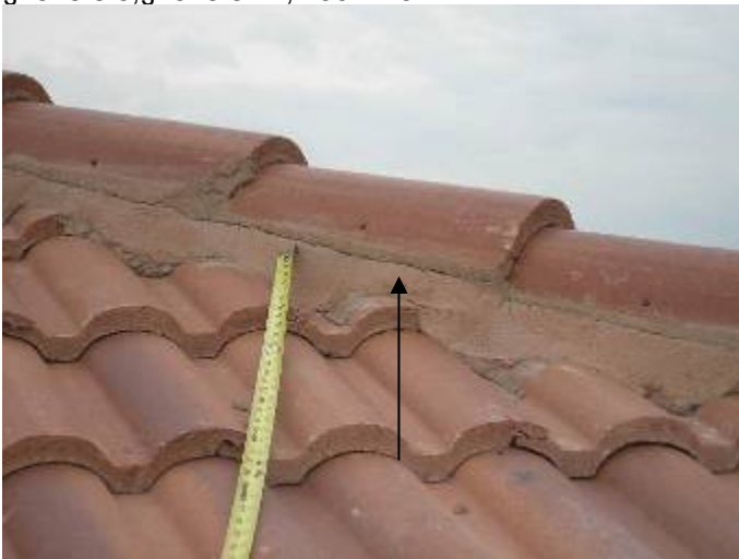
Some of the hip & ridge cap tiles are not correctly secured or bonded. §1518.8.5, §1518.8.11, 1507.4.5.2.1
