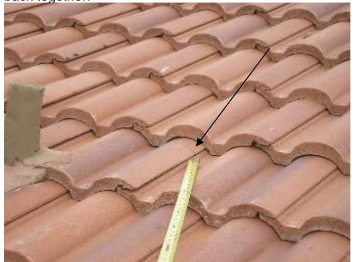
There are broken & loose roof tiles over the 2 nd floor. The tiles need to be removed & replaced; not "glued" back together. §1518.8.5, §1518.8.11, 1507.4.5.2.1
