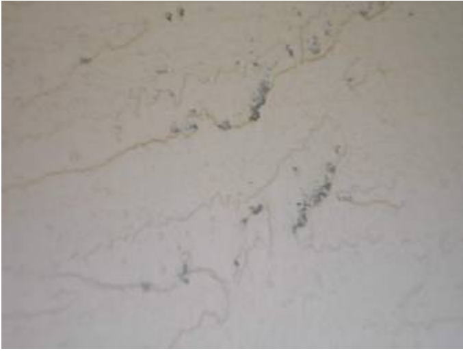
It appears that only one coat of paint is on the wall.
