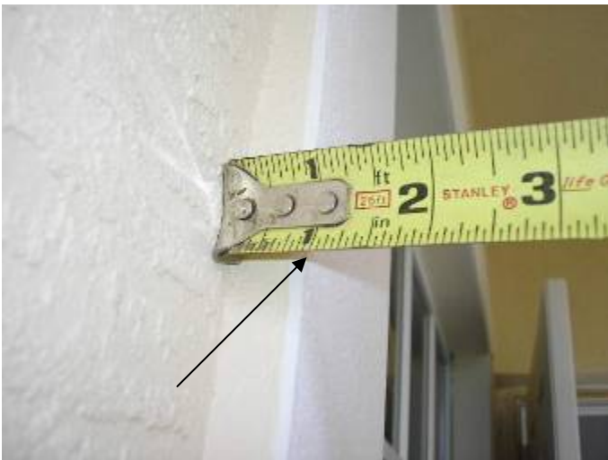
The stucco at some at the walls is concave or curved in & does not appear to be the correct thickness. §2509.1.1
