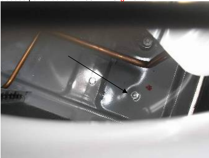
The A/C condensers are not secured properly. There are not enough straps or fasteners at the base of the units. M301.13.1
