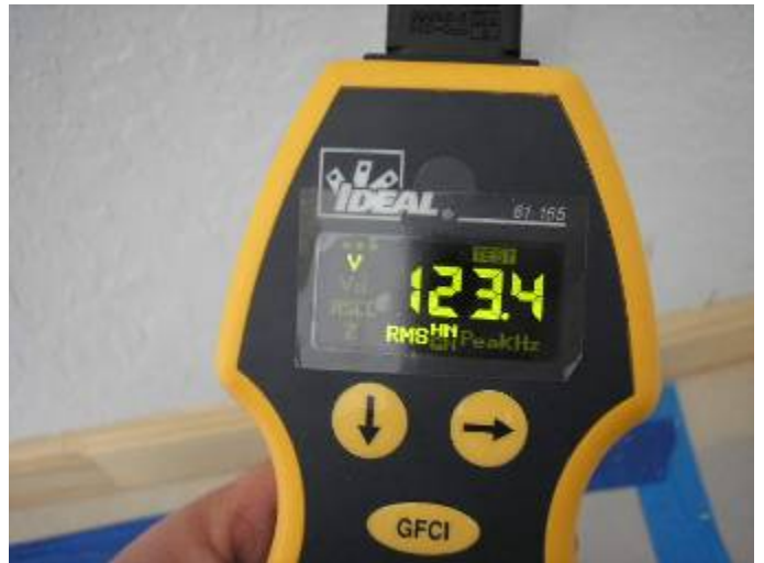
Many of the receptacle outlets had excessive voltage drops at the throughout the house. 2002(NEC) 210.19 Conductors
