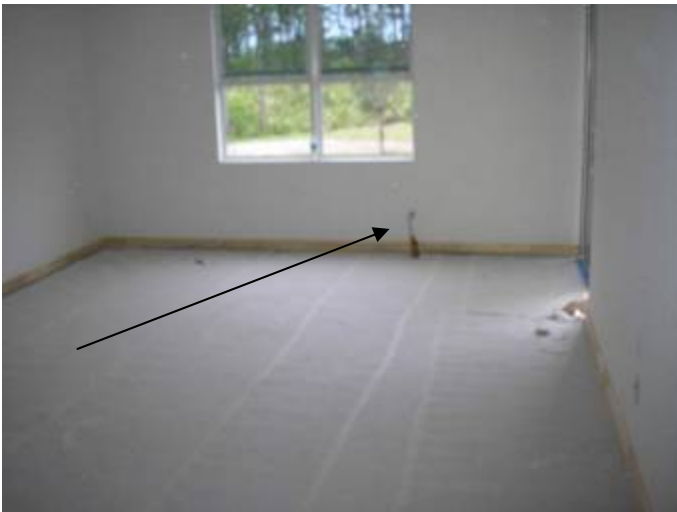
Location of the previous photos. The voltage drops should not exceed 5%. 2002(NEC) 210.19 Conductors
