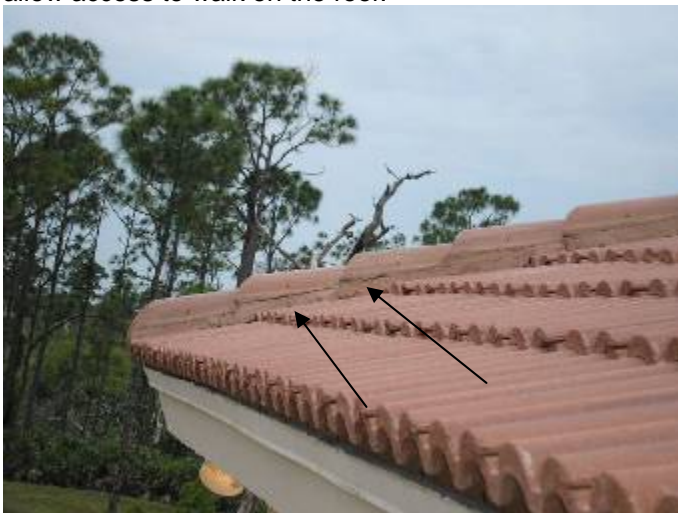
Some of the hip & ridge cap tiles are not correctly secured or bonded. §1518.8.5, §1518.8.11, 1507.4.5.2.1
