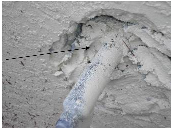
The main water supply piping was not correctly secured or sealed at the wall. Sheathing is required to protect the copper piping & was not visible. §P305.1
