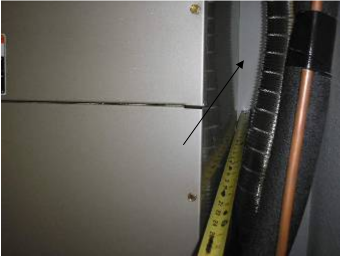
There is not enough clearance around this AC air handler. §13-410.1.ABCD.3.0.3
