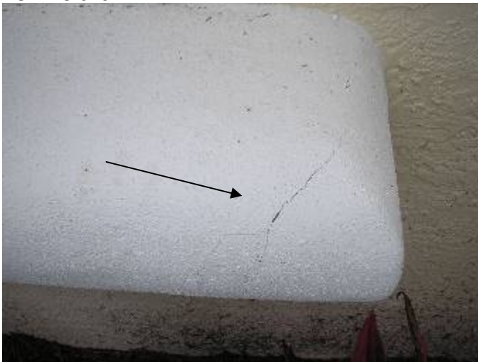
Damaged areas & unsealed openings in the stucco trim & Styrofoam banding need to be corrected. §13-606.1.ABC.1.2
