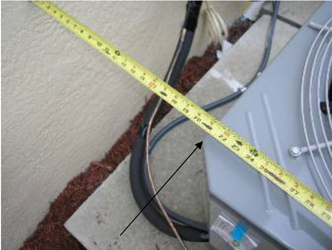
The AC condensing units are turned the wrong way. 36 " working space clearance is required at the electrical access panel covers. 2002 NEC §110.26
