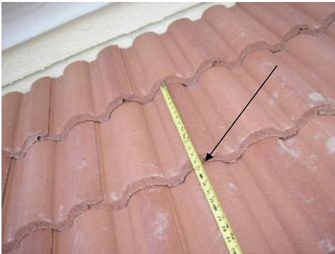
The roof tiles are 16" to 16 & 1/2" in length. There should be no more than 13 – 13 & 1/2 inches of exposed roof tile to allow for the correct headlap. §1518.8.11
