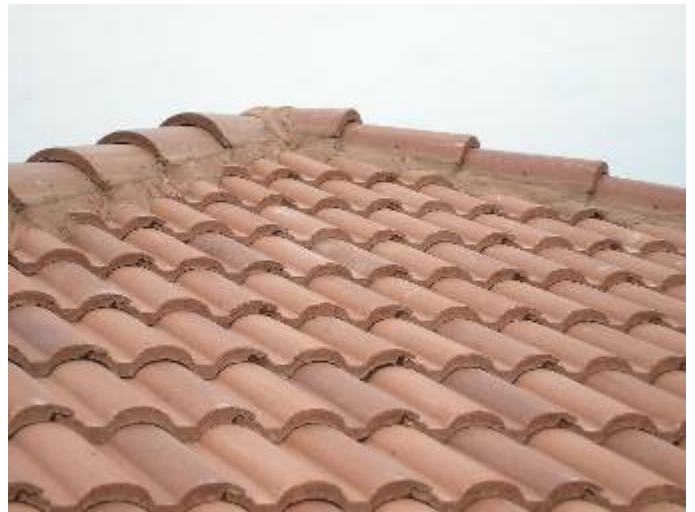
Location of the previous photos at the left & right sides of the upper roof.
